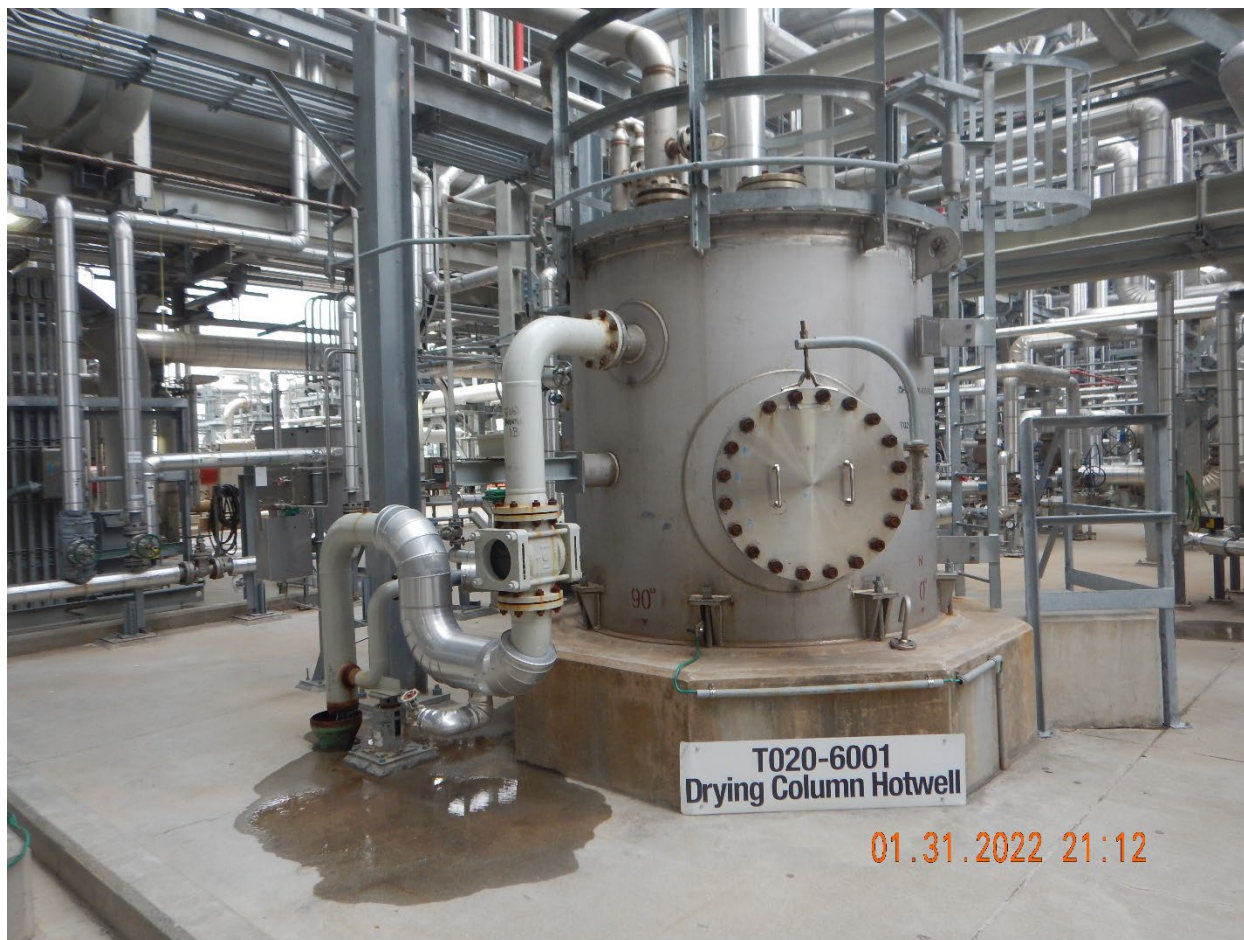
Drying Column Hotwell. Actual photo time was 02/01/2022 at 09:12AM.
