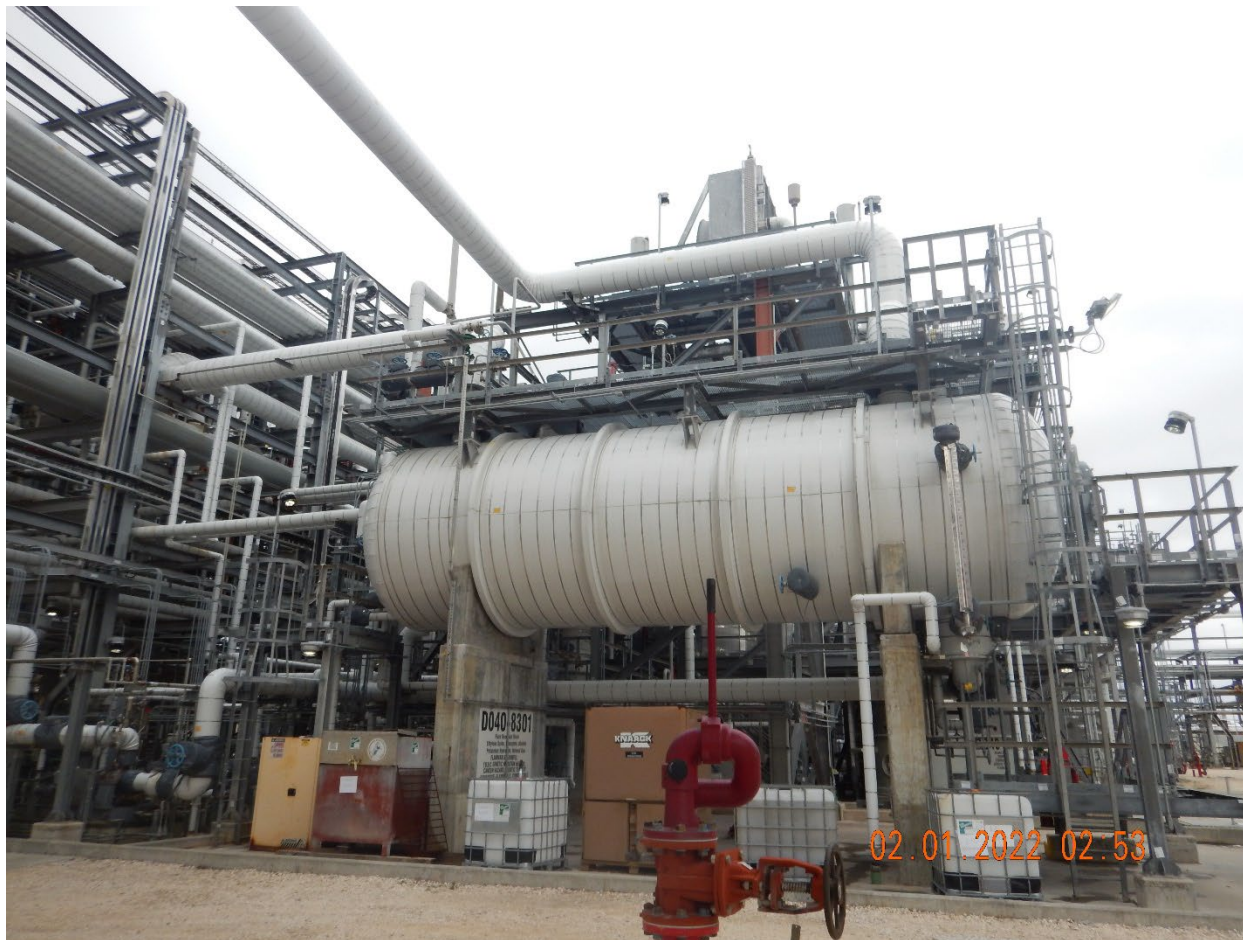
ETO 4/5 Knockout Tank prior to Flare Knockout. Actual photo time was 02/01/2022 at 02:53PM.
