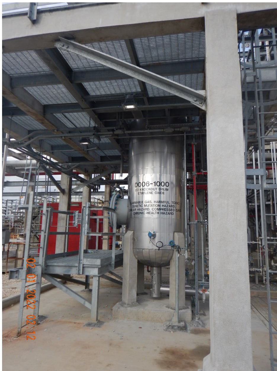
EO Knockout Drum for purging rail cars. Actual photo time was 02/01/2022 at 02:12PM.
