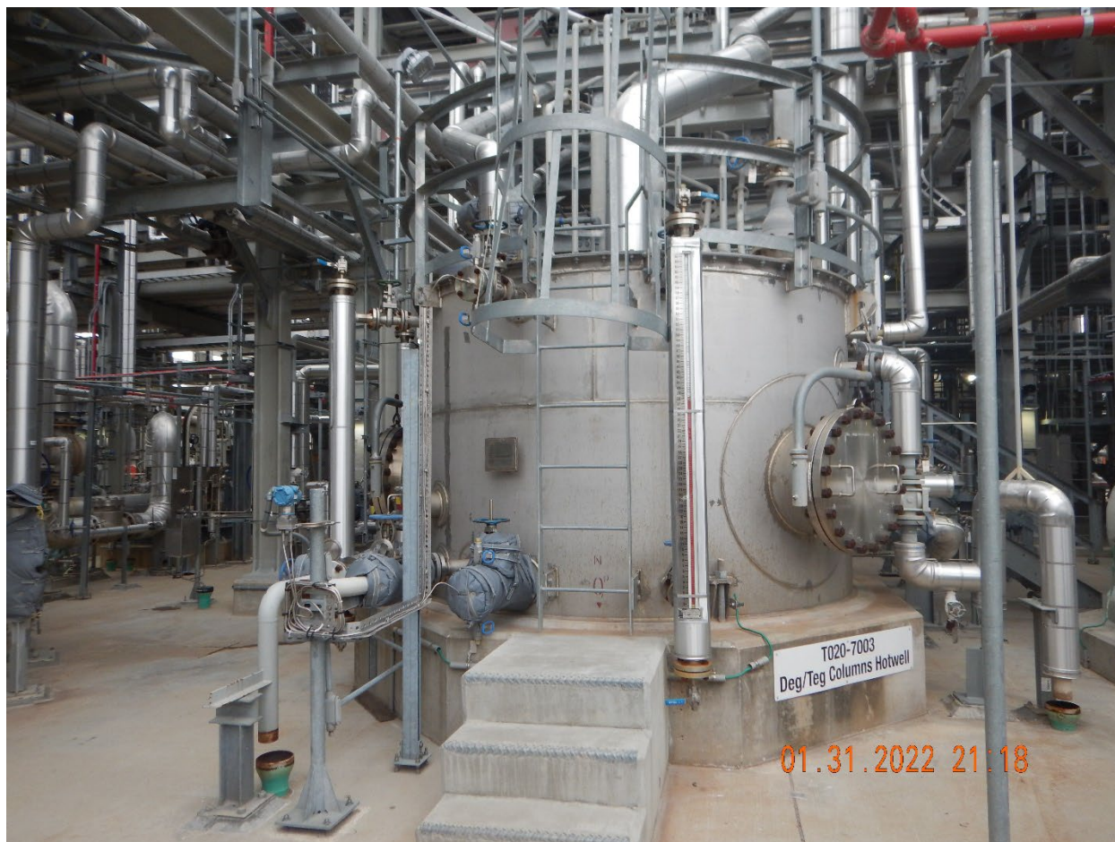
Deg/Teg Columns Hotwell. Actual photo time was 02/01/2022 at 09:18AM.
