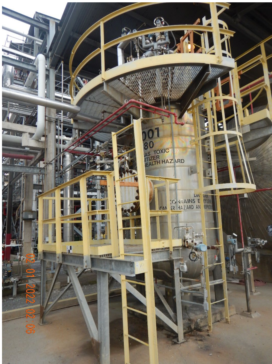
EO Break Tank. Actual photo time was 02/01/2022 at 02:06PM.
