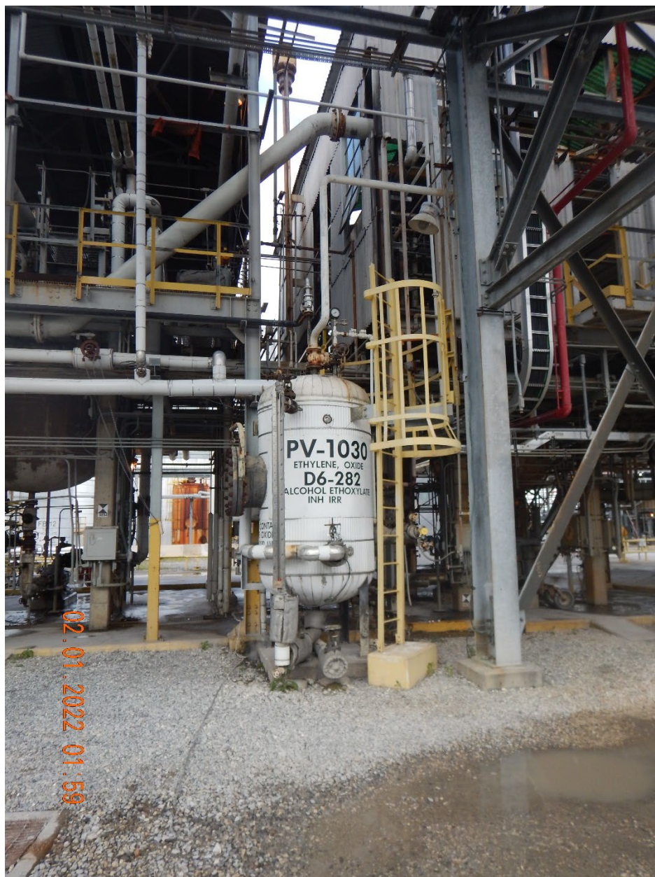
PV-1030 Knockout Pot, serves ETO 1 unit. Actual photo time was 02/01/2022 at 01:59PM.
