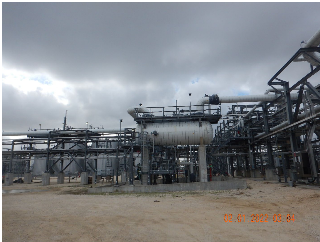
Combined Flare Knockout Tank. Actual photo time was 02/01/2022 at 03:04PM.
