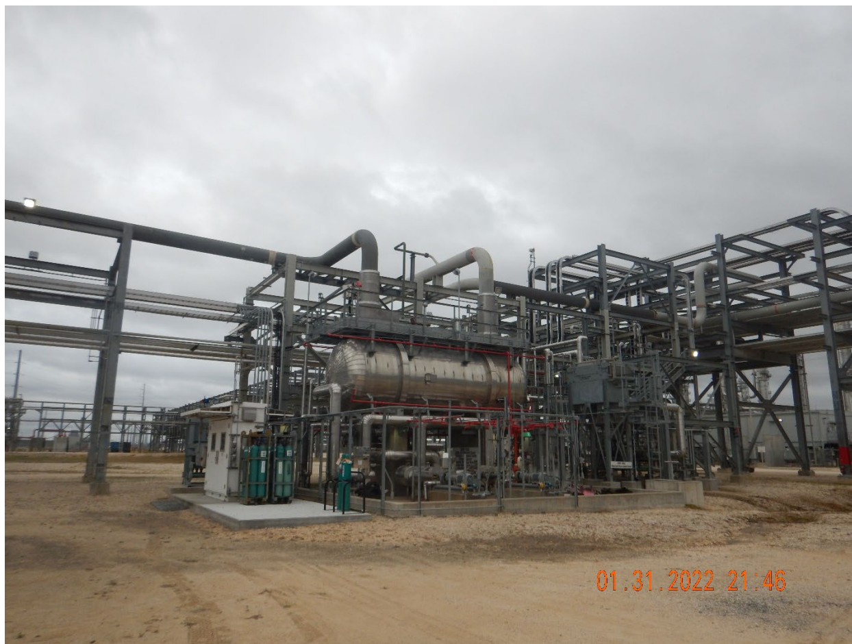
EO Flare Knockout Drum. Actual photo time was 02/01/2022 at 09:46AM.
