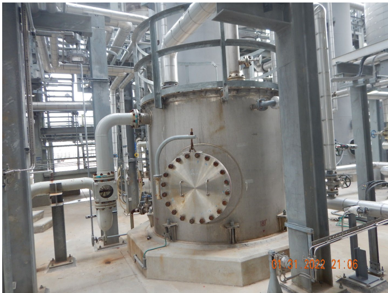
Evaporator Hot Well. Actual photo time was 02/01/2022 at 09:06AM.
