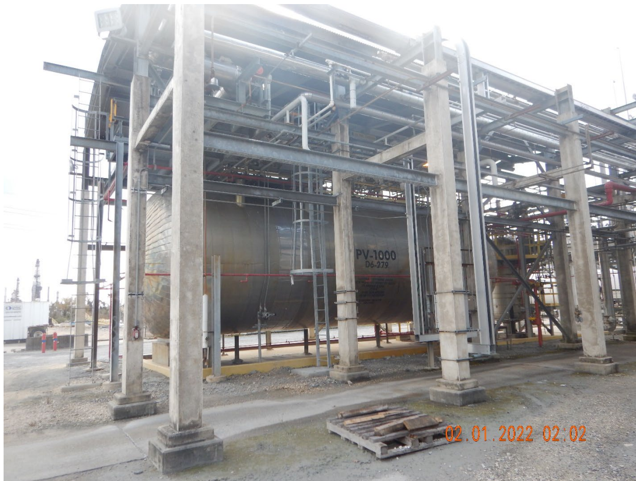
PV-1000 EO Tank, served by the EO Loop. Actual photo time was 02/01/2022 at 02:02PM.
