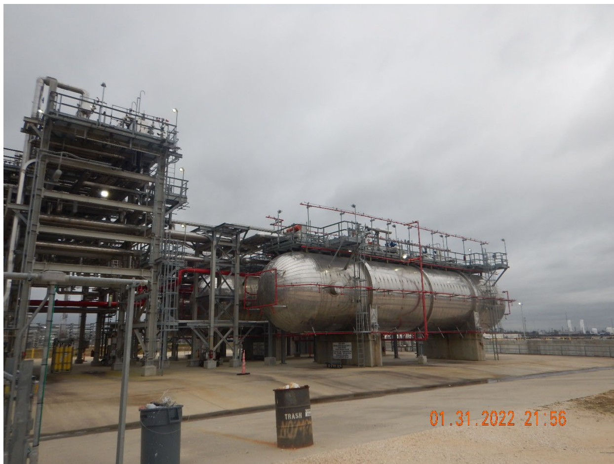
EO Bullet Storage Tanks. Actual photo time was 02/01/2022 at 09:56AM.
