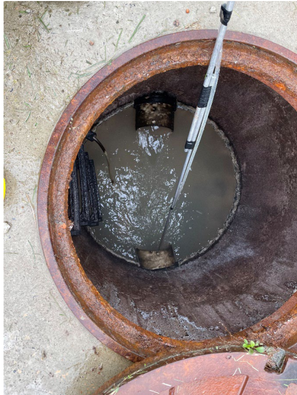
Photo #4. The facility's sampling probe was resting at the bottom of the monitoring manhole.
