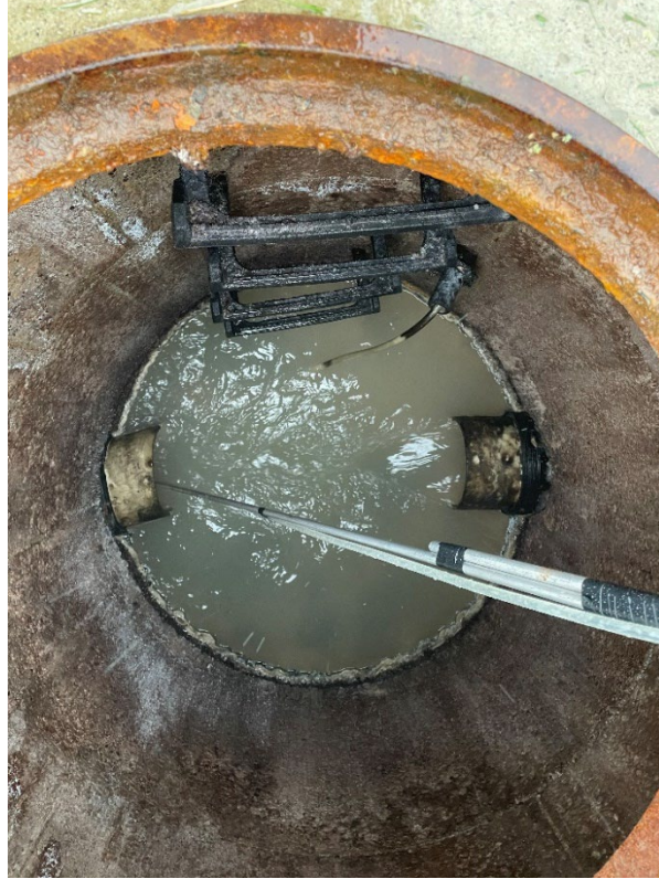
Photo #1. Samples were collected from the discharged pipe in the monitoring manhole.
