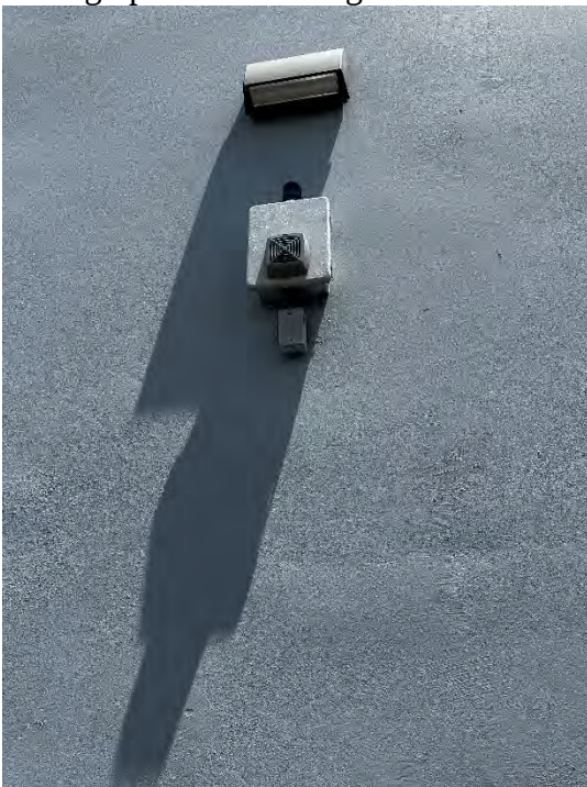
Photograph 10: Fire alarm outside the CAA.
