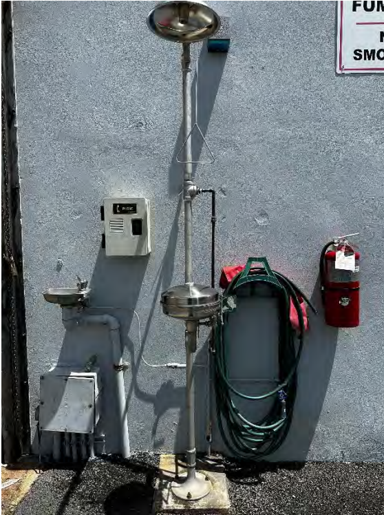
Photograph 11: Emergency equipment outside the CAA.
