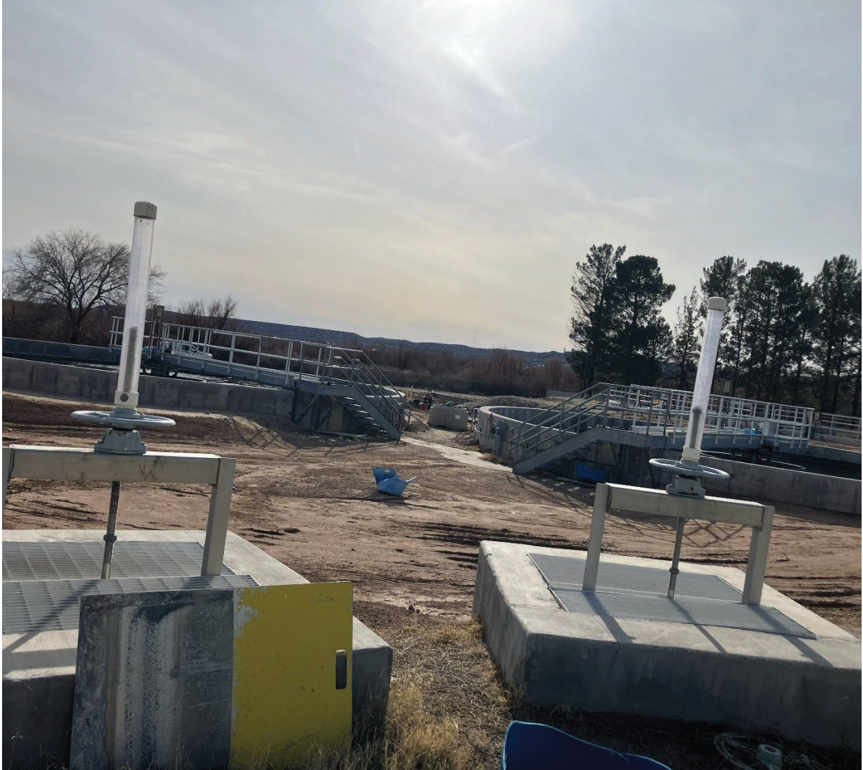
Flow regulators for the two clarifiers.
