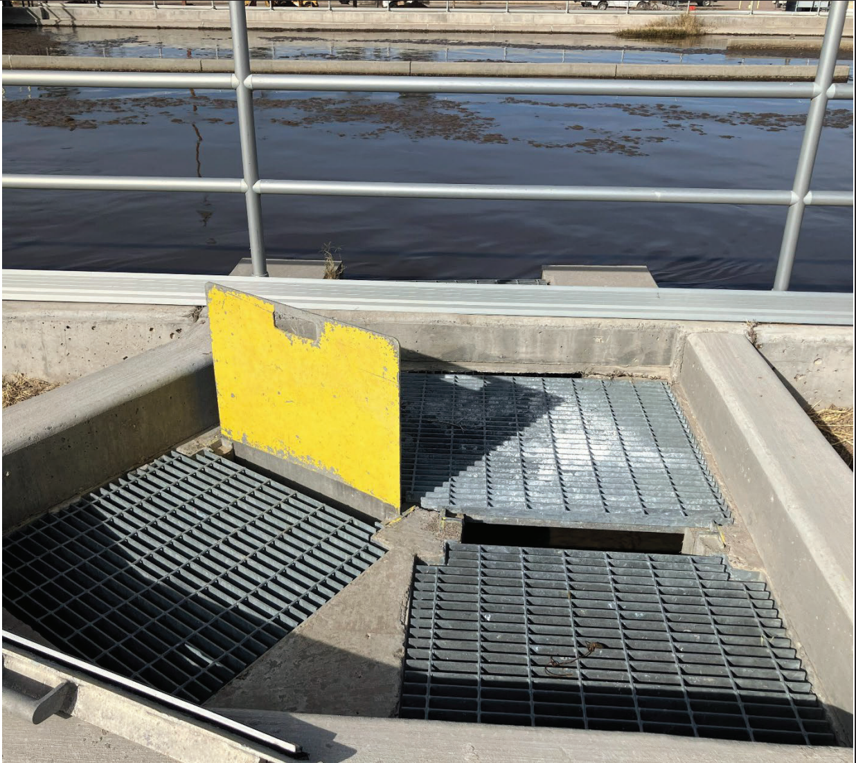
Flow splitter from aeration basin to clarifiers
