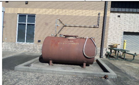
Photo-8 Used Oil Tank (Faded Label)
