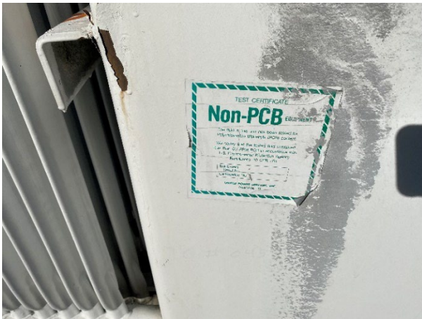
Photo 60: Non-PCB Transformer leaking oil.
