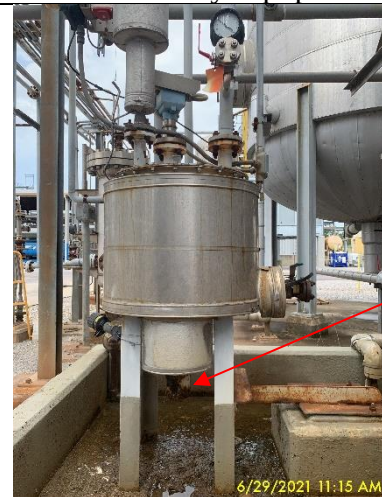
Picture-5 Potential Rust on the Ancillary Equipment associated with the Waste J2 Methanol Tank
