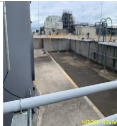
Picture-11 Secondary Containment DAI Spent MEK Tank Area
