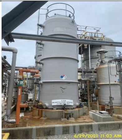
Picture-1 Waste J2 Methanol tank
