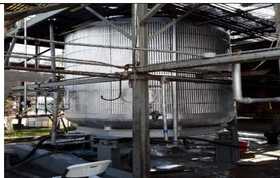
Photo-14 Production Area #3, Reactor and associated piping painted
