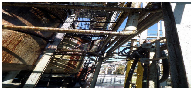
Photo-9 Production Area #3, Stained piping of the Reactor
