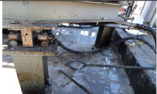
Photo-6 Production Area #3, Open drip pan and solid debris inside the containment area
