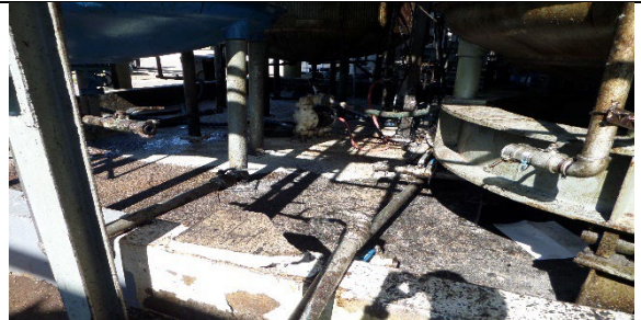
Photo-7 Production Area #3, Chipped secondary containment wall
