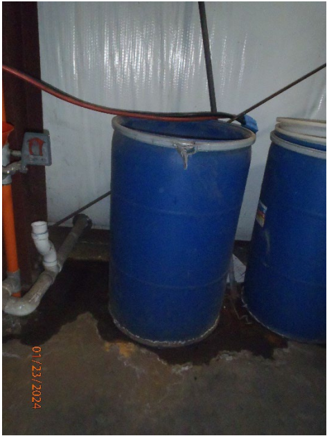
Picture 1 – Battery Charging Station overspill drum
