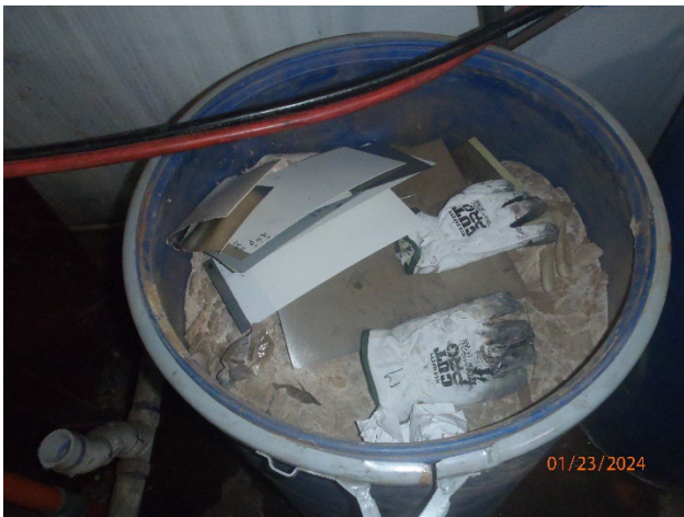
Picture 2 – Battery Charging Station overspill drum
