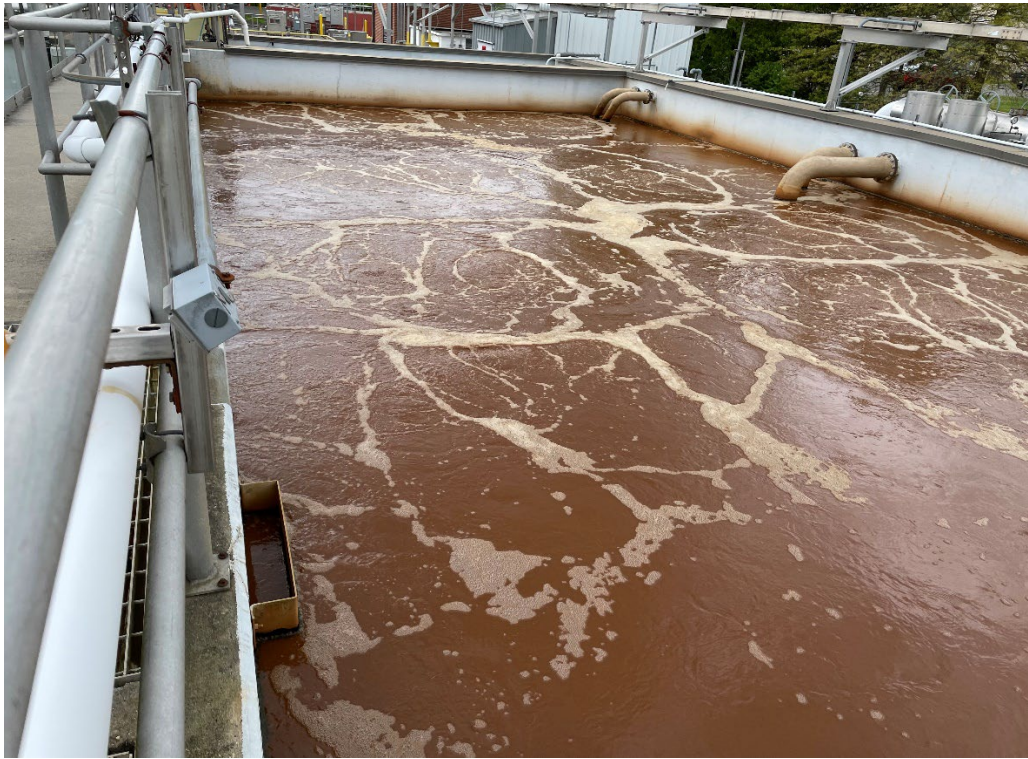
Photo #1. Uneven air distribution in the aeration tank was observed.
