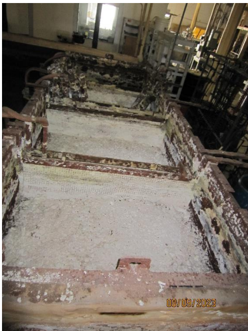
Photo #3 – Out of service large barrel plating line tanks.
