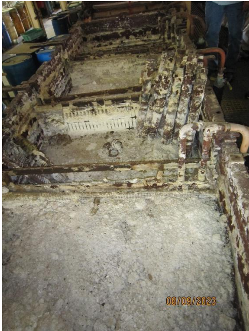
Photo #1 – Out of service large barrel plating line tanks.
