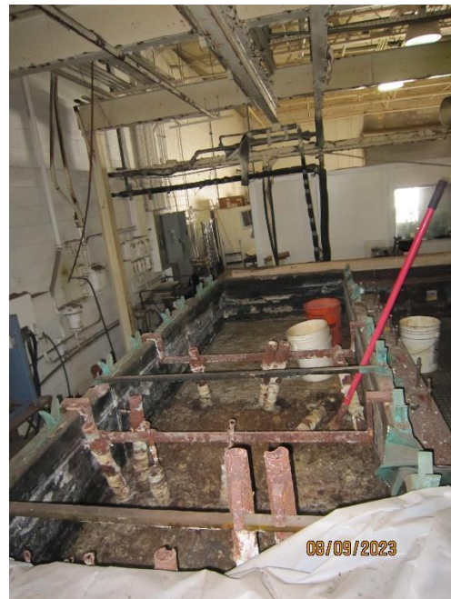
Photo #4 – Out of service large barrel plating line tanks.
