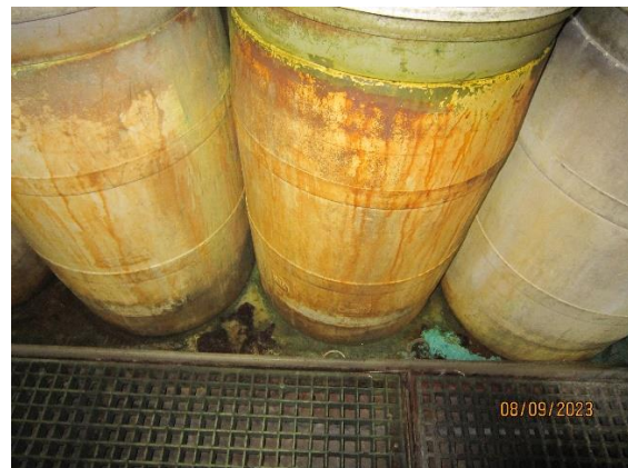
Photo #8 – Residual waste on the floor of the the cadmium plating line.
