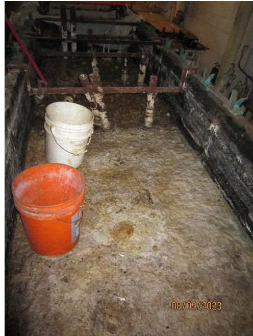
Photo #2 – Out of service large barrel plating line tanks.
