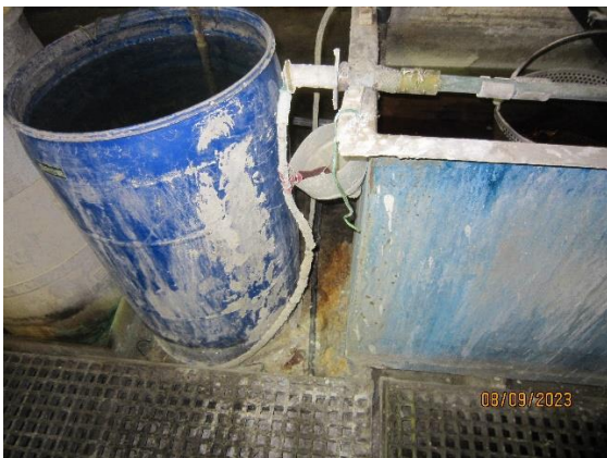
Photo #7 – Residual waste on the floor of the the cadmium plating line.
