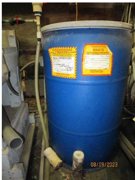
Photo #35 – 55-gallon containers of toxic hazardous waste filters.
