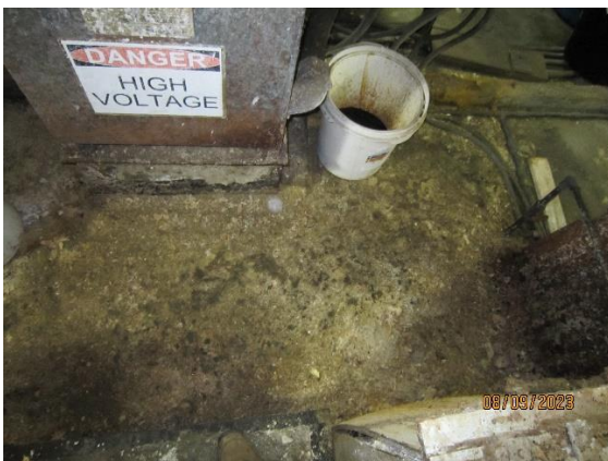
Photo #9 – Residual waste on the floor of the the cadmium plating line.
