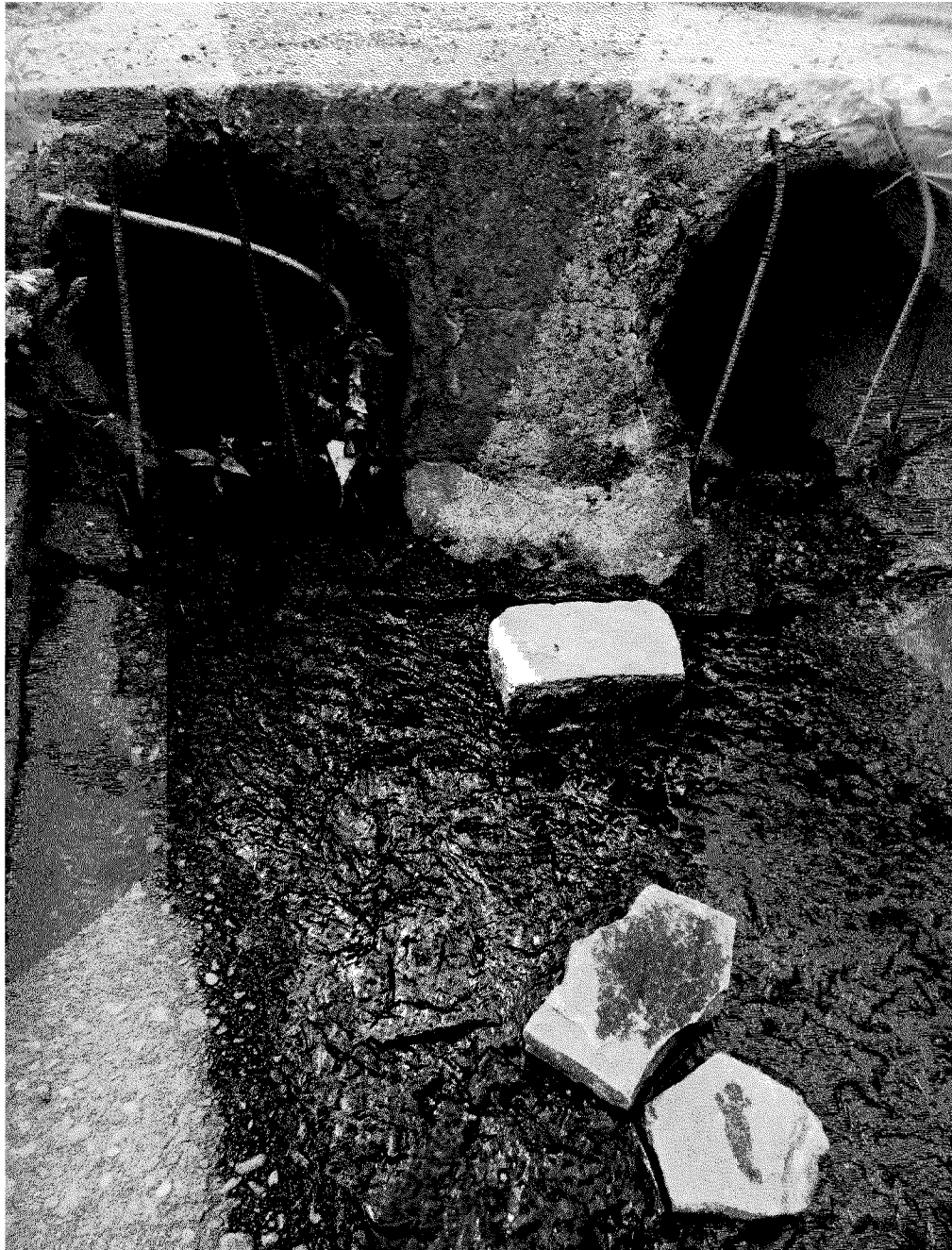
Photo 5: LQ-05 (photo taken 05/28/2024 at approx. 13:00) Outfall located near 5 Suntaug Road, discharging into Lake Quinsigamond. Sample points are indicated by a red X.
