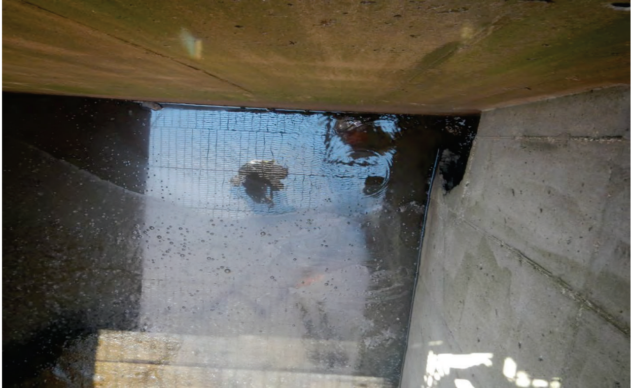
Photo 20, oil sheen in the discharge of Outfall 001.
