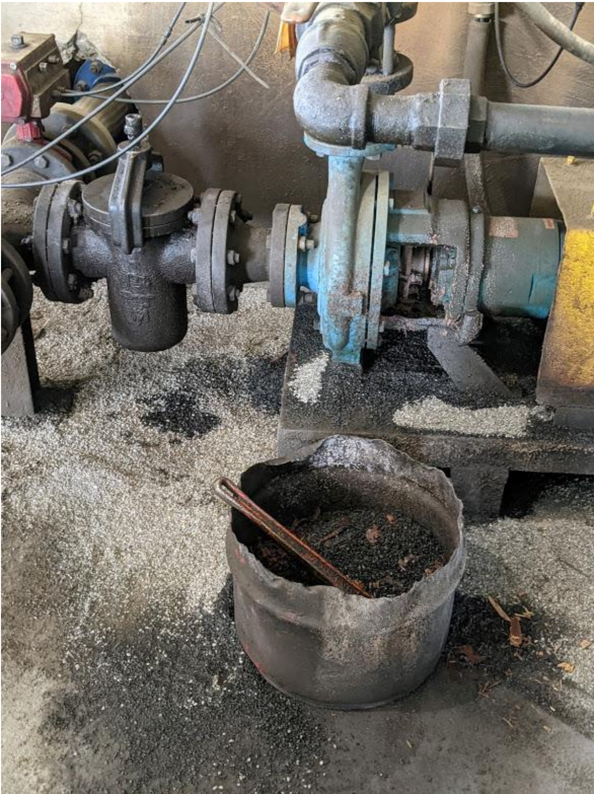
Photograph 2 of 3: SAA container used to collect incidental spills from filtration of hazardous material
