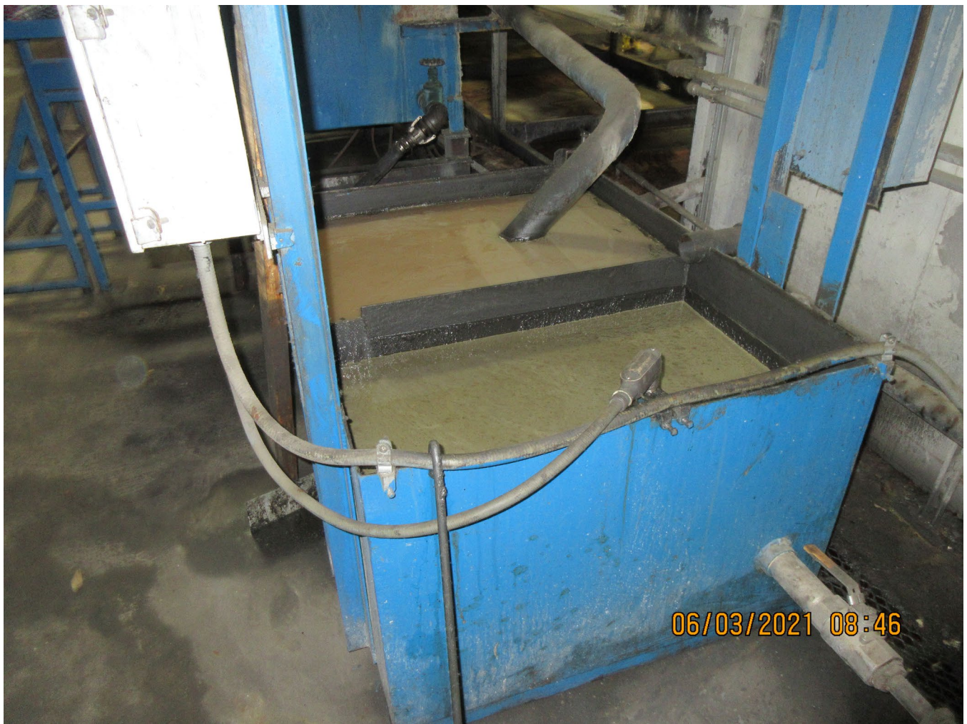
Photo 3 – Oil Separation tanks in Chemical Treatment Area
