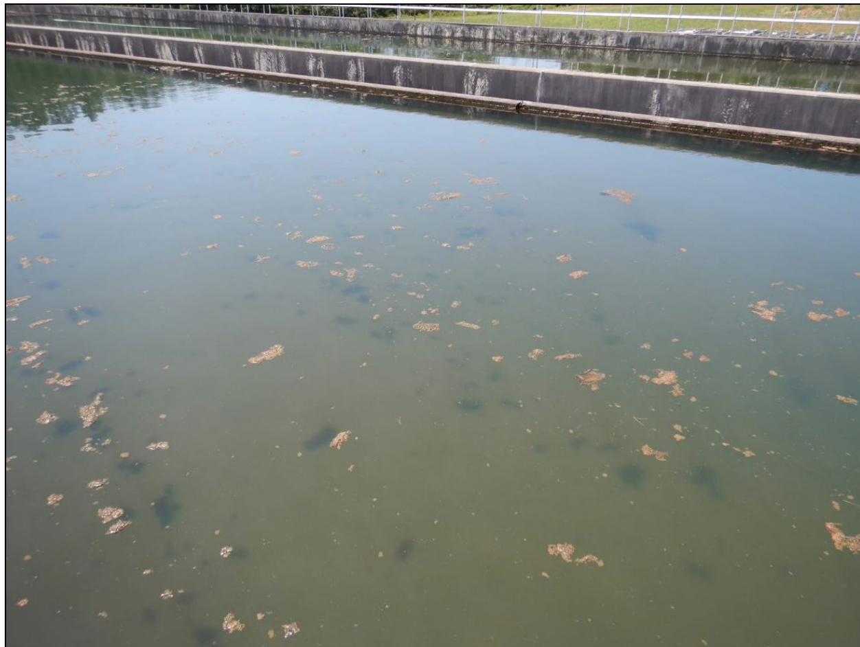
Photograph 22. Sedimentation Basin No. 6 View of floating, bulking solids at the surface of Sedimentation Basin No. 6. System representatives stated that this was a common challenge in the summer.
