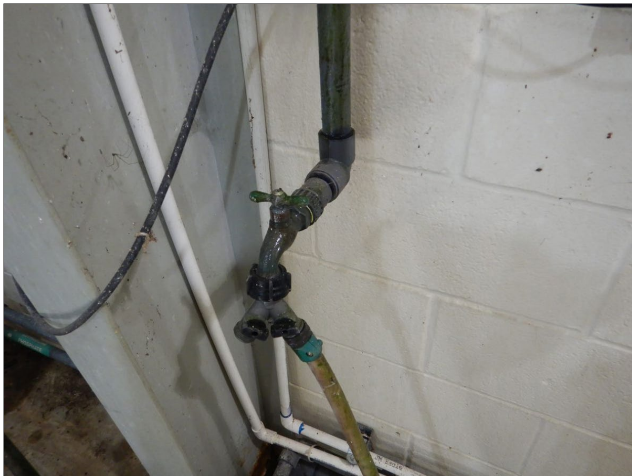
Photograph 12. Potable Water Line, Chemical Storage Room, Ouachita WTP View of a potable water line with a threaded hose tap in the caustic soda, poly-orthophosphate, and coagulant chemical storage room. This line did not contain backflow prevention, but System representatives stated that an RPZ outside the building created backflow prevention for this entire building.
