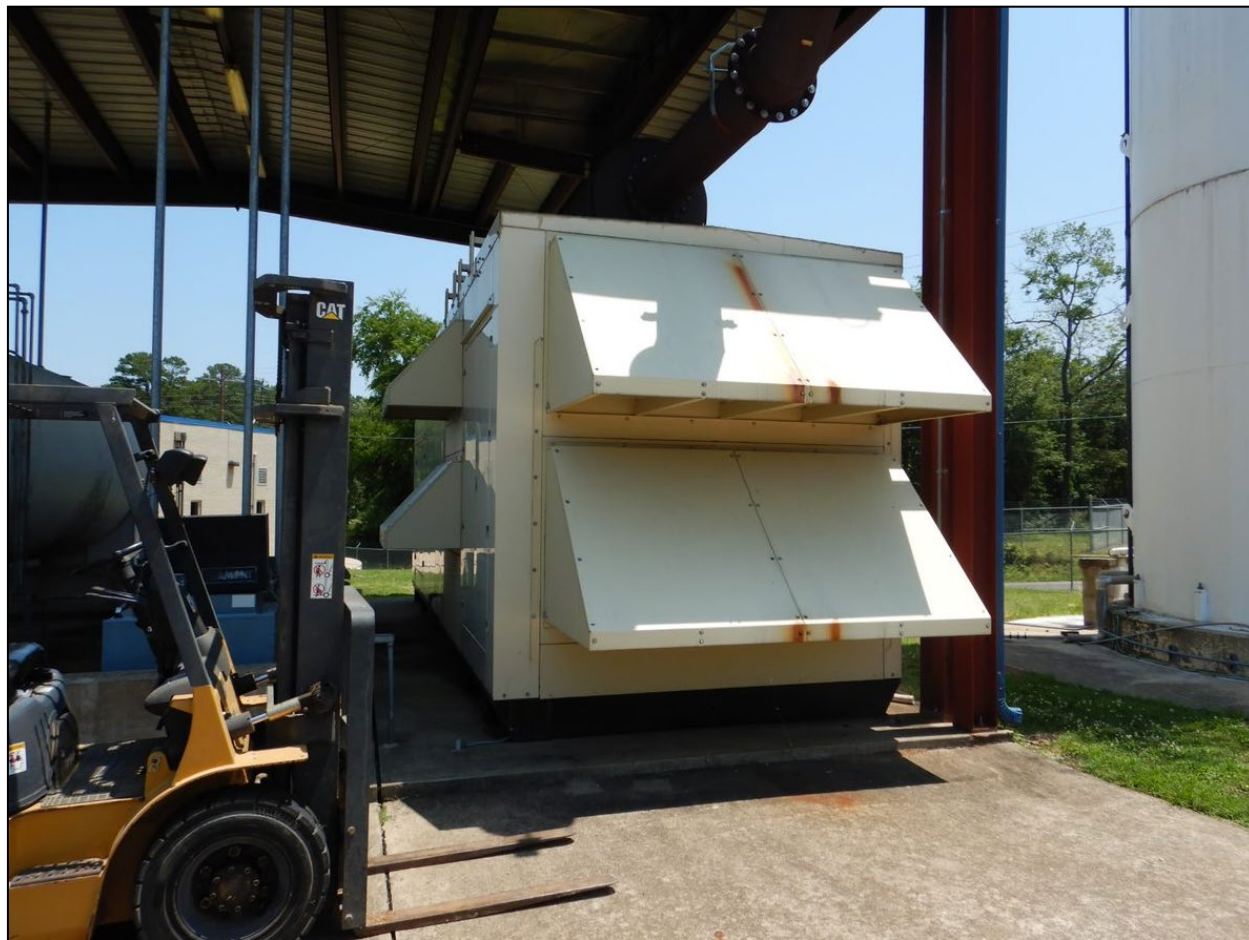
Photograph 36. Mounted Generator, Ouachita WTP View of the mounted 2.0 MW backup generator at the Ouachita WTP. The Water Production Manager stated that the generator could handle the full load of the WTP in the event of a power outage, and that the generator would turn on automatically.
