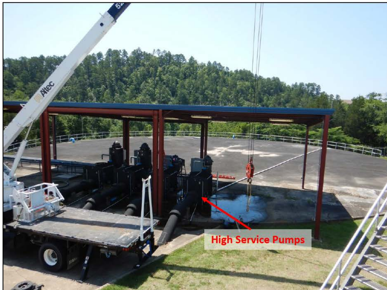
Photograph 27. Clear Well #3, Ouachita WTP View of the 2,000,000gallon Clear Well #3 that was present onsite at the Ouachita WTP. Also visible in this image are the four, high service pumps that send treated water into the distribution system.
