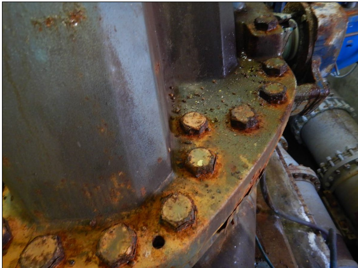
Photograph 39. Pump No. 4, Music Mountain Pump Station View of the metal loss/corrosion that was taking place on the bolts and flange of Pump No. 4. The metal also appeared to be wet.
