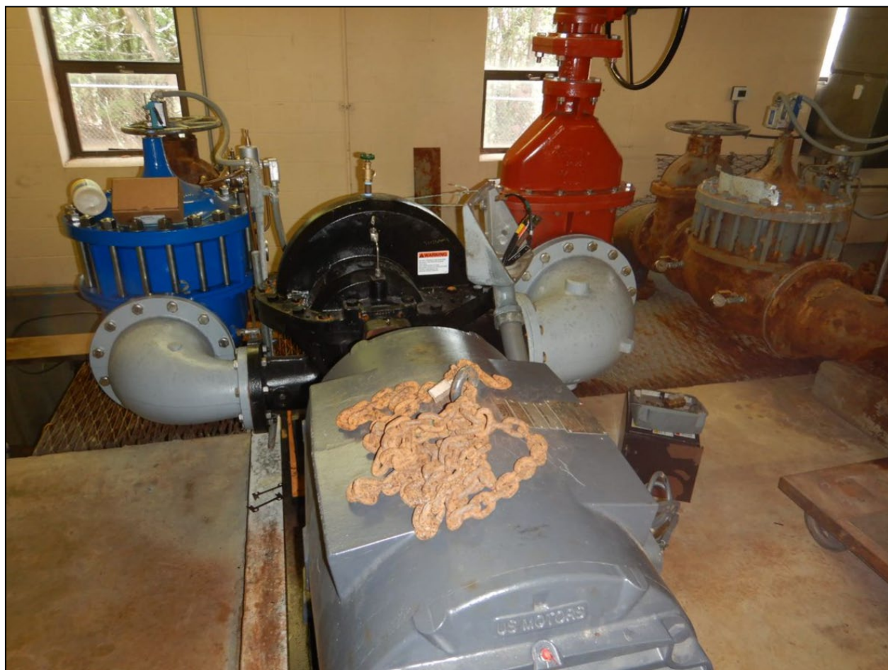
Photograph 38. Music Mountain Pump Station View of a newly replaced pump inside of the Music Mountain Pump Station.
