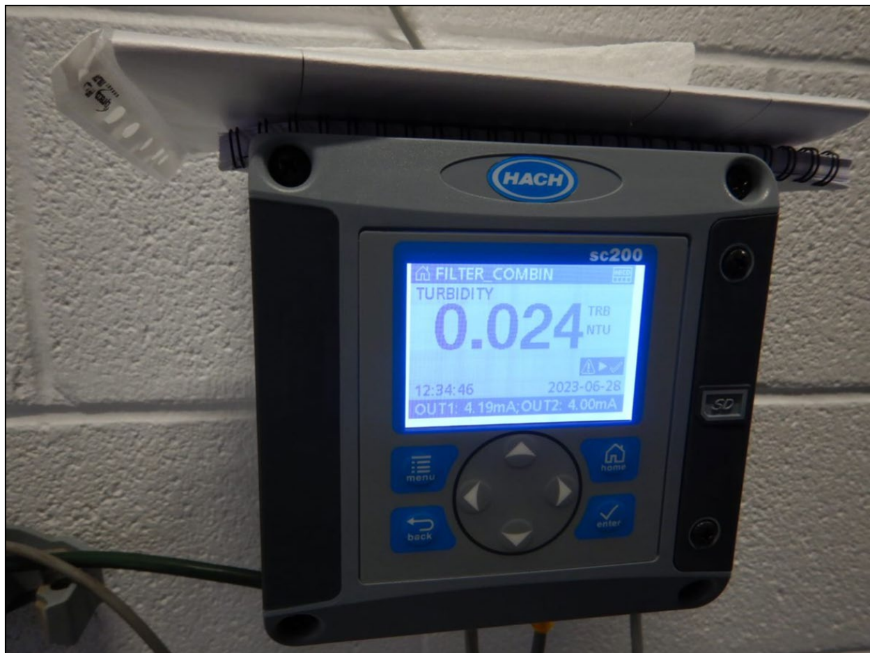
Photograph 26. Combined Filter Effluent Turbidimeter View of the combined filter effluent turbidimeter that was present inside of the sodium hydroxide storage room. The turbidimeter was reading 0.024 NTU at 12:34 p.m., and System representatives stated that this reading came from a common effluent line extending from the filters.
