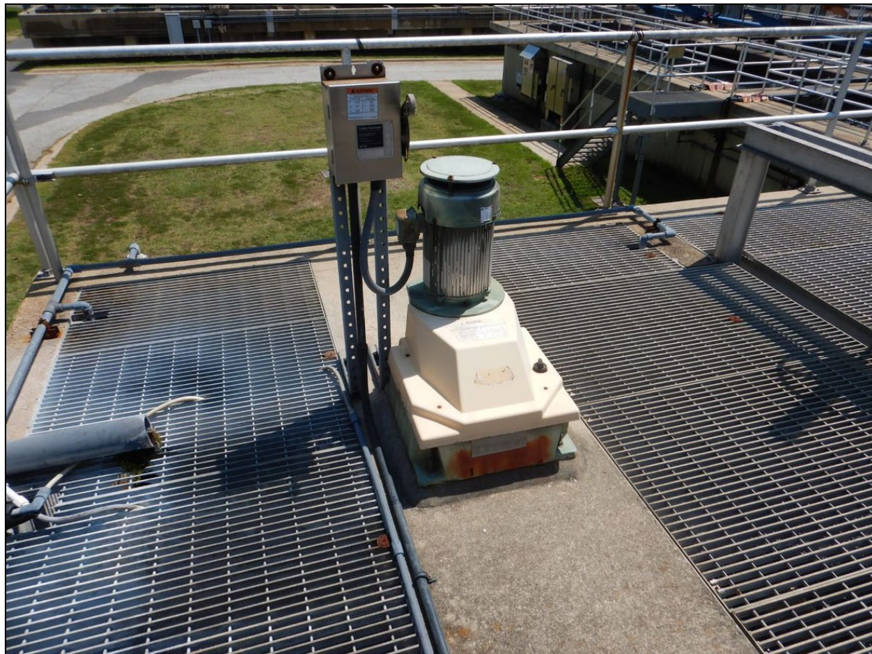
Photograph 16. Rapid Mixer, Ouachita WTP View of one of the two rapid mixers at the Ouachita WTP. Only one mixer was in use during the inspection, and System representatives stated that only one was needed for adequate mixing.
