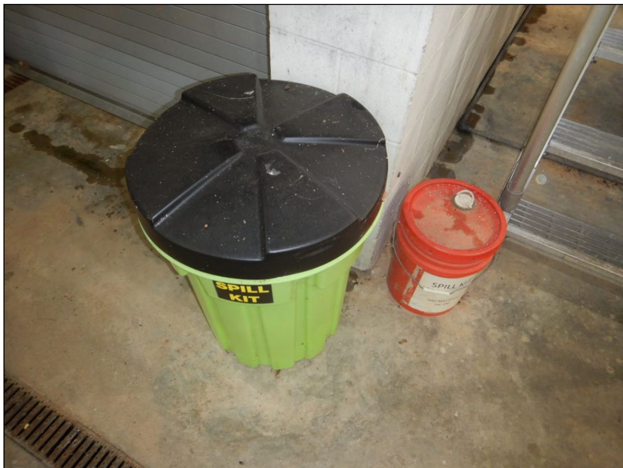
Photograph 14. Chemical Storage Room, Ouachita WTP View of a chemical spill kit that was present in the caustic soda, poly-orthophosphate, and coagulant chemical storage room.
