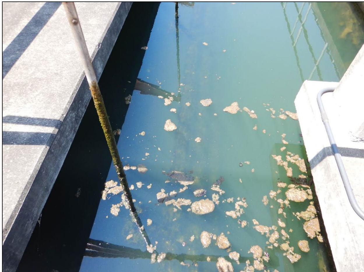
Photograph 21. Floating Solids, Flocculation Chamber View of floating, bulking solids that were floating on surface of the flocculation chamber for Sedimentation Basin No. 6. System representatives stated that this was a common challenge in the summer.
