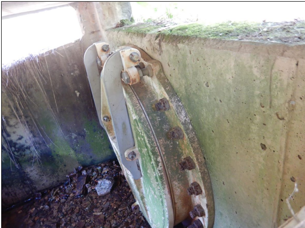
Photograph 33. Overflow Pipe, Clear Well #3 View the end of the overflow pipe that extended from Clear Well #3 and terminated below grade under a manhole. A flapper was covering the end of the pipe and it had a tight seal.
