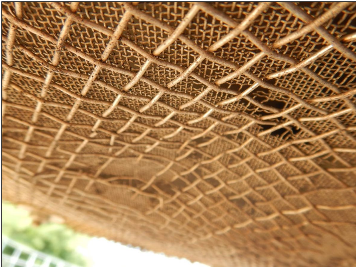
Photograph 31. Air Vent, Clear Well #3 View of the mesh screen covering the opening top one of the air vents on top of Clear Well #3. The screen was ripped and had holes.
