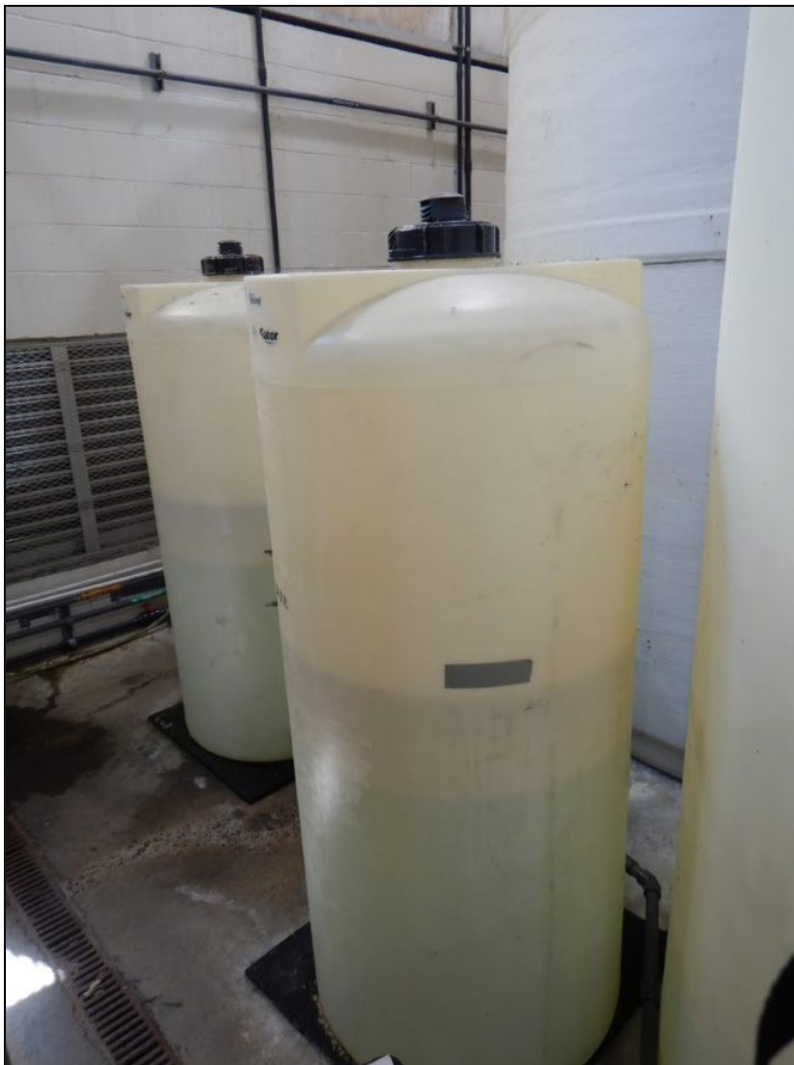
Photograph 7. Chemical Storage Room, Ouachita WTP View the two poly-orthophosphate day tanks that were present inside of the caustic soda, poly-orthophosphate, and coagulant chemical storage room.
