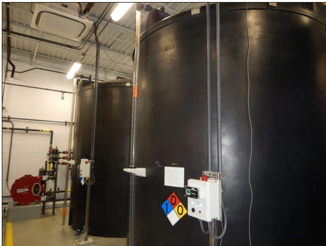
Photograph 25. Sodium Hydroxide Storage Room, Ouachita WTP View of the two, sodium hydroxide storage tanks at the Ouachita WTP. There were electronic level indicators present next to each of the tanks.
