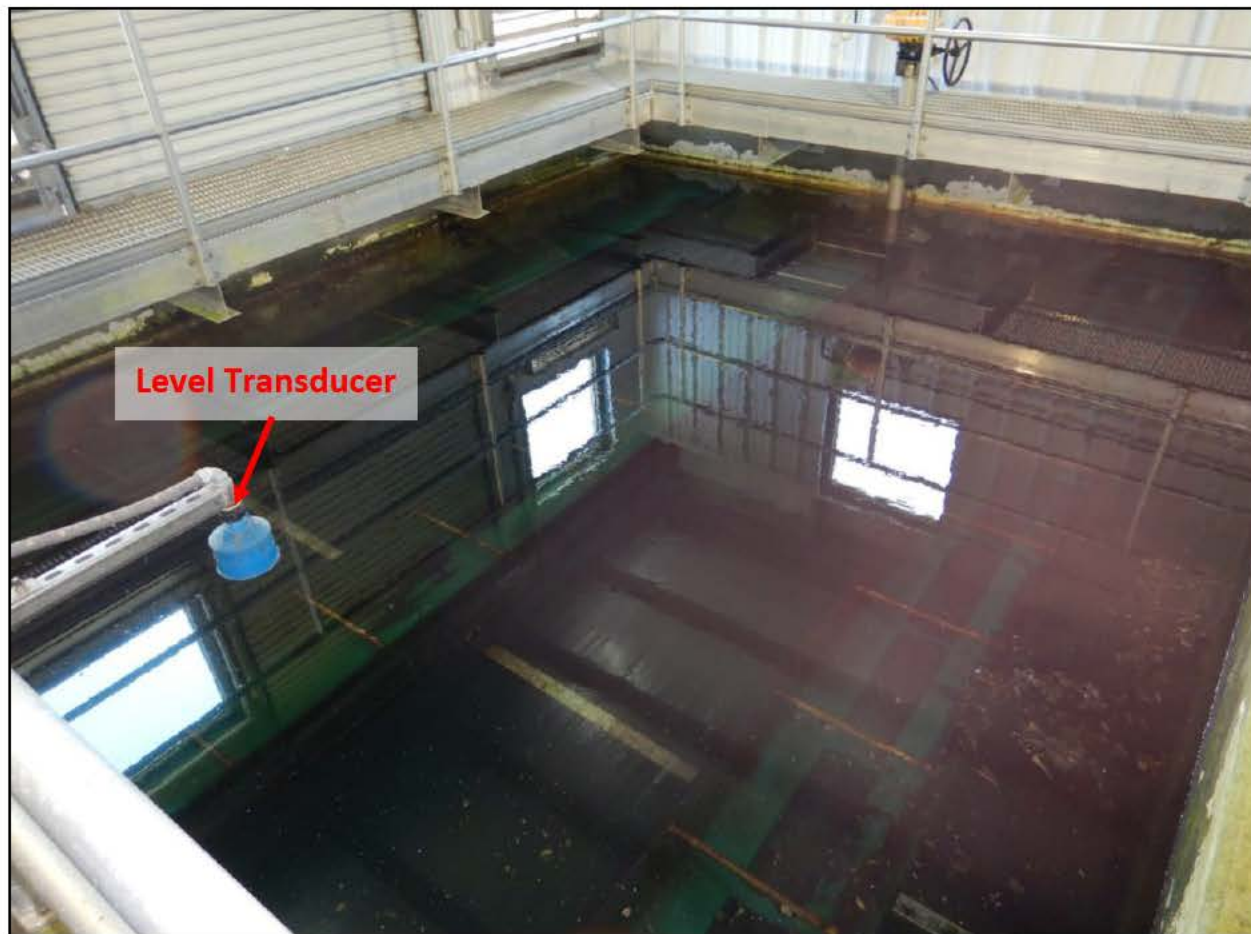
Photograph 24. Filter No. 2, Ouachita WTP View of Filter No. 2 at the Ouachita WTP. There are nine total filters at the WTP, and each contains a level transducer which determines when a backwash cycle should occur.
