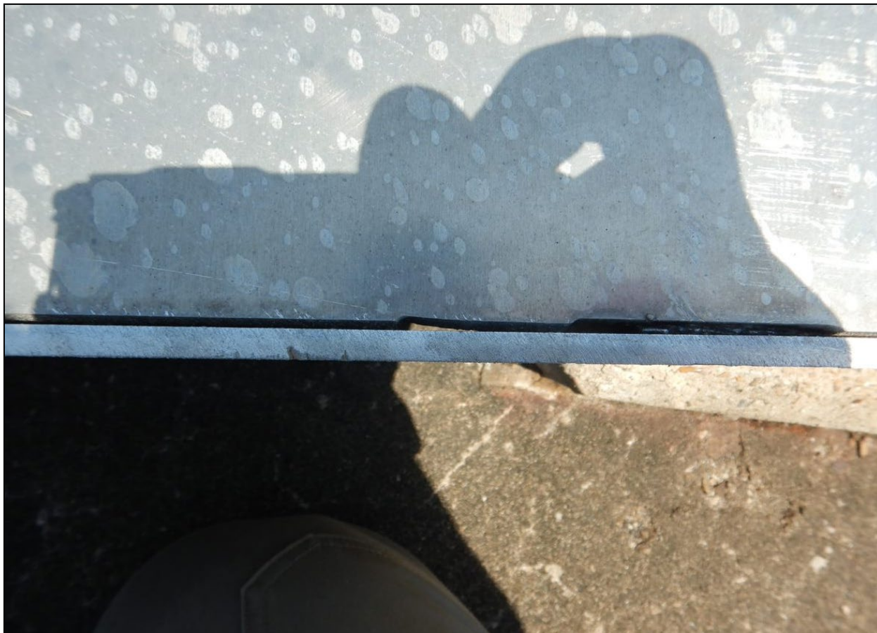
Photograph 29. Shoebox Lid, Clear Well #3 Hatchway Close up view of the seam of the shoebox lid covering the elevated hatchway leading to Clear Well #3. There was a crack in the seam that would allow rainwater to get through.
