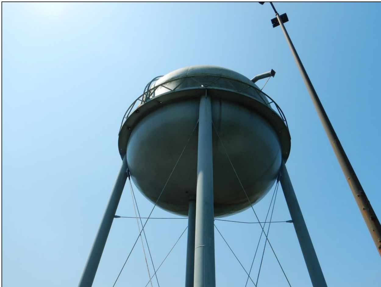
Photograph 4. Backwash Water Storage Tank View of the 100,000-gallon backwash storage tank that holds finished water until it is needed for a backwash cycle.
