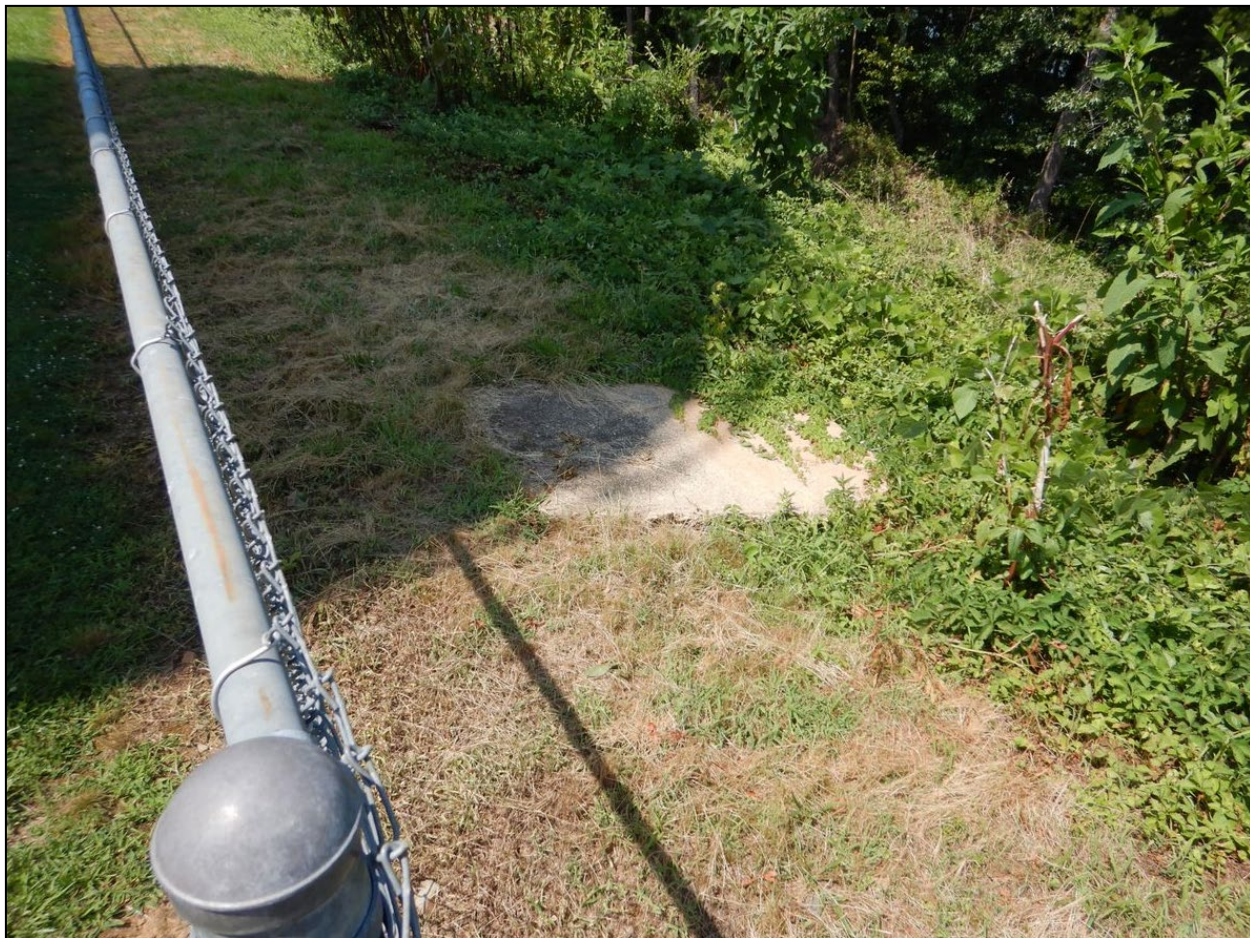
Photograph 6. Concrete Splash Pad, Backwash Storage Tank View of the concrete pad that was positioned below the terminus of the overflow pipe that extended off of the backwash storage tank. The pad appeared to be worn in the area closest to the tank
