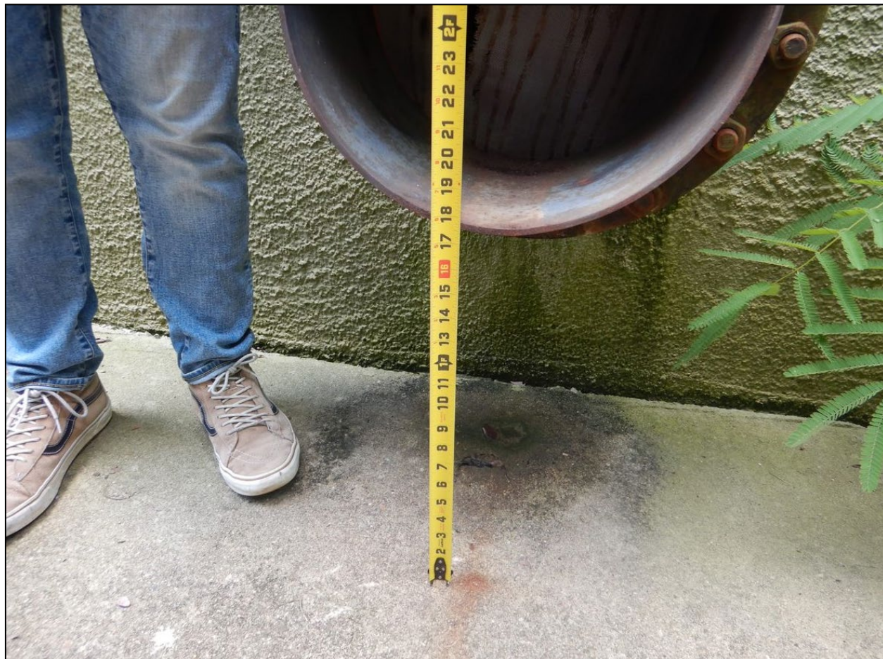
Photograph 46. Overflow Pipe, Music Mountain Water Storage Tank View of the end of the overflow pipe extending from the Music Mountain Water Storage Tank. The pipe terminated over a concrete splash pad, but it was not two pipe diameters above the pad.
