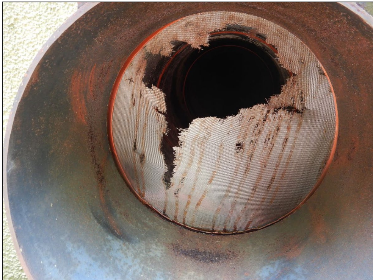
Photograph 45. Overflow Pipe, Music Mountain Water Storage Tank View of the inside of the overflow pipe that extended from the tank. The mesh screen under the flapper was ripped and had a large hole.
