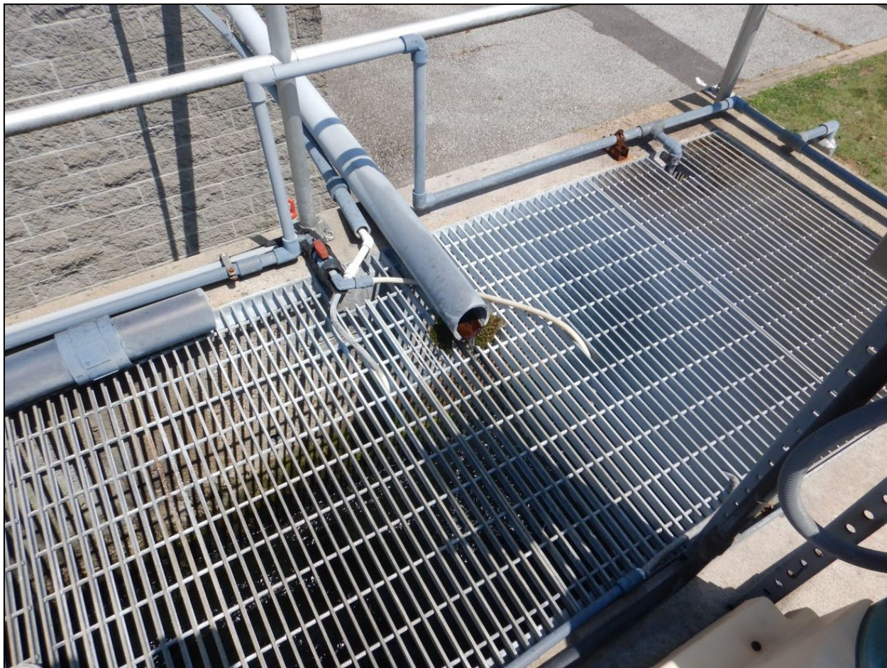
Photograph 17. Chemical Feed Lines, Ouachita WTP View of the chemical injection lines used at the rapid mix chamber at the Ouachita WTP. System representatives stated that this was where coagulant was injected.
