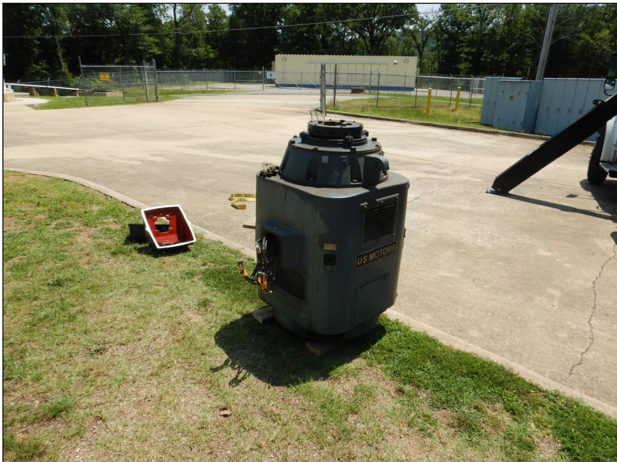
Photograph 35. Pump No. 2 Motor View of the high service Pump No. 2 motor was sitting on the ground next to the other pumps because it was under repair.
