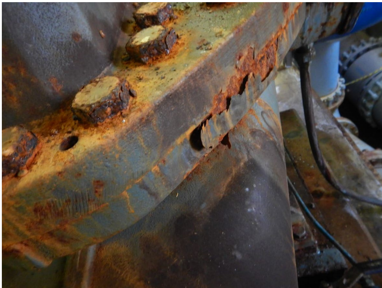
Photograph 40. Pump No. 4, Music Mountain Pump Station Close up view of the metal loss/corrosion that was taking place on the bolts and flange of Pump No. 4. The metal also appeared to be wet.
