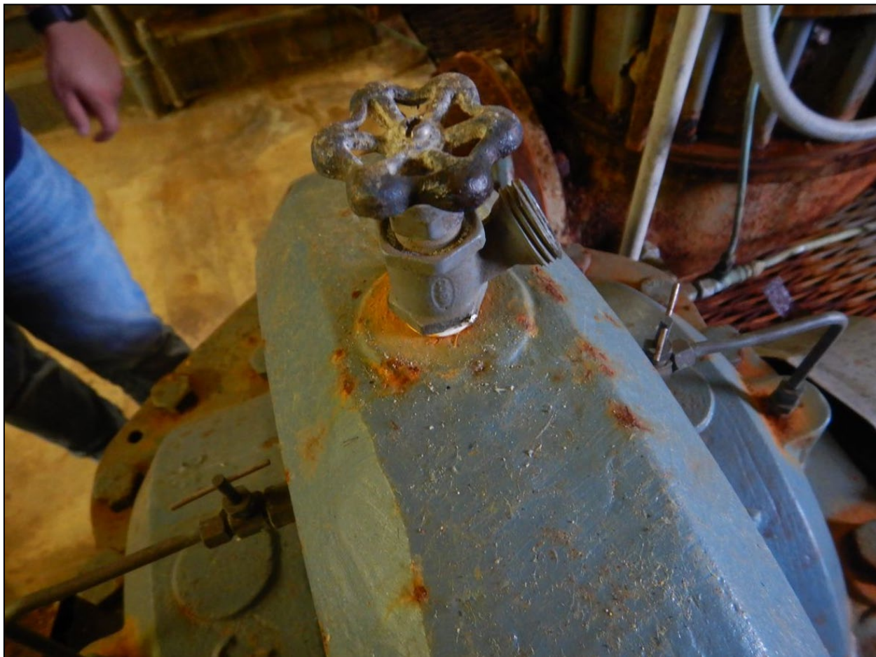
Photograph 42. Threaded Hose Tap, Music Mountain Pump Station Additional view of a threaded hose tap without backflow prevention that was extending off of a pump in the Music Mountain Pump Station.
