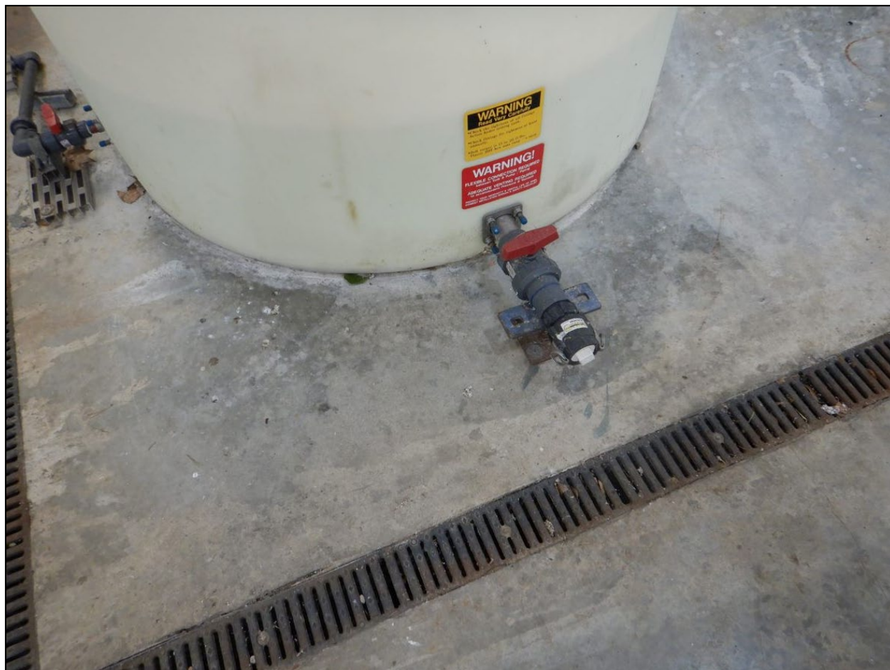
Photograph 9. Chemical Storage Room, Ouachita WTP View of the drainage on the floor surrounding the chemical tanks inside of the caustic soda, poly-orthophosphate, and coagulant chemical storage room. System representatives stated that the drain led to an onsite backwash product pond. It is unknown if this presents a concern with the plant's NPDES discharge.
