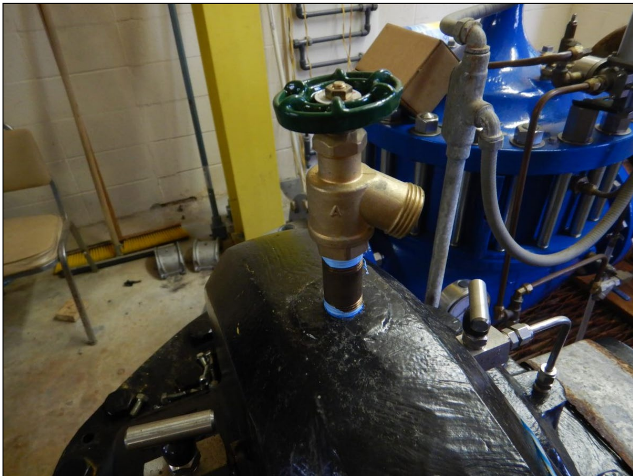
Photograph 41. Threaded Hose Tap, Music Mountain Pump Station View of a threaded hose tap without backflow prevention that was extending off of a pump in the Music Mountain Pump Station.
