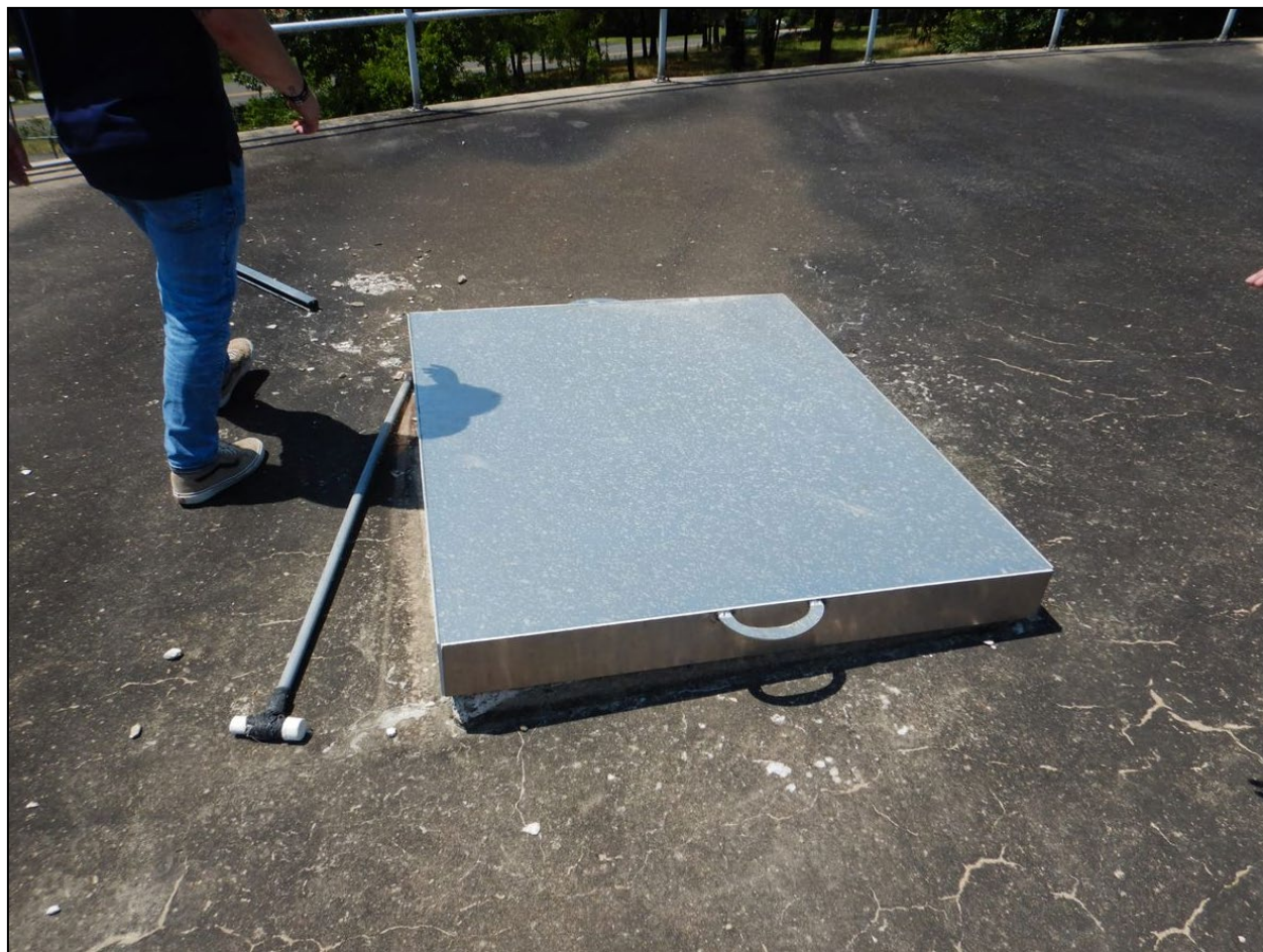
Photograph 28. Hatchway, Clear Well #3 View of the elevated hatchway leading to Clear Well #3 that was covered by a loose-fitting, shoebox style lid.
