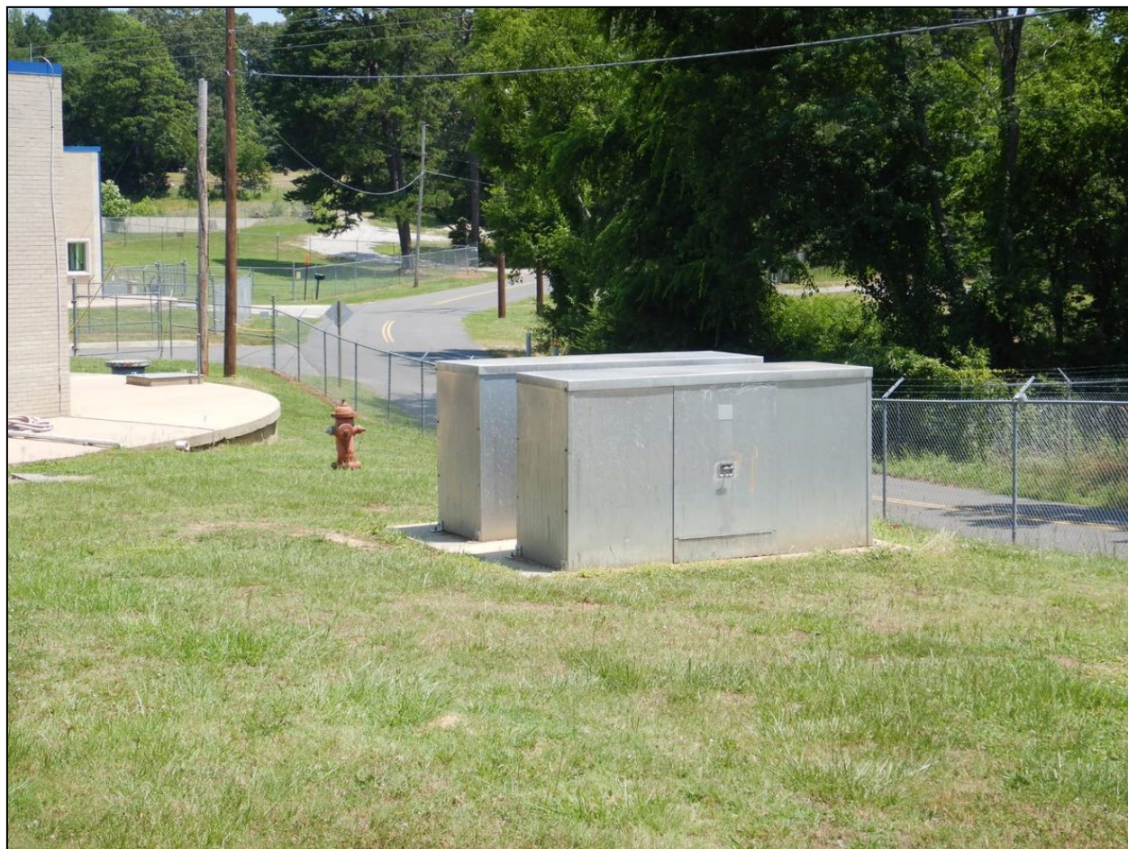
Photograph 13. RPZ Vaults, Ouachita WTP View of the two RPZ vaults containing RPZs outside of the chemical storage rooms. The RPZs are used to create backflow prevention.
