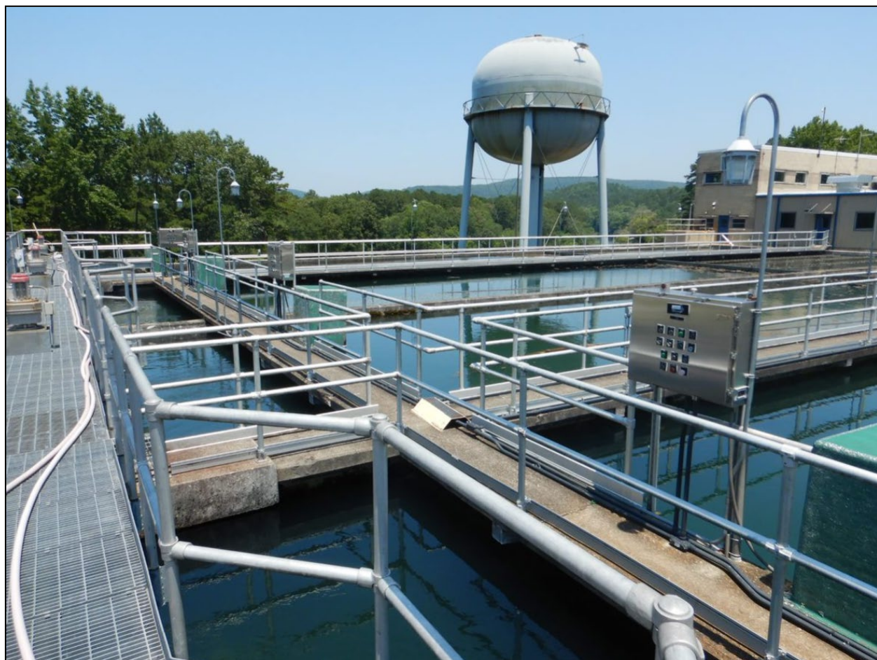
Photograph 18. Sedimentation Basin Nos. 1-3, Ouachita WTP View of Sedimentation Basin Nos. 1-3. Not pictured are Basin Nos. 4 and 5, which are also clustered in this area.
