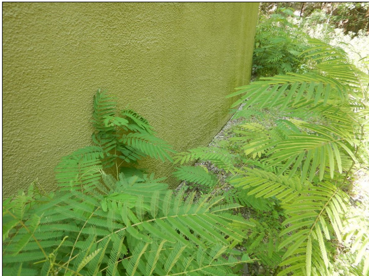
Photograph 47. Music Mountain Water Storage Tank View of the back of the Music Mountain Water Storage Tank. There were plants growing against the back wall of the tank and System representatives stated that the mowing crews had not been mowing behind the tank.
