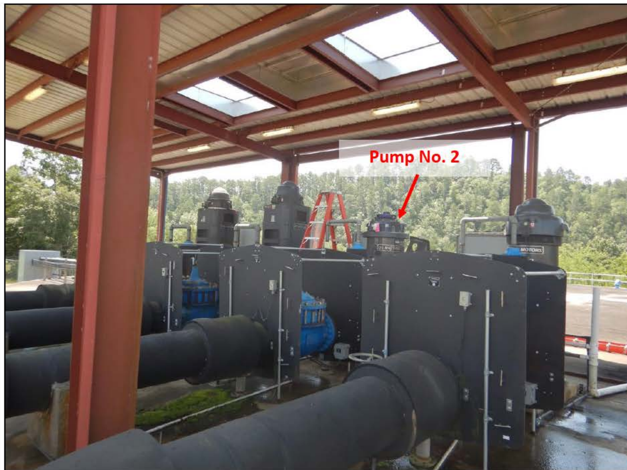
Photograph 34. High Service Pumps, Ouachita WTP View of the four high service pumps that are used to pump finished water from Clear Well #3 into the distribution system. Pump No. 2 was offline during the inspection because the motor was being repaired.
