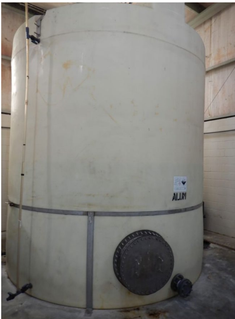
Photograph 8. Chemical Storage Room, Ouachita WTP View the coagulant storage tank that was present inside of the caustic soda, poly-orthophosphate, and coagulant chemical storage room.
