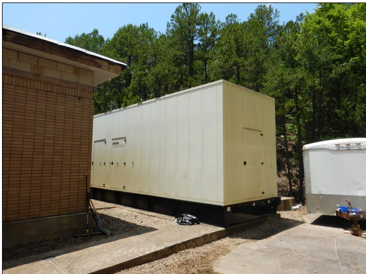
Photograph 43. Backup Generator, Music Mountain Pump Station View of an emergency backup generator that was present outside of the Music Mountain Pump Station. The Water Production Manager stated that it would turn on automatically in the event of a power outage.
