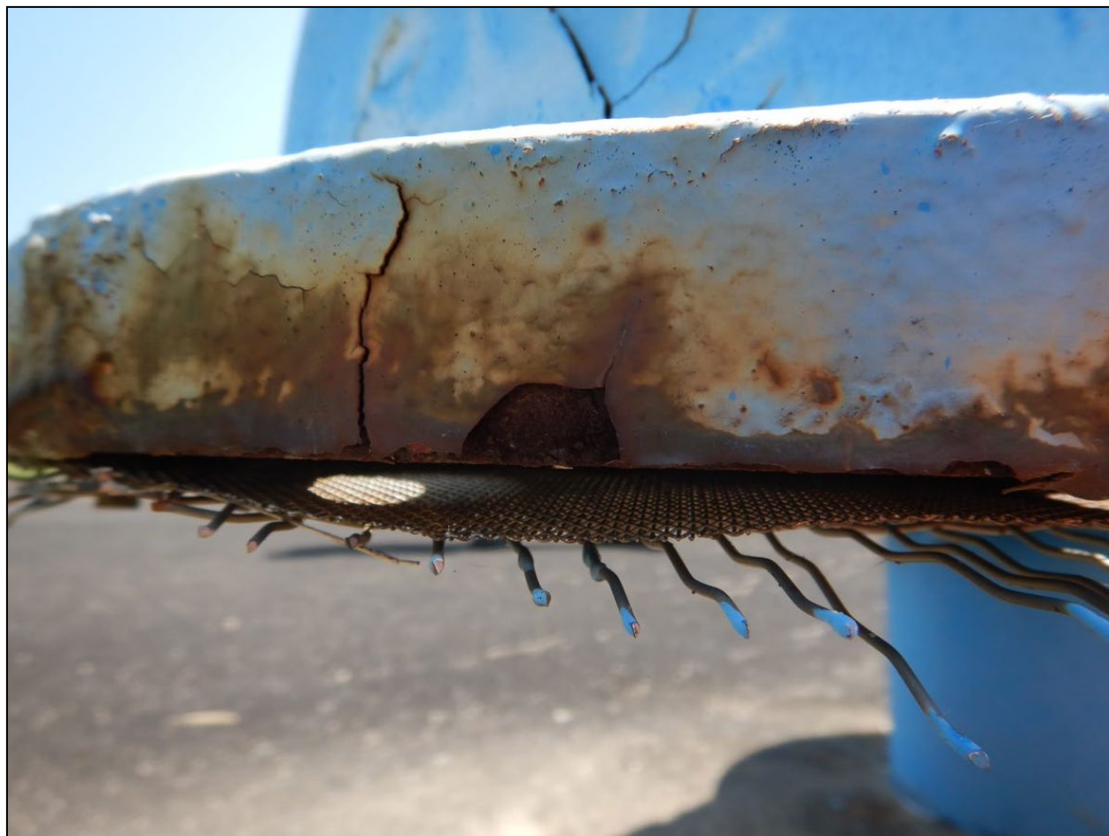
Photograph 32. Air Vent, Clear Well #3 Side view of a mesh screen covering the opening top one of the air vents on top of Clear Well #3. The screen was not securely fastened to the opening, creating a large hole.
