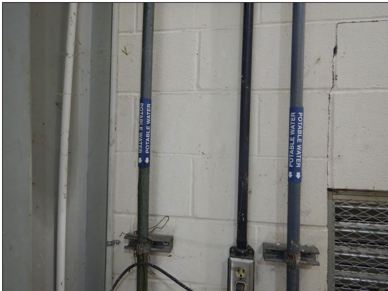
Photograph 11. Potable Water Lines, Chemical Storage Room, Ouachita WTP View of the potable water lines used to inject carry water for chemical addition in the caustic soda, poly-orthophosphate, and coagulant chemical storage room. These individual lines did not contain backflow prevention, but System representatives stated that an RPZ outside the building created backflow prevention for this entire building.
