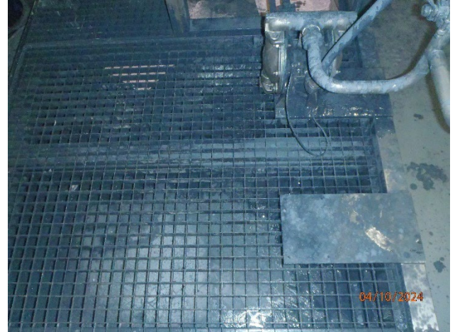
Picture 9 – Primer Purge Recovery System secondary containment for pump
