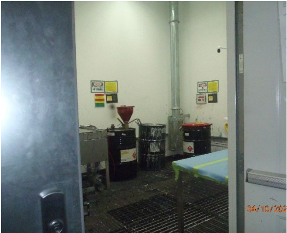
Picture 7 – Paint Shop Paint Mix Room SAA
