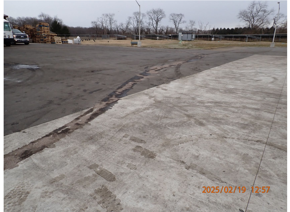
P2190044 – Quick dry over hydraulic fluid leak.
