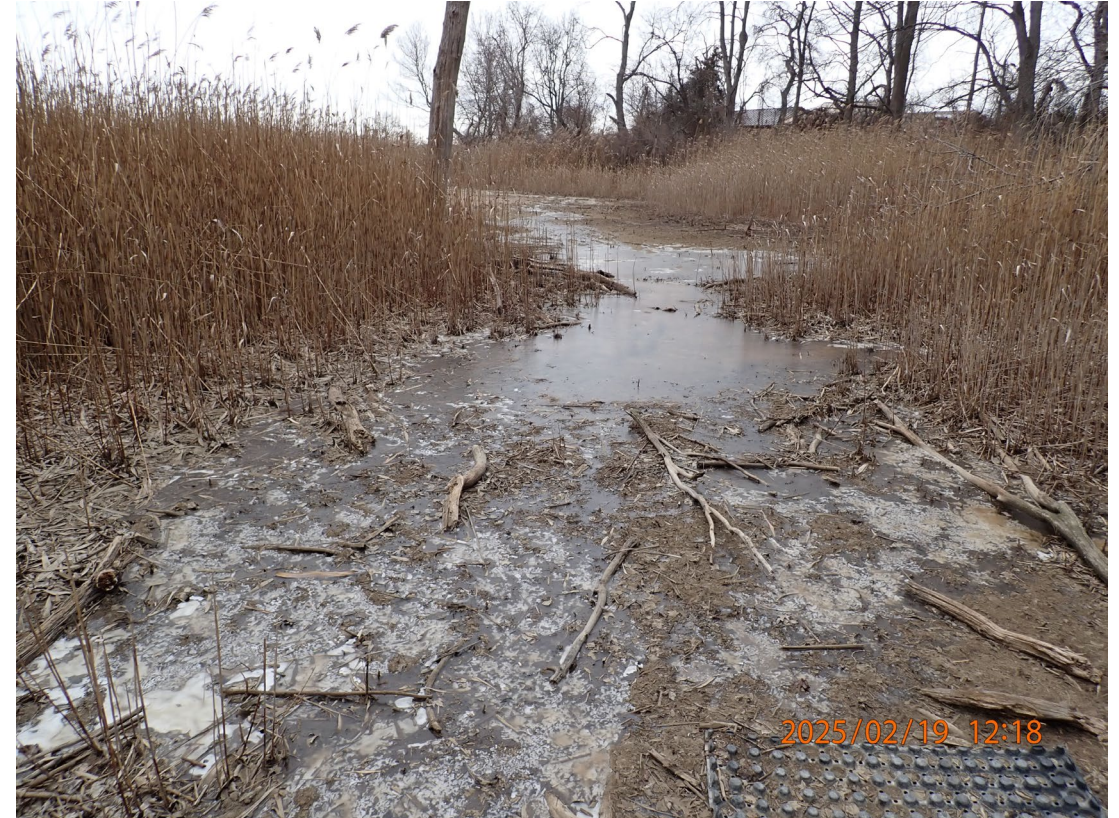
P2190020 – Frozen, unauthorized discharge leaving the southeastern portion of the spray field.
