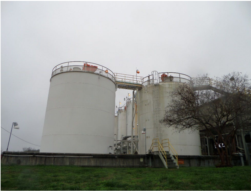
Photograph 7: Hazardous Waste Tank Farm
