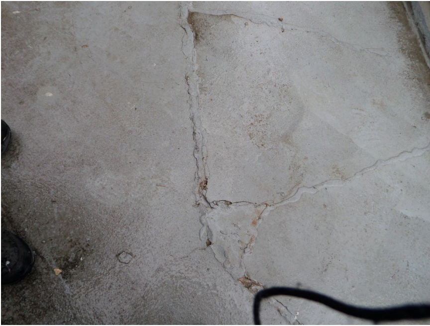
Photograph 11: Some Minor Cracking in Coating
