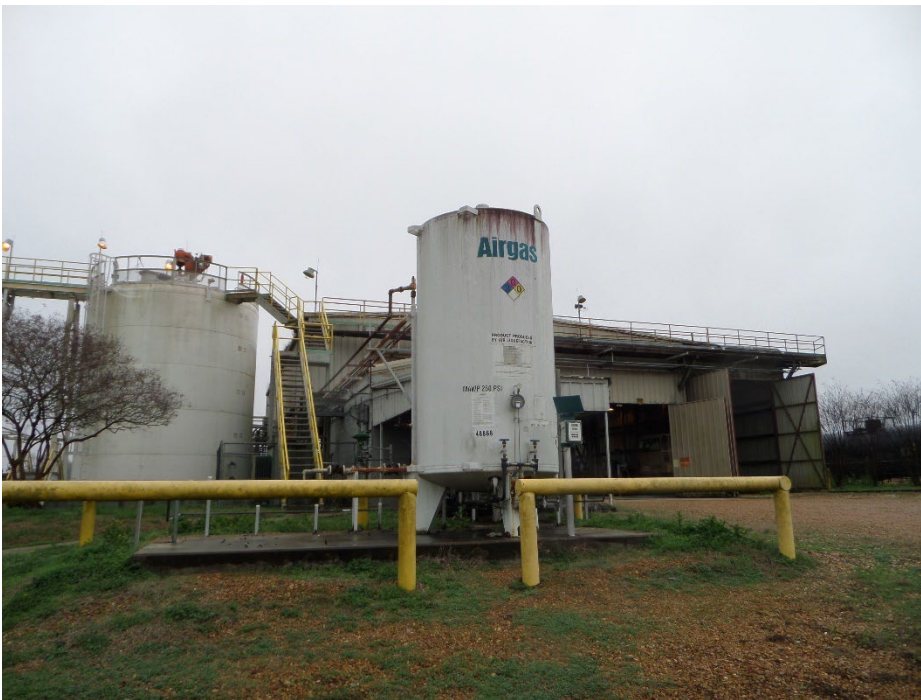
Photograph 8: Nitrogen Tank for Hazardous Waste Tank Farm and Piping
