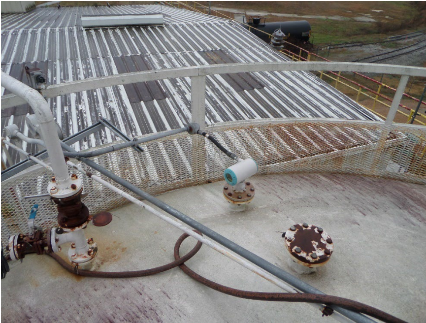
Photograph 18: Missing Coating and Corrosion on Top of Tank 4105
