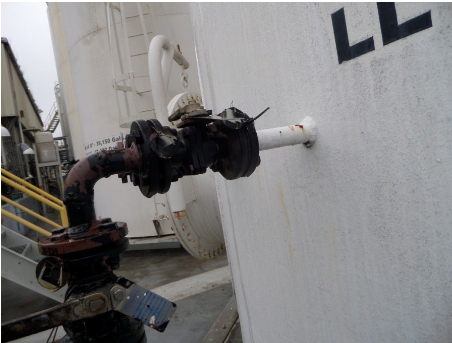
Photograph 13: Missing Coating & Corrosion and Obscured LDAR (Subpart BB) Tags
