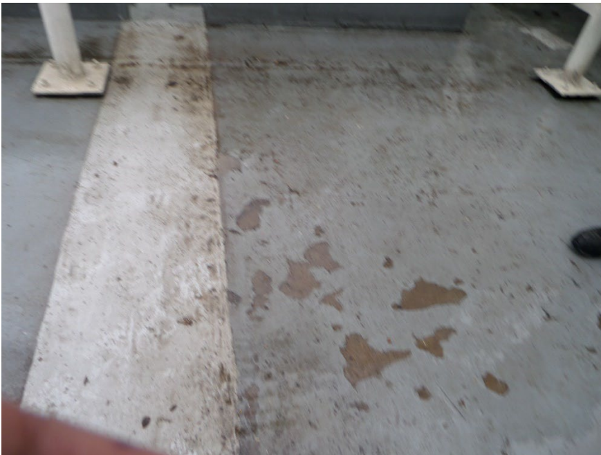
Photograph 10: Missing Coating in Tank Farm
