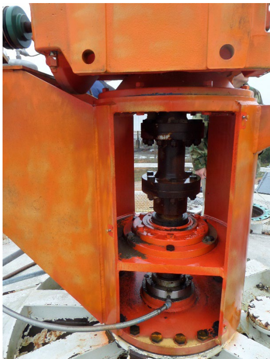
Photograph 19: Impeller Motor, Some Corrosion Visible on Tank Around Impeller Motor Base
