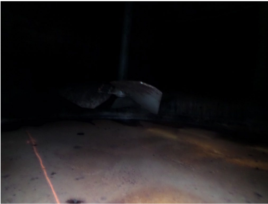
Photograph 9: Picture of Bottom Impellar in Tank 4105
