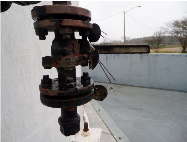
Photograph 15: Illegible LDAR Tags on Ancillary Equipment Subject to Subpart BB
