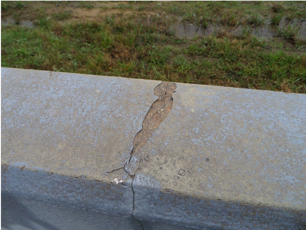
Photograph 12: Hairline Crack in Containment Wall and Missing Coating
