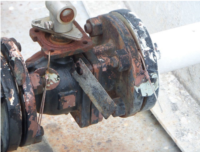
Photograph 14: Illegible LDAR Tags on Ancillary Equipment Subject to Subpart BB
