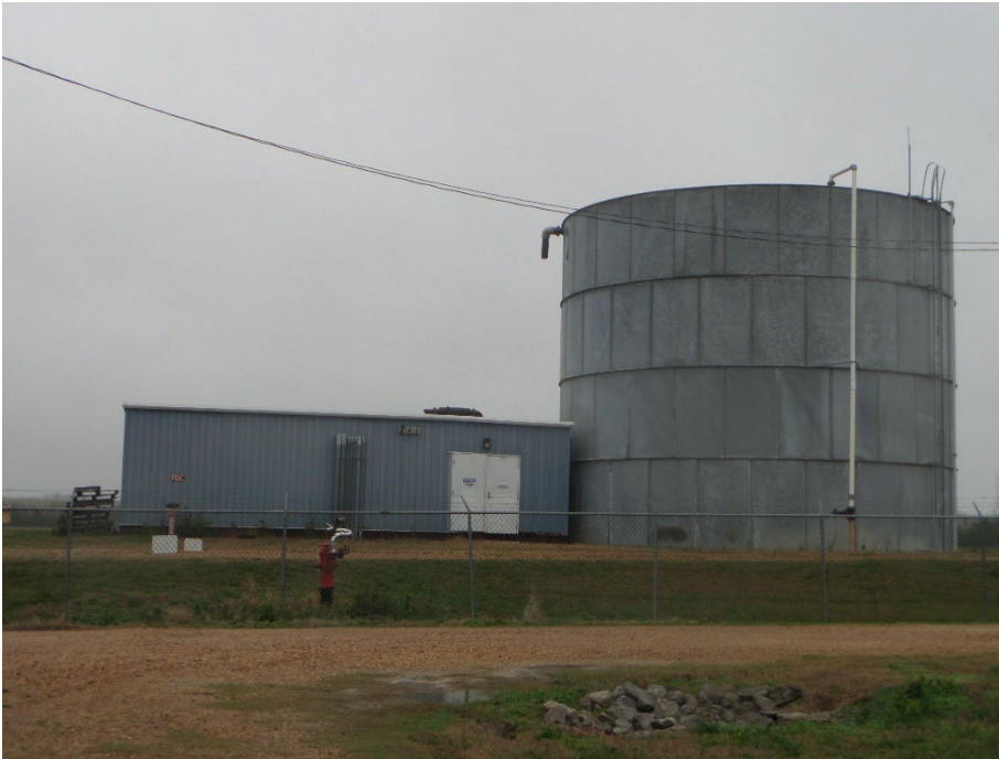
Photograph 1: Water Cannon and 250,000-gallon Water Tank
