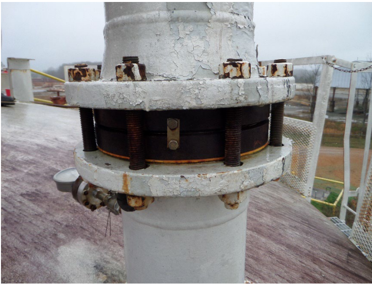
Photograph 17: Corrosion on Connector & Bolts
