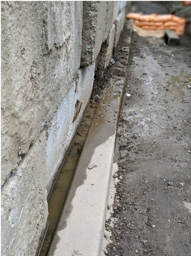
Photograph 15 of 30: Liquid that Appears to be Seeping Through the Wall
