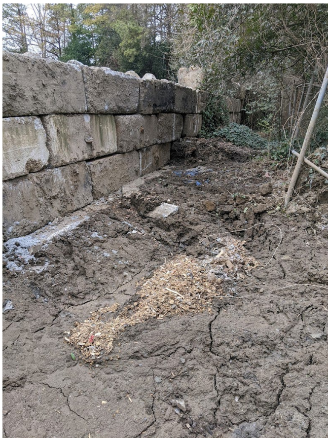
Photograph 13 of 30: Debris Settling in Jig Pad Area Behind Wall
