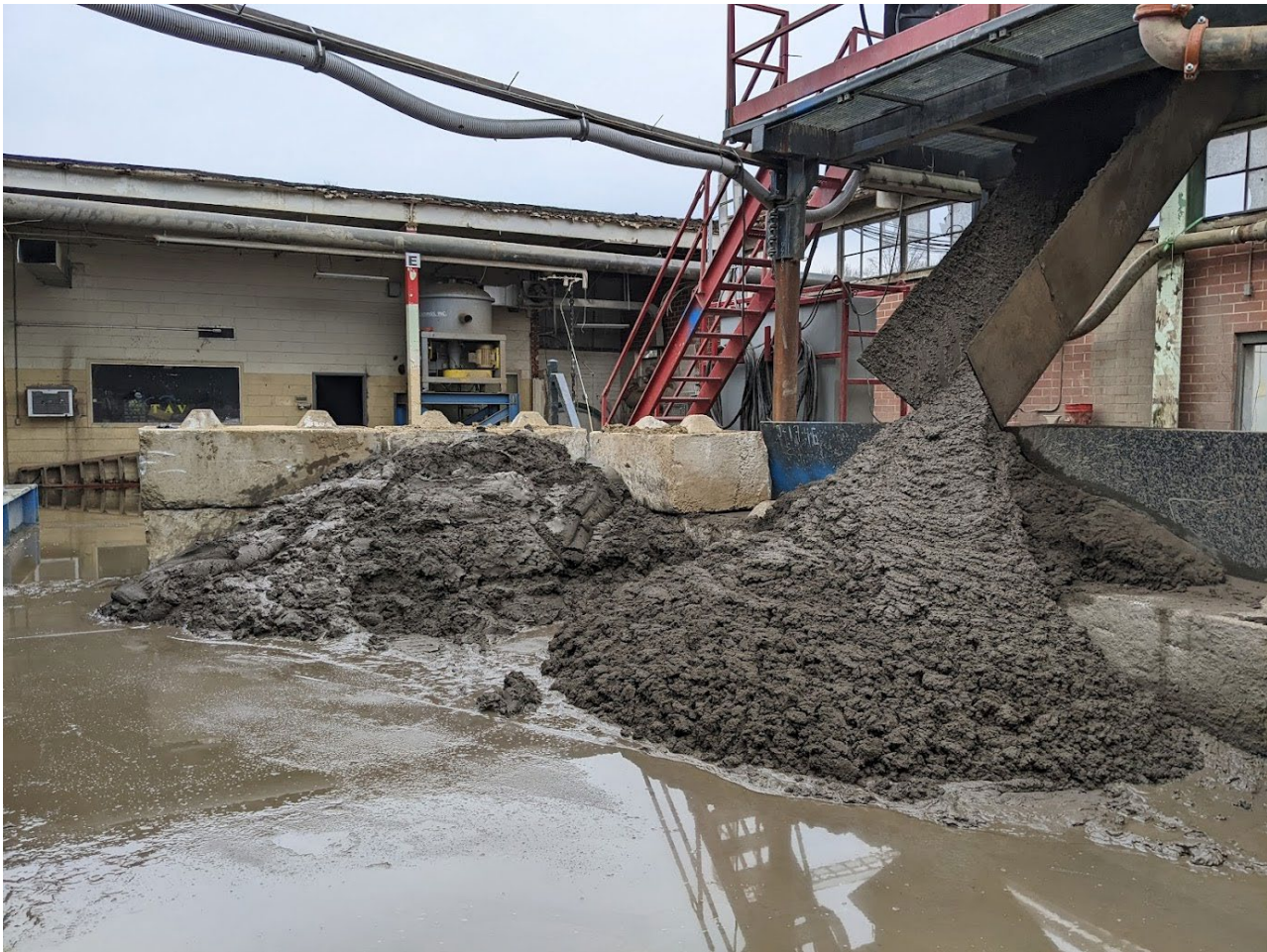
Photograph 19 of 30: Sludge from Centrifuge
