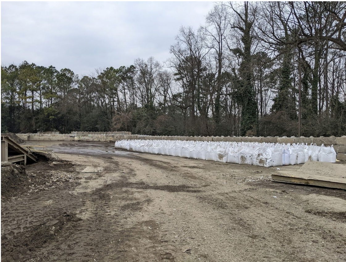
Photograph 4 of 30: Jig Pad Area with New Wall Addition and Super-Sacks
