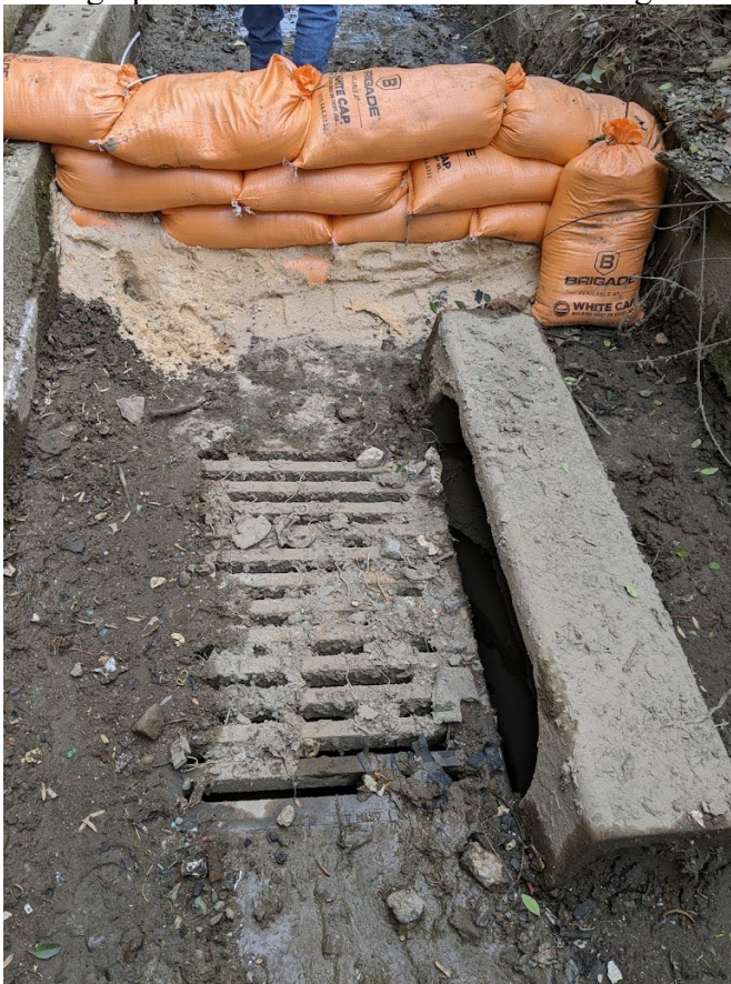
Photograph 11 of 30: Close up of Storm Drain with Debris Behind Jig Pad Wall
