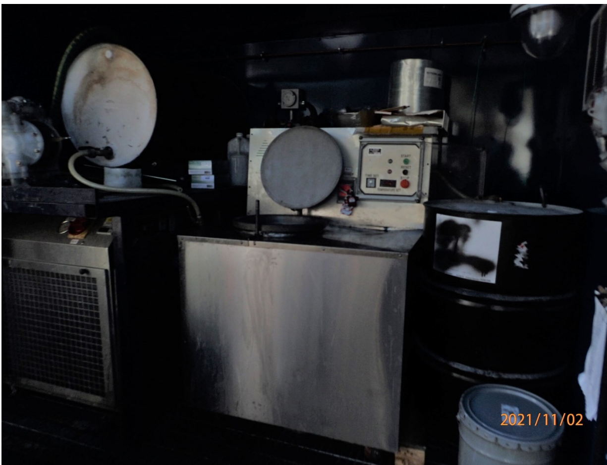
Photo 2: Acetone Recovery Unit. Not currently operating.
