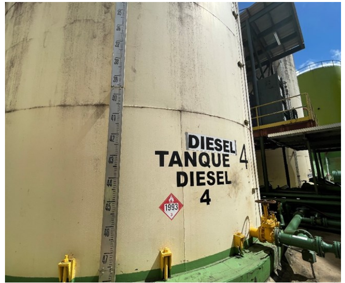
Picture 22 - OIL ENERGY SYSTEMS- At the Tank #4 Diesel Storage Area there was one (1) aboveground Tank #4 with storage capacity of 211,596-gallons used to store Diesel product that belongs to Trans-Fuel Company.
