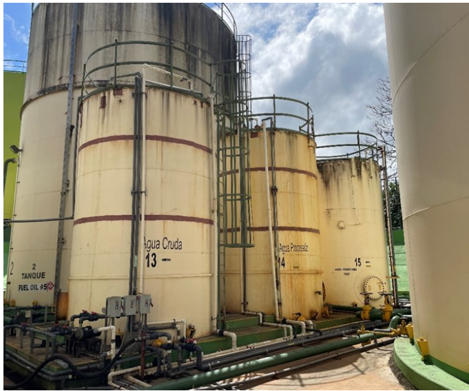
Picture 21- OIL ENERGY SYSTEMS — At the Used Oil/ Water Storage Area there was one (1) aboveground Tank #5 with storage capacity of 211,596-gallons used to store used oils/water mixture at the generator facility was not labeled or marked clearly with the words “Used Oil.”
