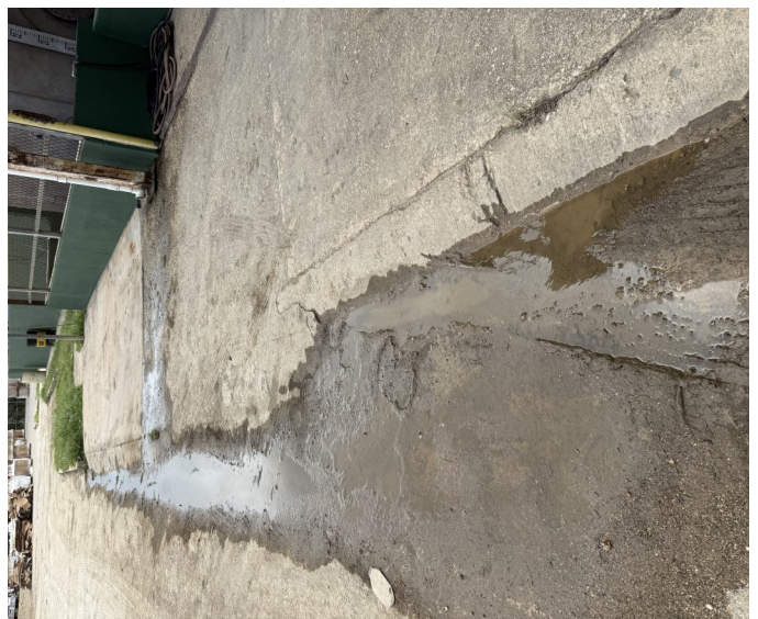
Picture 32 - OIL ENERGY SYSTEMS- At the Sidewalk Area there was an oil spill running toward a rainwater sewage system,
