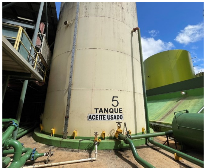
Picture 20 - OIL ENERGY SYSTEMS- At the Used Oil/ Waster Storage Area there was one (1) aboveground Tank #5 with storage capacity of 211,596-gallons used to store used oils/ water mixture at the generator facility was not labeled or marked clearly with the words “Used Oil.”
