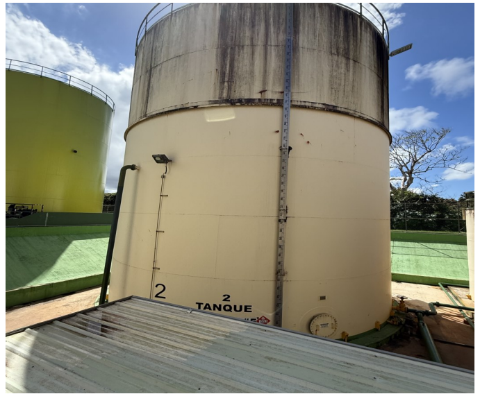
Picture 18 - OIL ENERGY SYSTEMS- At the Tank #2 Decanting Fuel Oils Storage Area there was one (1) aboveground Tank #2 with storage capacity of 422,382-gallons used to store and fuel oils mixed with used oil at the generator facility was not labeled or marked clearly with the words “Used Oil.”
