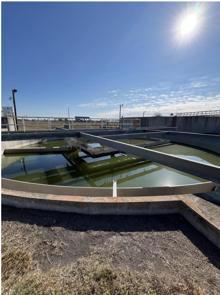
Clarifier #1 Out of Service with Cracked Well
