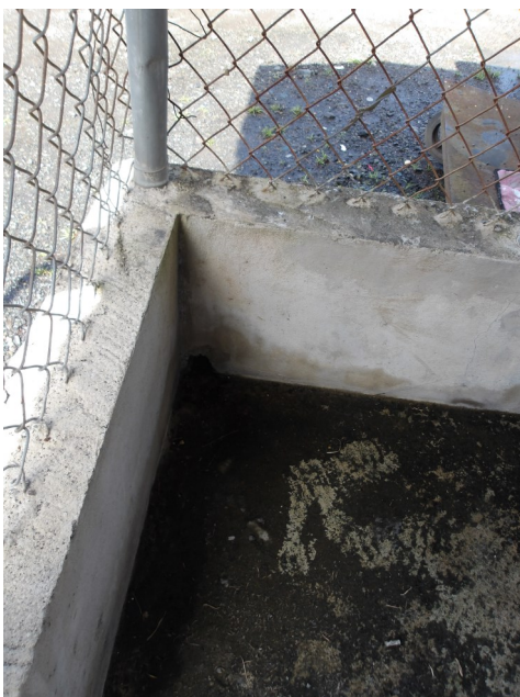
Picture 100-057 Inside view of HWSA controlled valve
