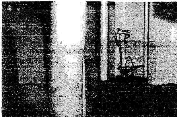
High water mark on the engineroom-pumproom bulkhead. A cargo pump turbine is at left.
