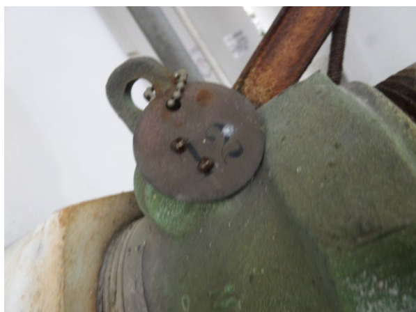
Figure 21: 11:54 AM Tank Farm
