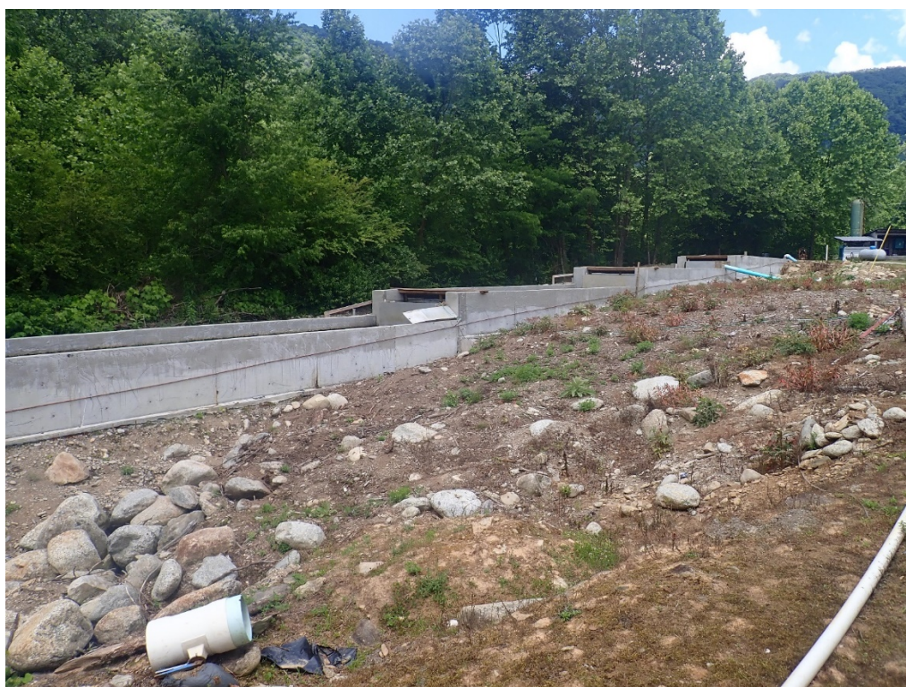
Photo 1. Six unpermitted raceways found operational.
