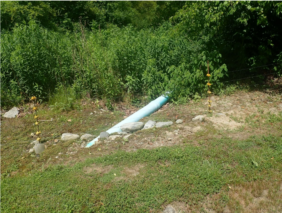
Photo 4. Pipe leading from unpermitted raceways to main raceway series.
