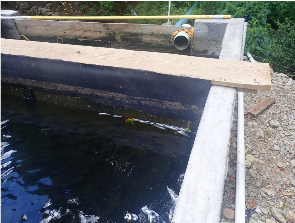
Photo 2. Trout seen swimming in final raceway of unpermitted raceways. Above pipe serves as overflow leading directly to riverbed. Background pipe discharges to main raceway series.
