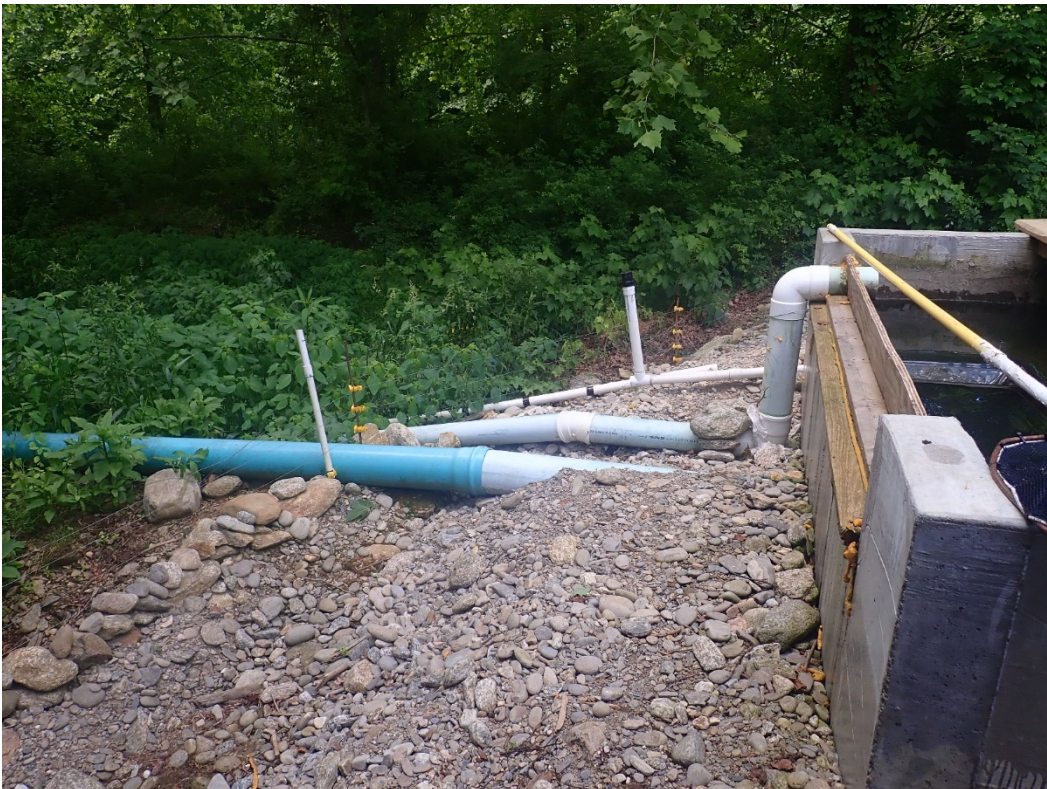
Photo 3. Side view of unpermitted effluent showing main outlet and overflow.
