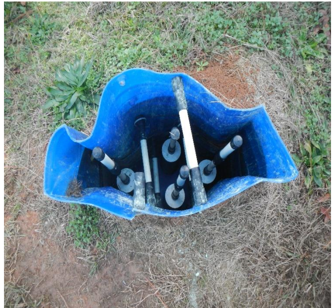
Photo 8. Sodium Sulfate tablet de-chlorination Tank.
