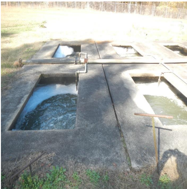
Photo 7. Chlorine contact Chamber.
