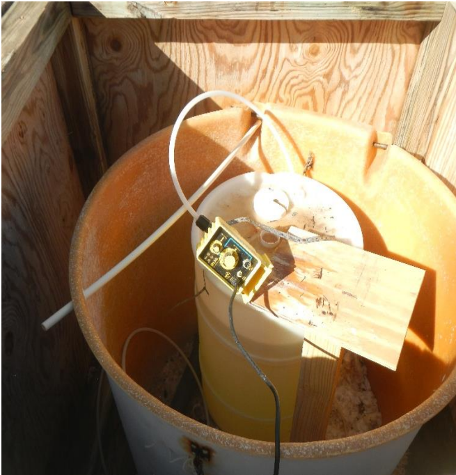
Photo 5. Liquid Chlorine tank.
