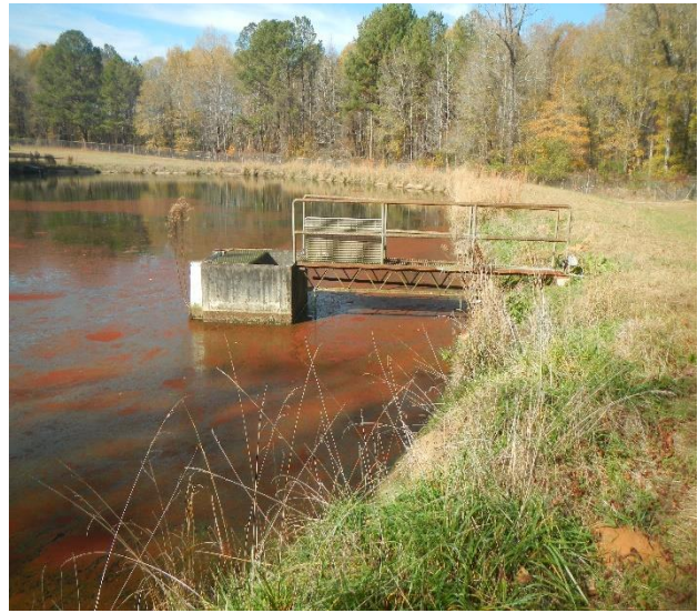
10. Vegetative growth observed inside the perimeter of the lagoon near the water line.
