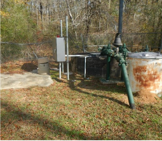
Photo 1. Influent pump station.
