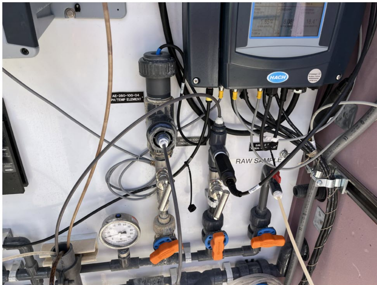
View of some of the process sampling equipment. (IMG_0018) (July 10, 2024: 2:01 PM) Photographed by D. Esparza
