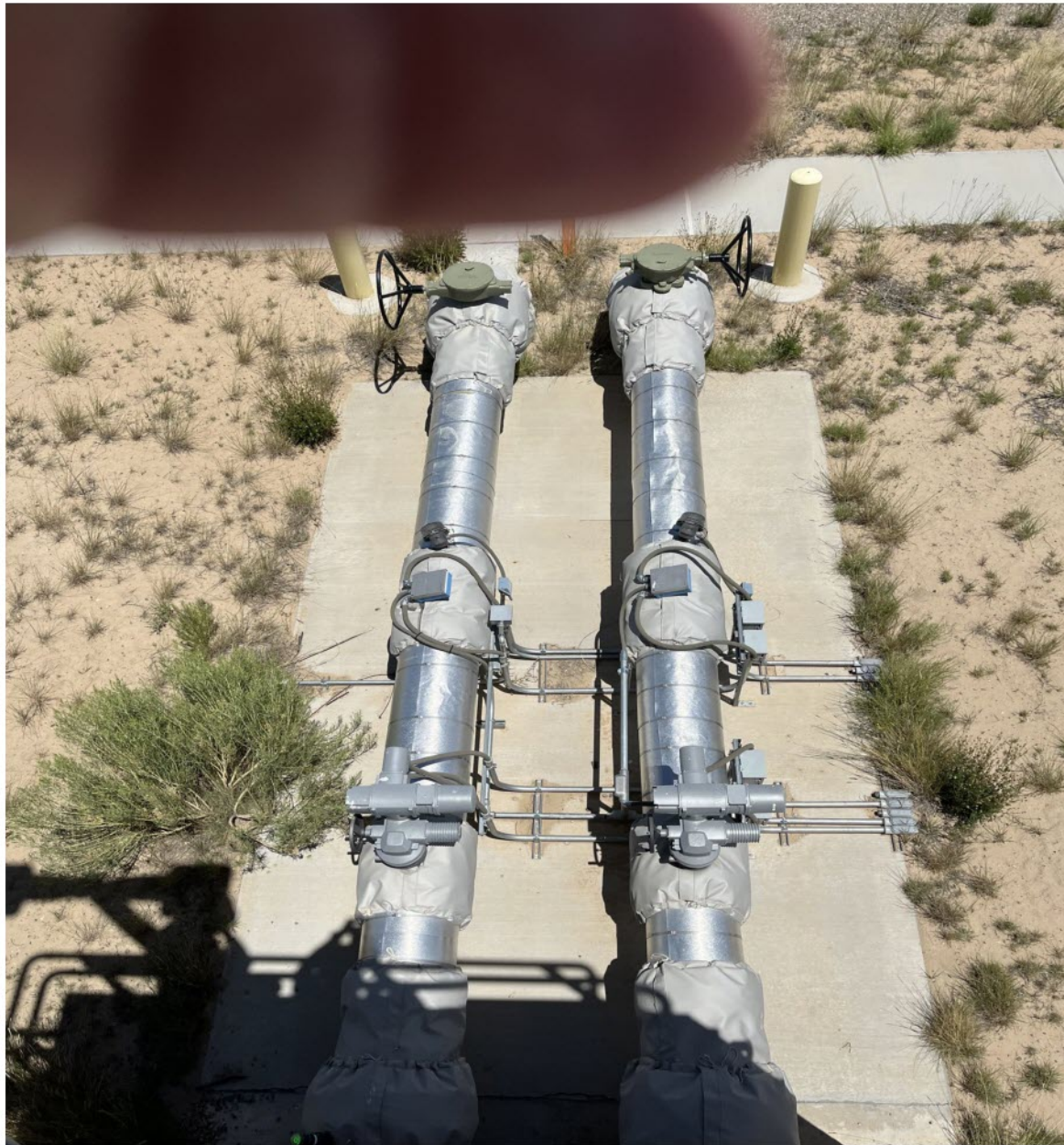
View of the raw water influent lines delivered from Pumping Plant #2 prior to the Rapid Mix process. (IMG_0013) (July 10, 2024: 1:51 PM) Photographed by D. Esparza
