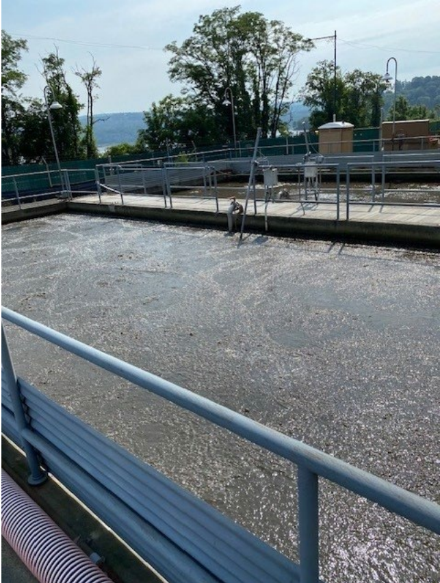
Photo #4: Target Hill Aeration Tank
