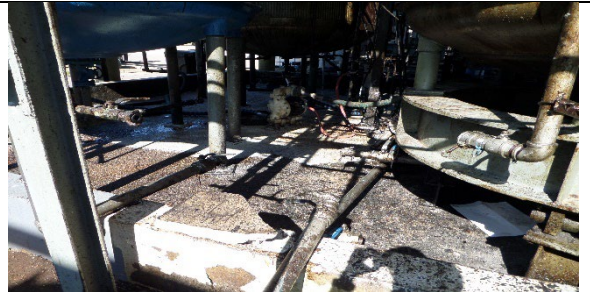
Photo-7 Production Area #3, Chipped secondary containment wall
