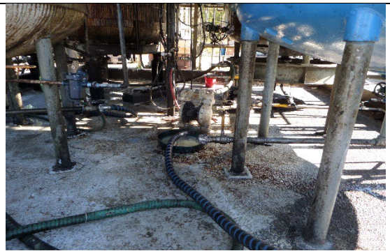
Photo-5 Production Area #3, Open drip pan and solid debris inside the containment area
