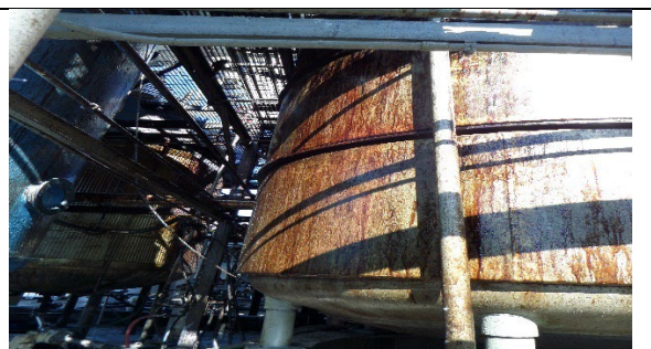
Photo-8 Production Area #3, Stained walls of the Reactor
