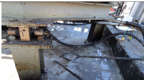
Photo-10 Production Area #3 Water dripping from one of the Reactor leg bracings
