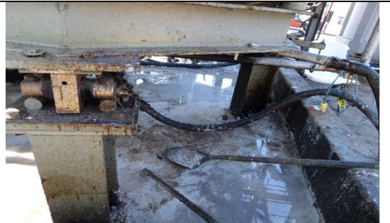
Photo-6 Production Area #3, Open drip pan and solid debris inside the containment area
