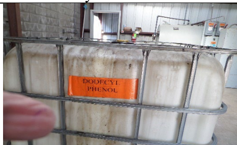
Photo-27 Dodecyl Phenol Material in the Boiler Room
