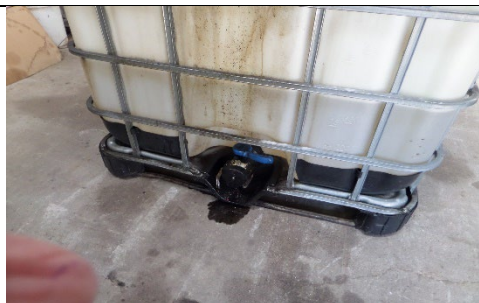
Photo-28 Leaking Waste Dodecyl Phenol Material in the Boiler Room
