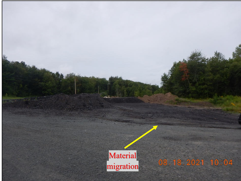
Photograph 23. Municipal Salt Storage Shed: (DSCN0720) View, facing west, of two asphalt road fill piles and one pile of soil stored west of the salt storage shed. Note the lack of cover, impermeable containment, and migration of material from the piles to the north.
