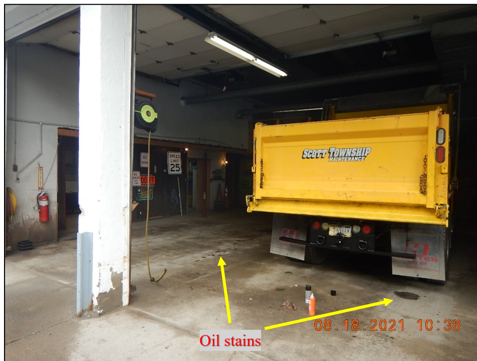
Photograph 27. Municipal Garage: (DSCN0727) View, facing southwest, of the interior of the municipal garage. Note the presence of oil stains on the floor.
