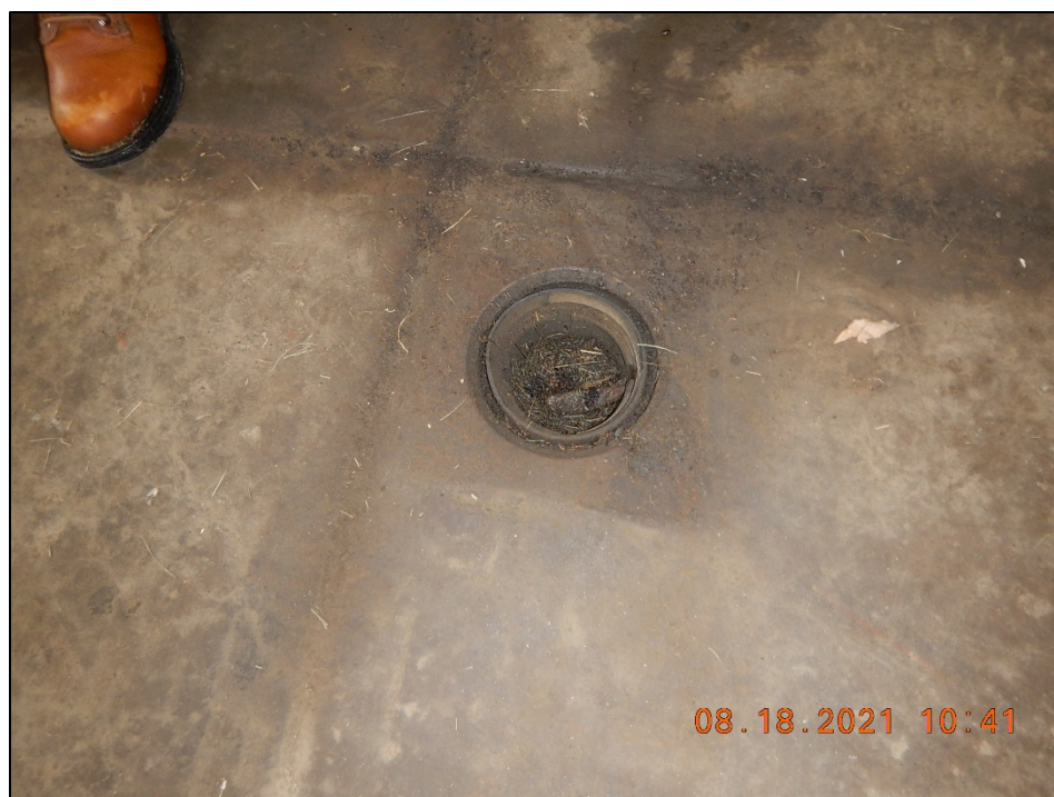
Photograph 28. Municipal Garage: (DSCN0732) View of a drain plug inside of the municipal garage.
