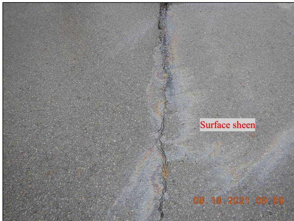
Photograph 8. Outfall #2: (DSCN0705) View of surface sheen that appears to be emanating from a crack in the pavement.
