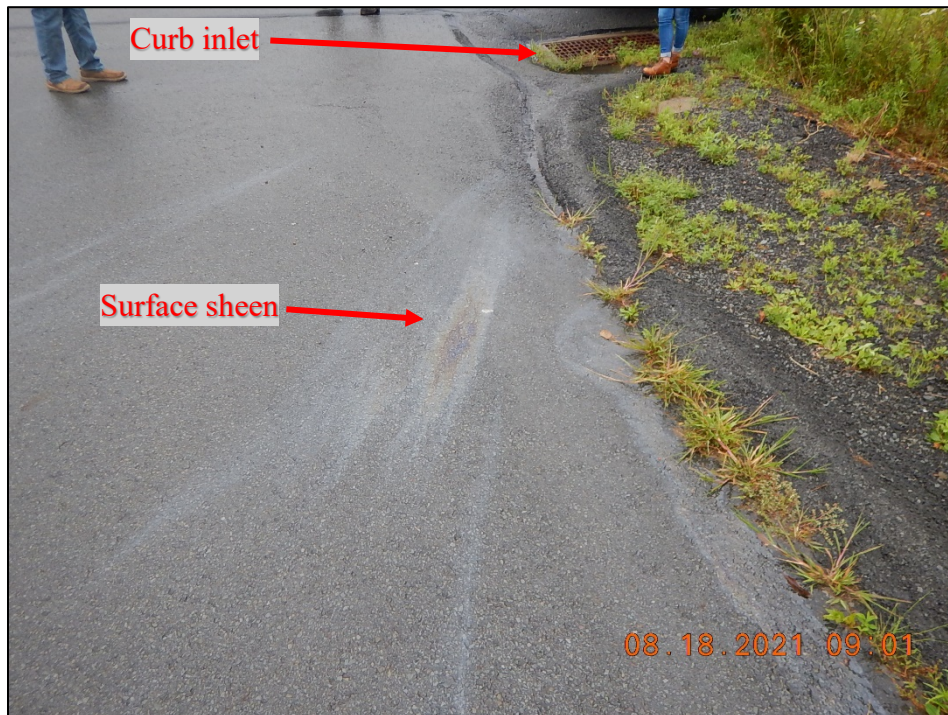
Photograph 4. Outfall #2: (DSCN0698) View, facing south, of surface sheen running down Meadow Drive towards the curb inlet shown in Photograph 6.
