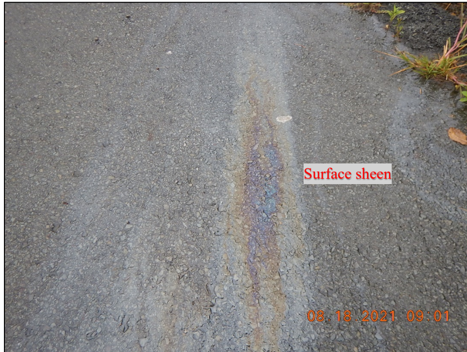
Photograph 5. Outfall #2: (DSCN0699) Close-up view, facing south, of the surface sheen shown in Photograph 7.
