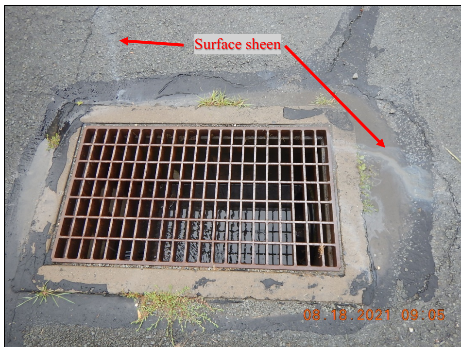
Photograph 6. Outfall #2: (DSCN0703) View, facing south, of the next most upgradient inlet from Outfall #2. Note the surface sheen flowing into the inlet.
