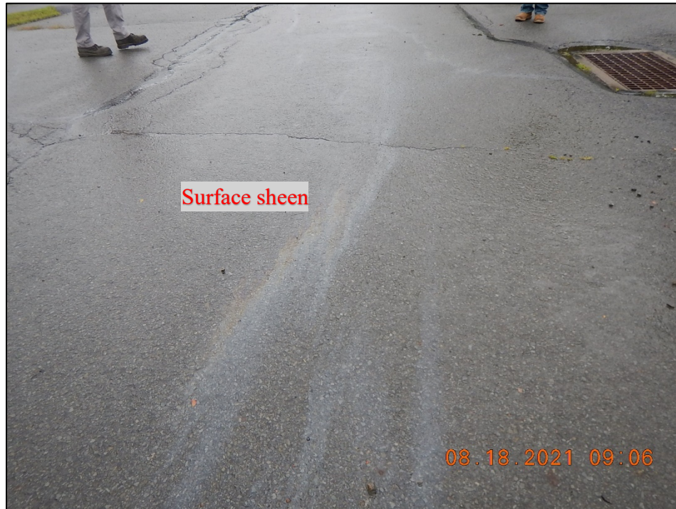
Photograph 7. Outfall #2: (DSCN0704) View, facing west, of surface sheen flowing along Laurel Drive to the inlet shown in Photograph 9.
