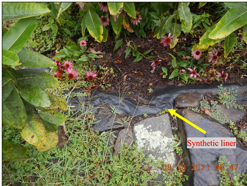
Photograph 16. Municipal Building Rain Garden: (DSCN0697) View of a synthetic liner beneath the municipal building rain garden.
