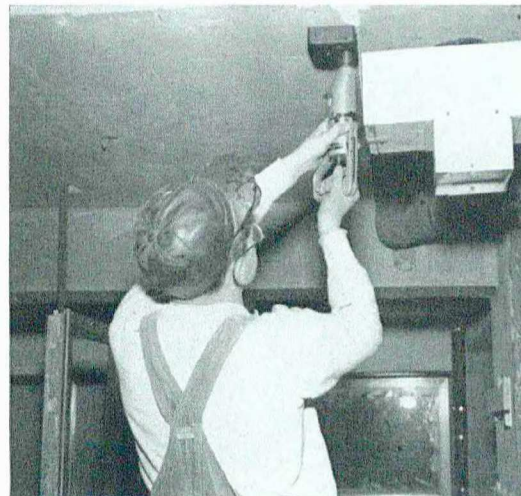
Hanging ductwork from a concrete ceiling. Alloy steel studs are seated firmly in concrete, steel.
