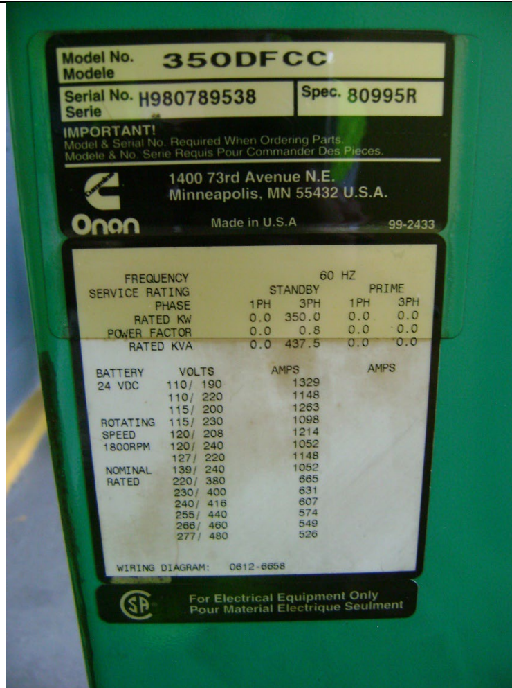
Plate on emergency generator.
