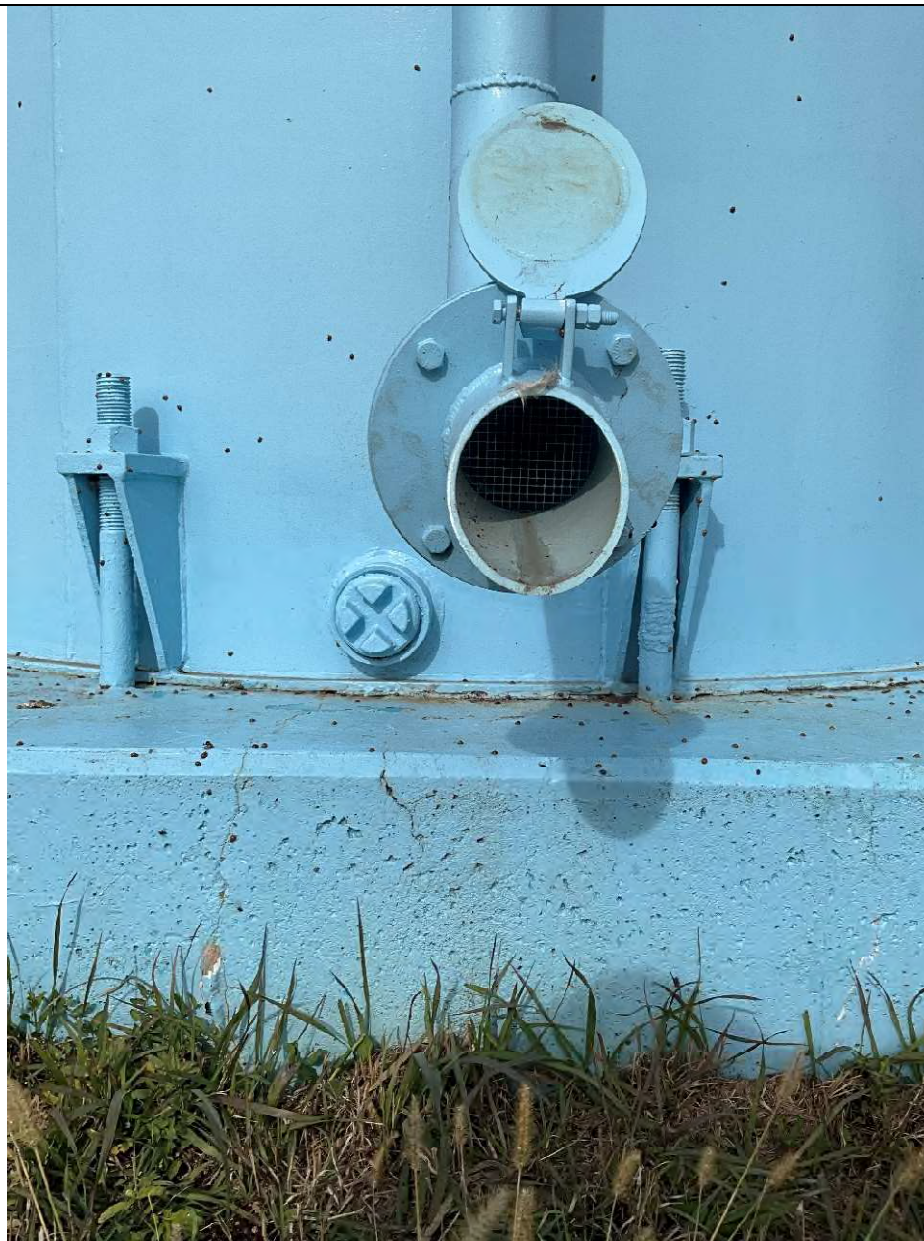
Cuba Tower overflow extended to 12-24" above the ground with screen
