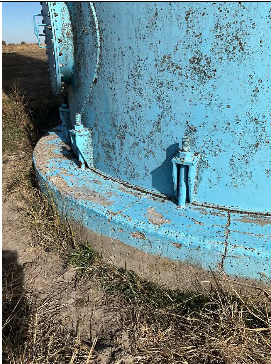
Mildew accumulation on exterior paint and cracks in the concrete base of the Francis Tower
