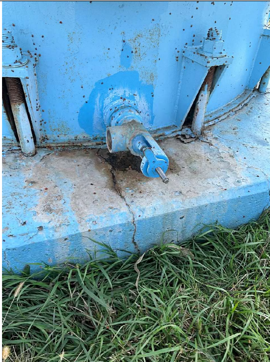
Narka Tower drain valve and concrete base with cracking
