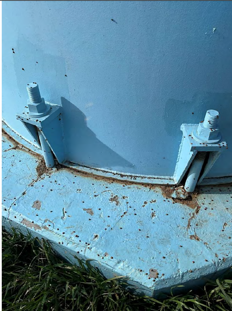
Narka Tower concrete base with minor cracking
