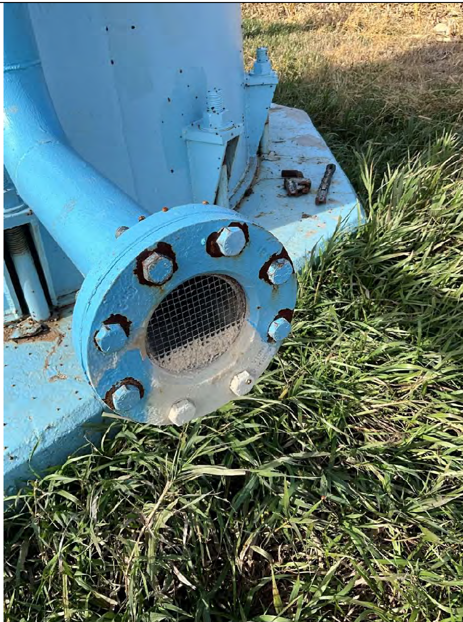
Narka Tower overflow with screen note calcium accumulation on the overflow screen
