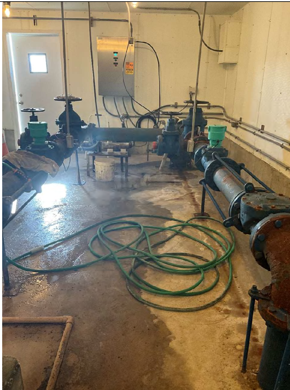
View of South Well piping
