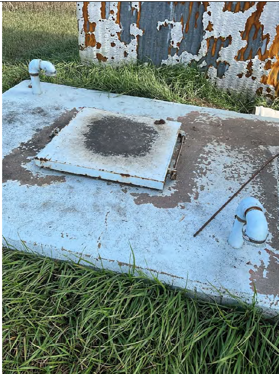
Norway Tower altitude valve pit
