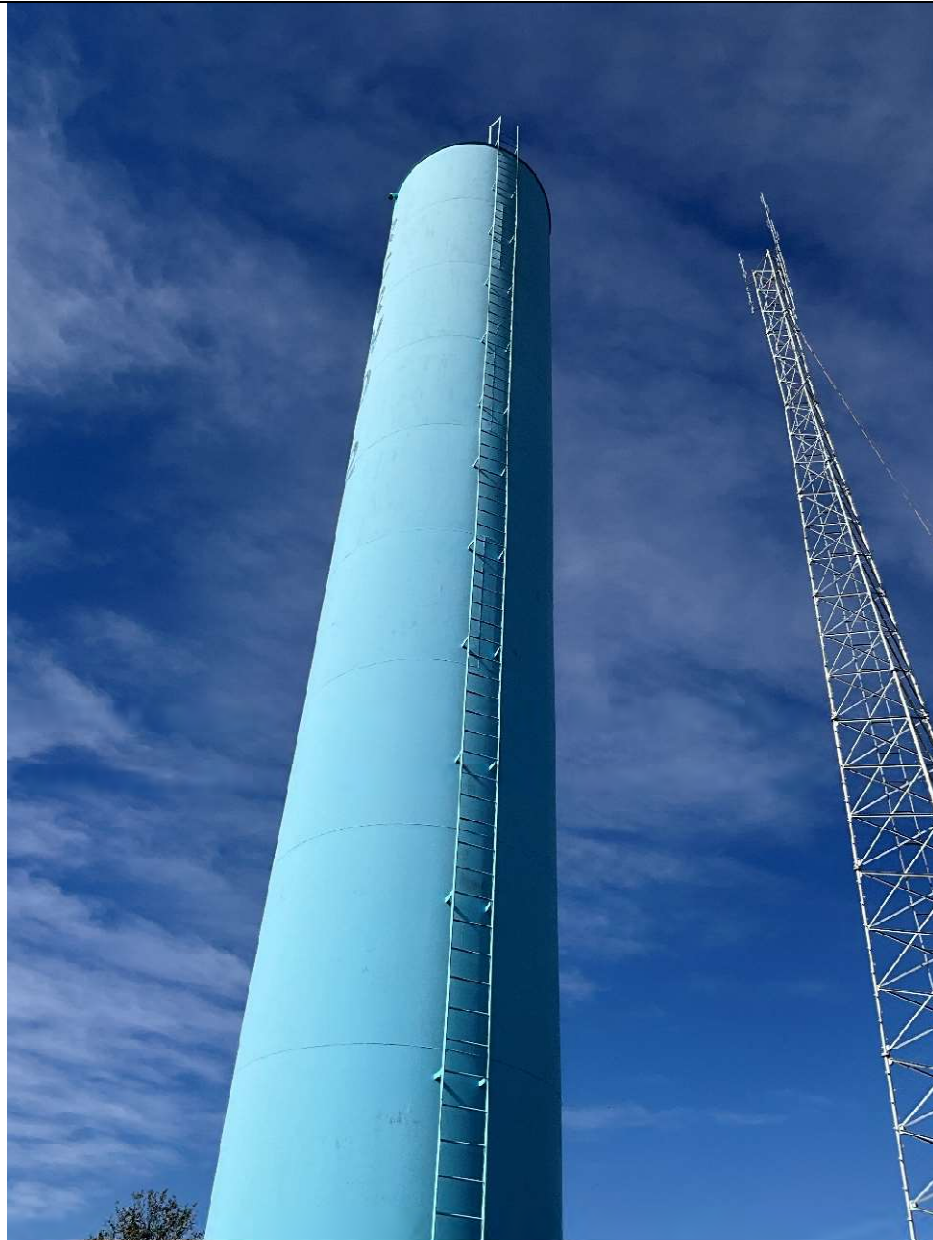
Francis Tower exterior – note the overflow is screeded but not extended to ground level
