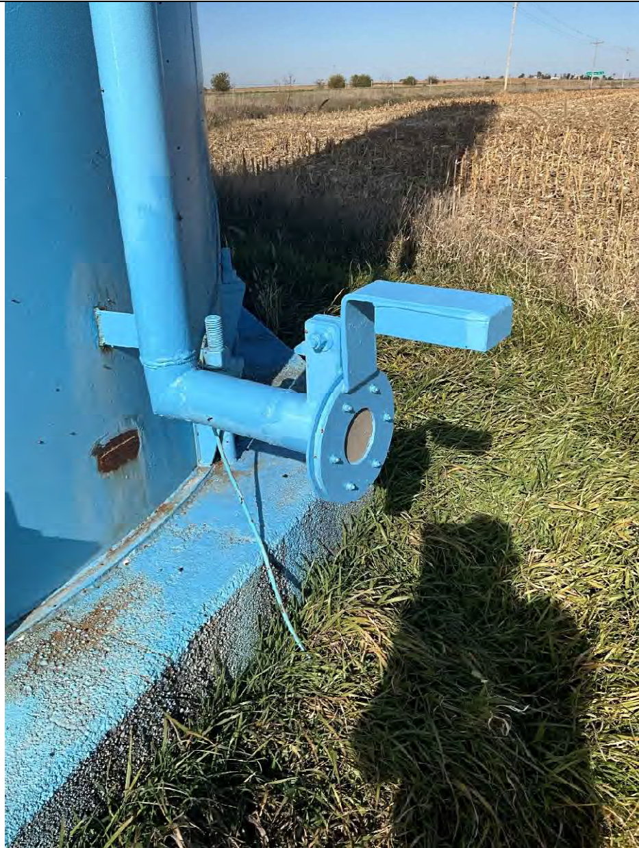
81 Tower -overflow discharge outlet with screen and without splash pad
