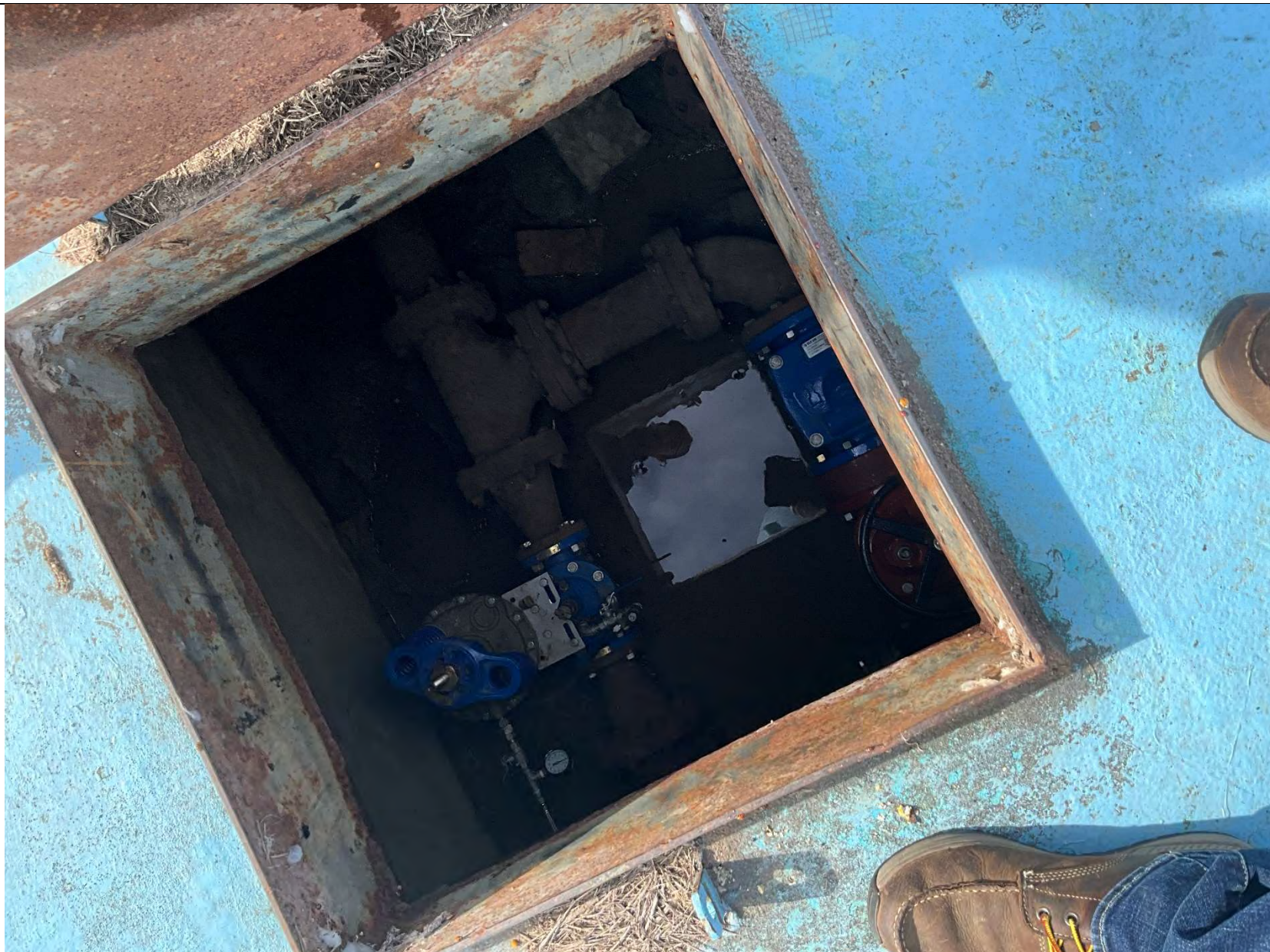
Narka Tower altitude valve vault with leak observed
