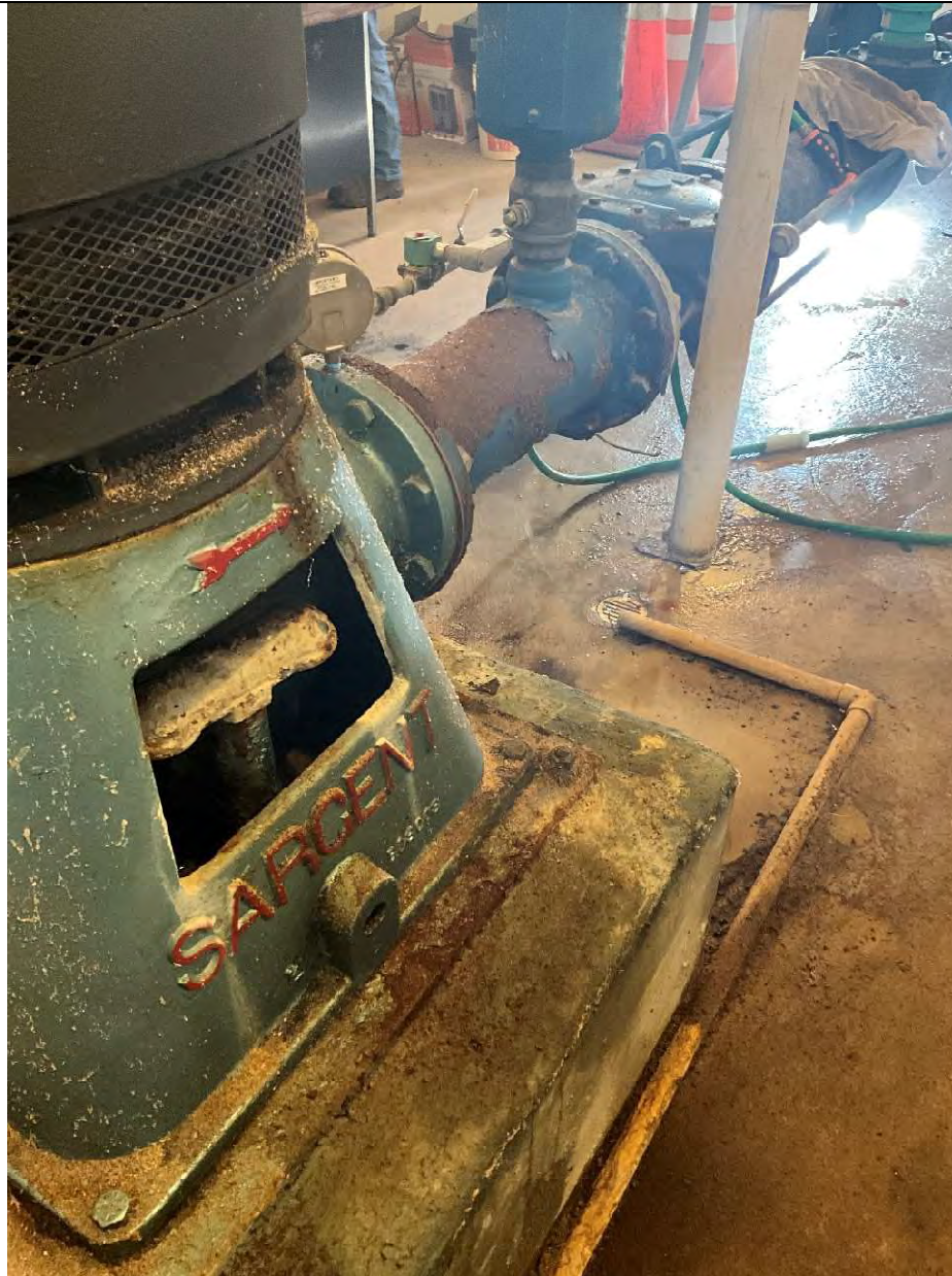
South Well with pump motor, casing vent, concrete well base, and pressure relief valve screened discharge line. Note corrosion on piping
