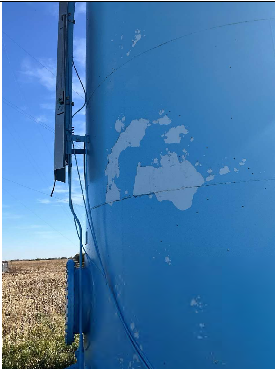
81 Tower exterior paint peeling after being recently painted
