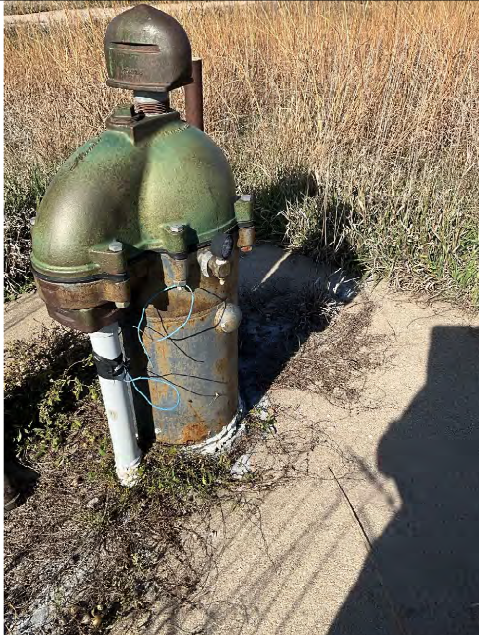
North Well – submersible pump with cracked concrete pad and tall vegetation surrounding
