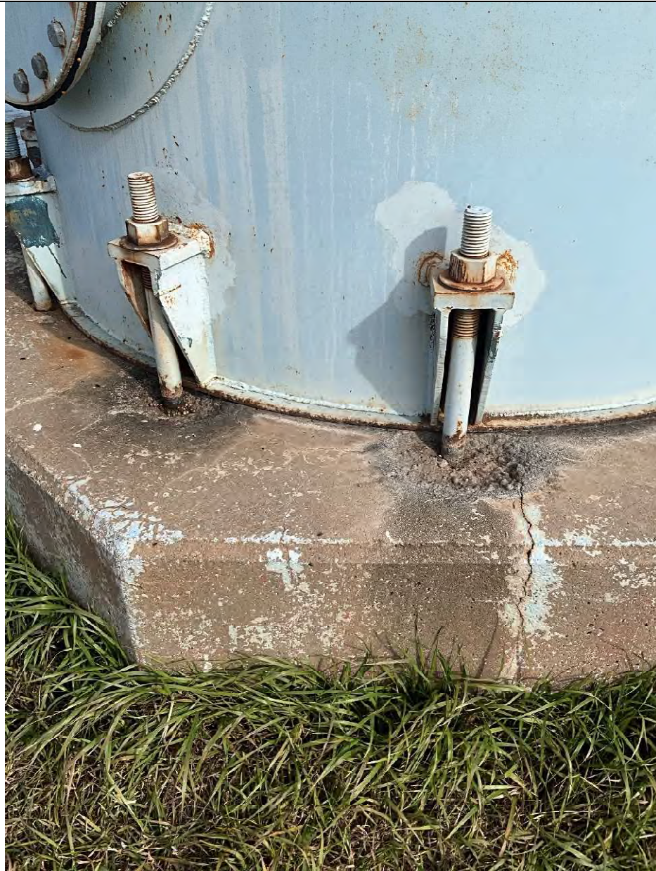
Norway Tower concrete base with cracks and pitting around the foundation bolts
