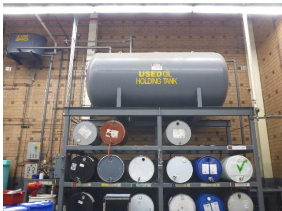
Photo 1: Used oil storage tank stored at the top of a shelving unit holding oil products in the Scrap Room.
