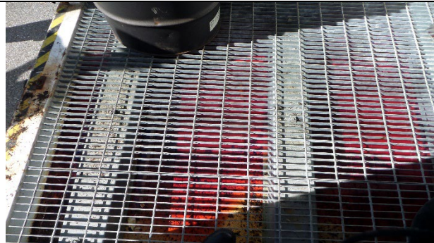
Photo-15 Unknown liquid spill in the secondary containment of Central Accumulation Point Storage Unit
