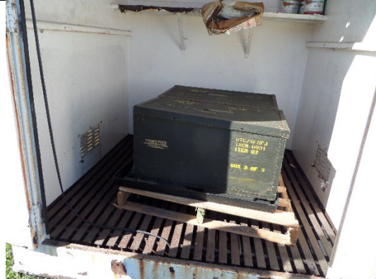
Photo-6 Nonhazardous Spent Batteries Boxes
