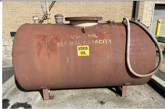
Photo-9 Used Oil Tank with a visible label
