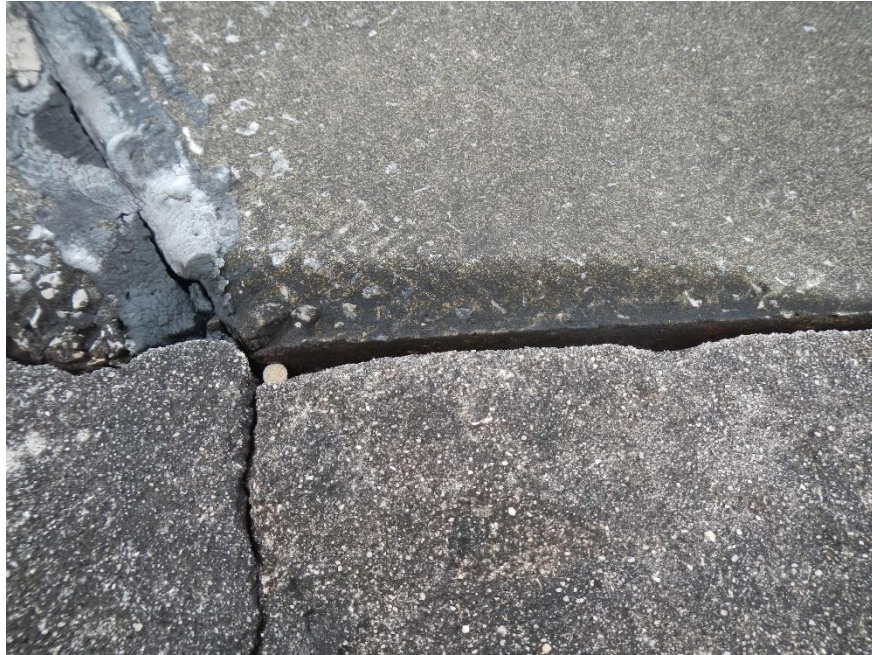
Photograph 13: Close-up image of missing seal around oval ground storage tank.
