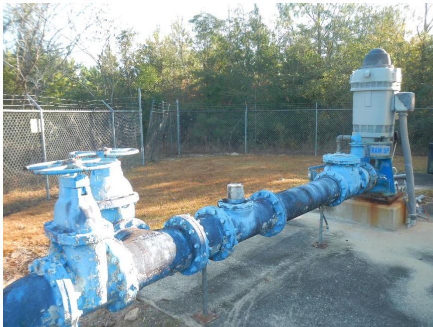
Photograph 2: Well 7 exhibiting biogrowth and corrosion.
