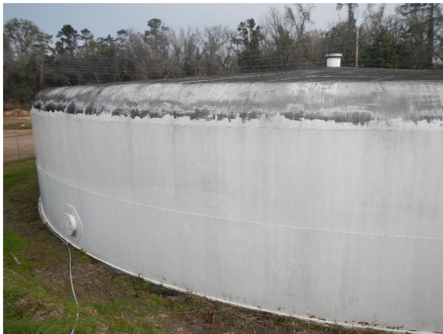
Photograph 16: Deteriorated seal on base of million-gallon ground storage tank.
