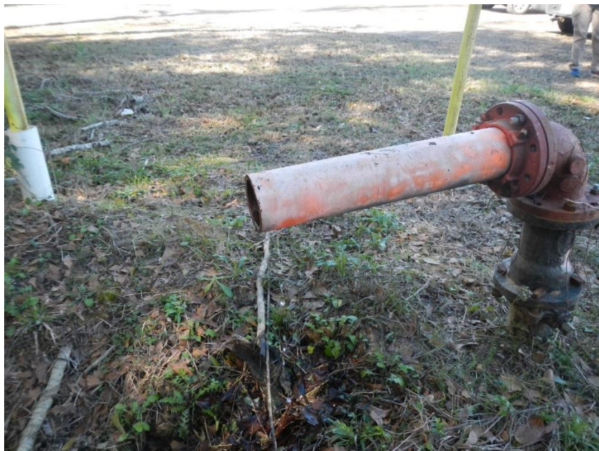
Photograph 6: Missing 24-mesh on discharge pipe at Well 4.
