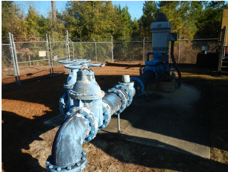
Photograph 1: Well 6 exhibiting biogrowth and corrosion.
