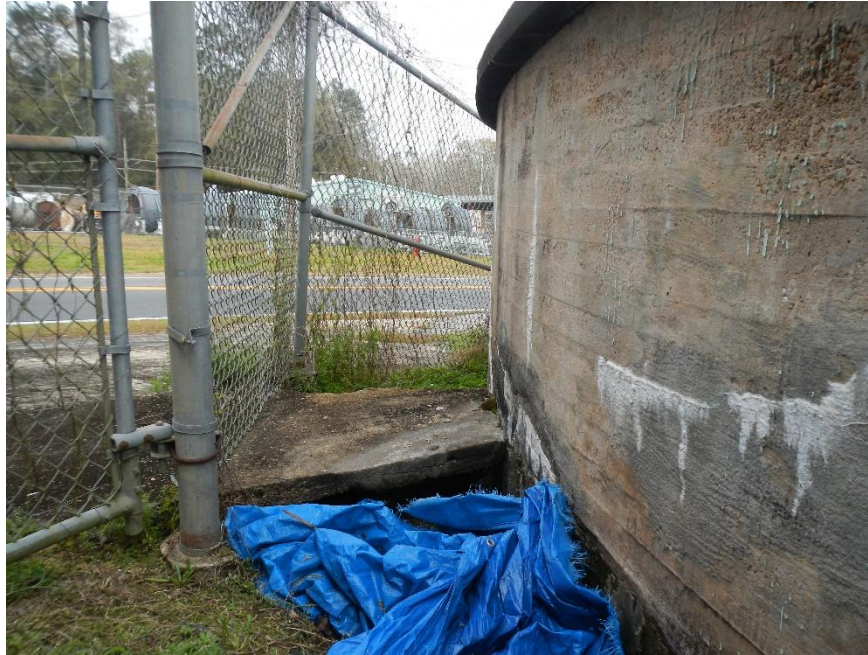
Photograph 15: Leak beneath concrete slab on southwest side of cone ground storage tank.
