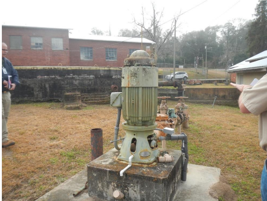
Photograph 5: Well 2 pump head and base exhibiting corrosion.
