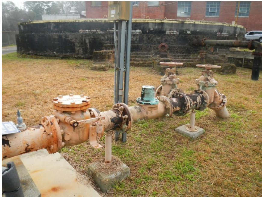
Photograph 4: Well 2 piping exhibiting corrosion.
