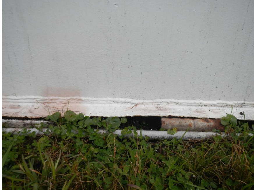
Photograph 17: Close-up of deteriorated seal on base of million-gallon ground storage tank.
