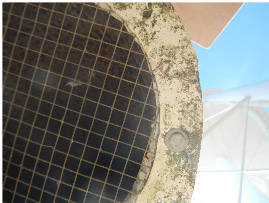
Photograph 9: Incorrectly sized mesh at Virginia elevated storage tank overflow.
