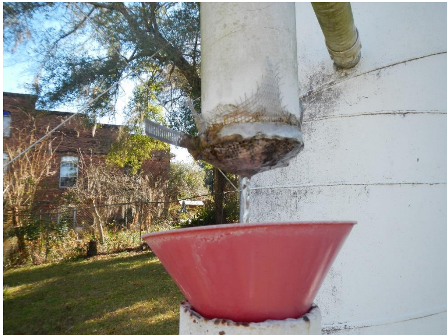
Photograph 18: Leaking overflow at Adams elevated storage tank.
