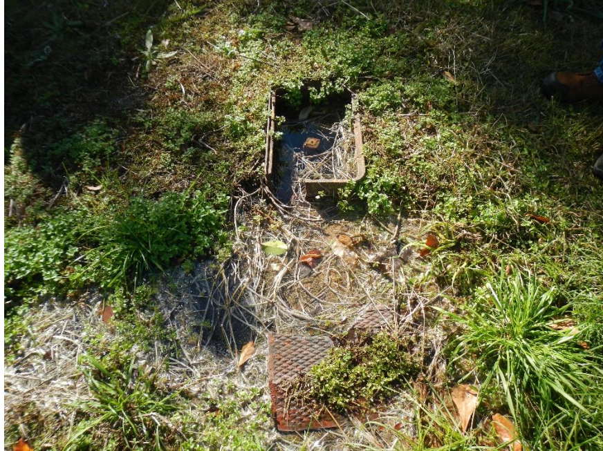
Photograph 19: Accumulation of water at the base of the support structure caused by leaking overflow at Adams elevated storage tank.
