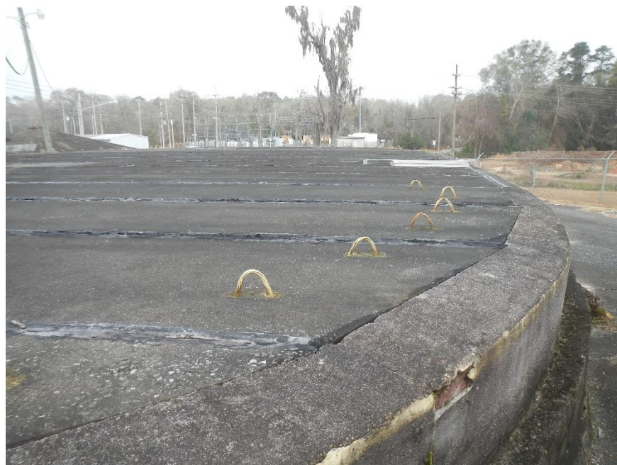
Photograph 12: Covering on oval ground storage tank, which lacks a sanitary seal and has significant cracking.
