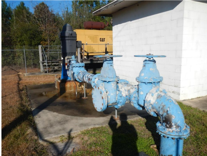
Photograph 3: Well 9 exhibiting biogrowth and corrosion.
