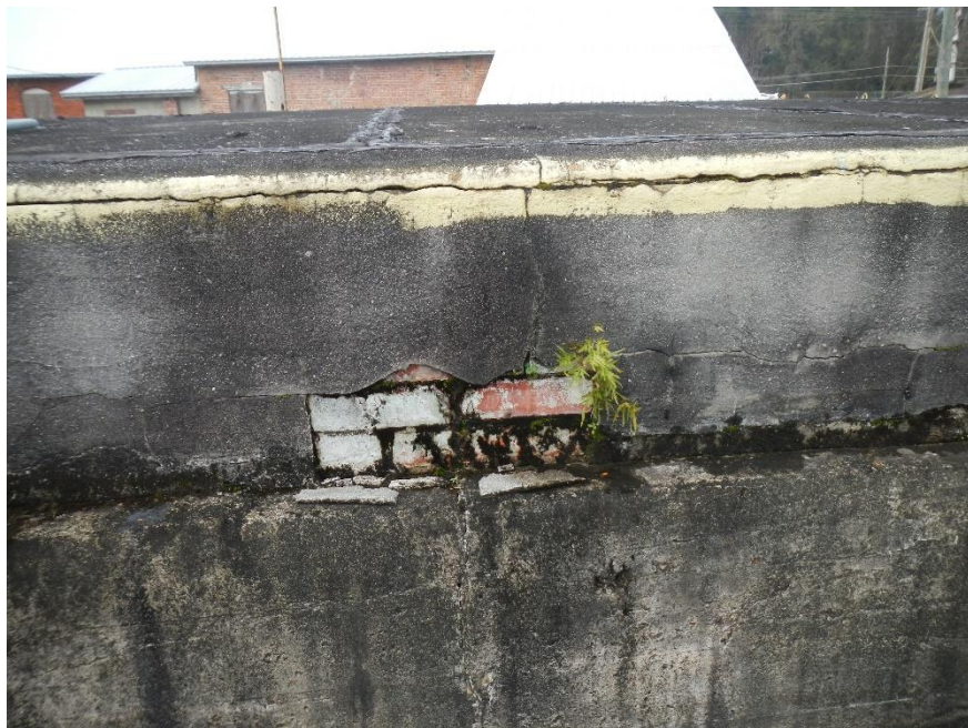
Photograph 14: Exterior deterioration on oval ground storage tank.
