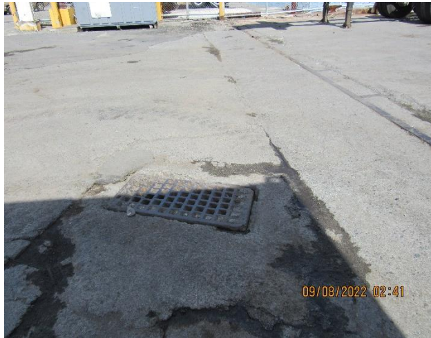
IMG 486 -A storm water catch basin within the fence line. The inlet of the catch basin is not protected.
