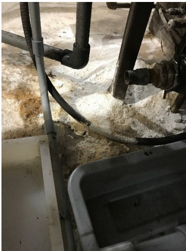
Photo-20 Waste Acid (D002) Spill
