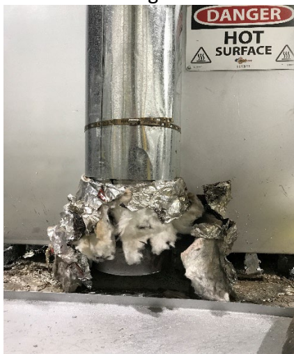
Photo-13 Lead Pot Insulation
