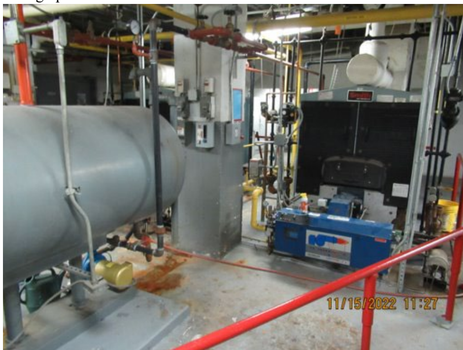
Photograph #8 – Boiler room
