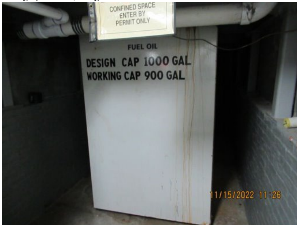
Photograph #9 – 1,000-gallon fuel oil tank located in basement
