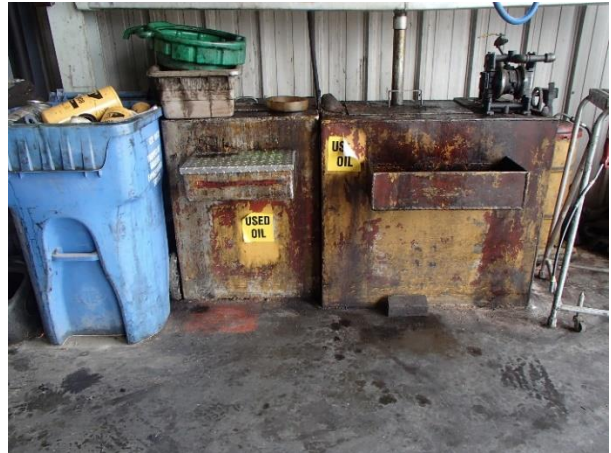
Photo 16: Building 45 used oil tanks.
