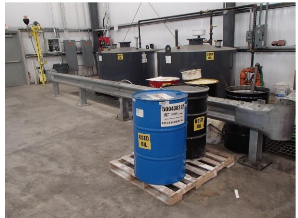
Photo 6: Building 278 Used Oil containers and tanks.
