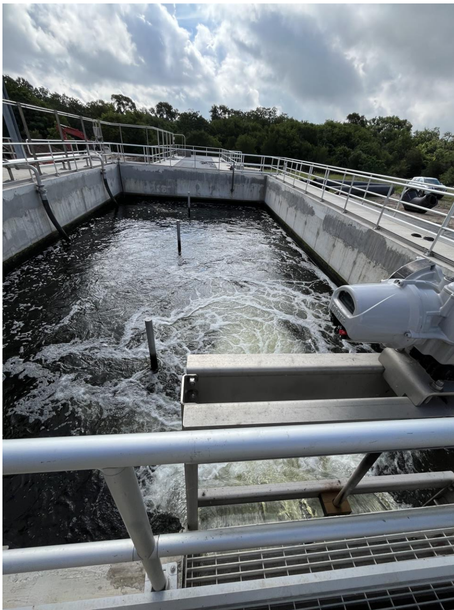
Post Aeration Basin
