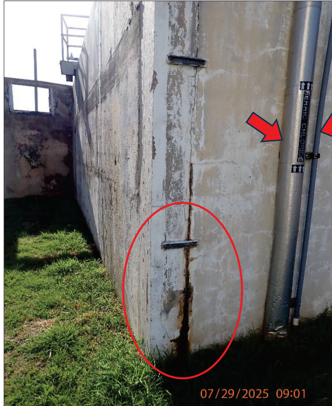
Photograph 5. 7/29/2025 09:01 P7290269.JPG Duncan WTP Flash Mixer
