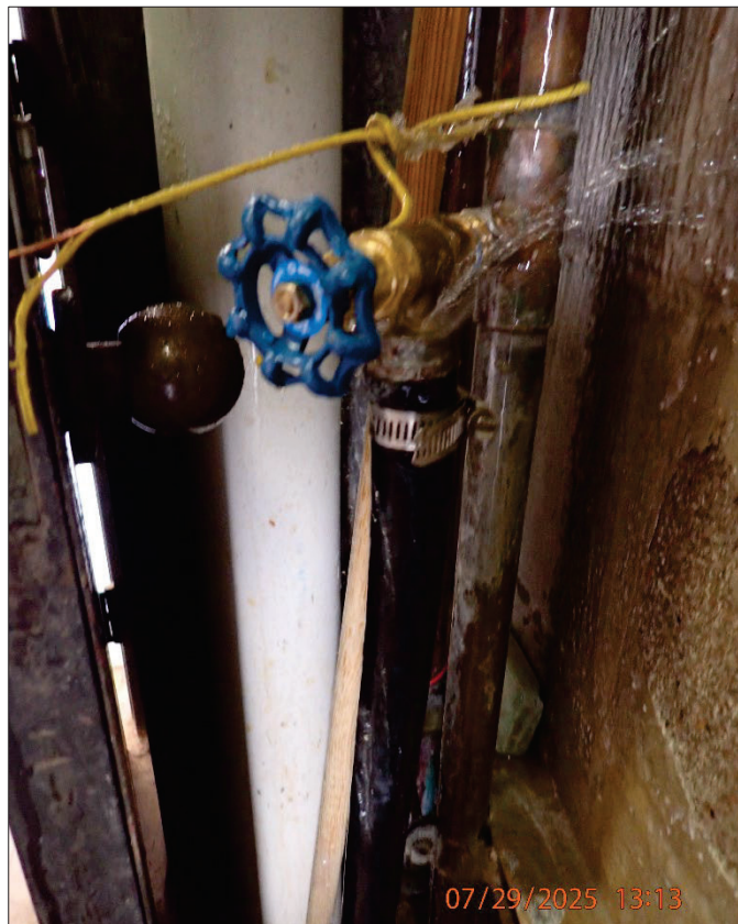
Photograph 46. 7/29/2025 13:13 P7290526.JPG ACH and Caustic Chemical Building
