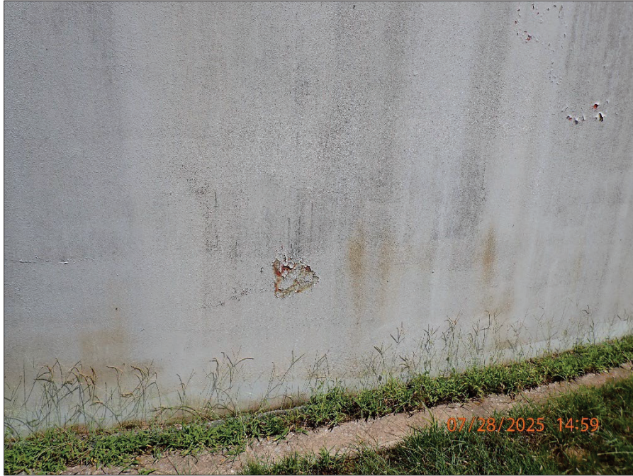
Photograph 71. 7/28/2025 14:59 P7280148.JPG 10th and Elk N.E Tank Description: Peeling surface coating at the 10th and Elk N.E Tank.
