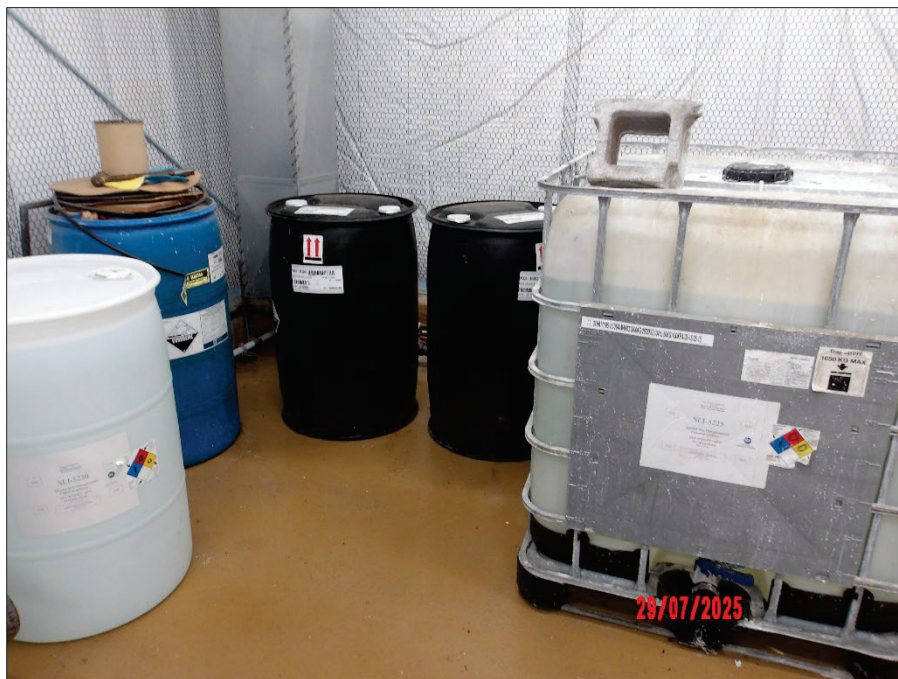
Photograph 40. 7/29/2025 10:27 100_0172.JPG Polyphosphate Storage Room Description: Storage of poly-orthophosphate, 23 percent hydrofluosilicic acid, and 12 percent sodium hypochlorite drums in the Polyphosphate Storage Room.
