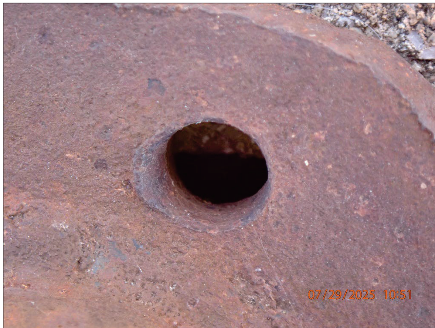
Photograph 36. 7/29/2025 10:51 P7290481.JPG 3.5 MG Clearwell
