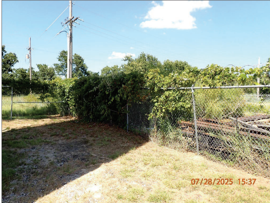
Photograph 73. 7/28/2025 15:37 P7280213.JPG North Industrial Tower #2 (East) Description: Vegetation growth on the security fencing around North Industrial Tower #2 (East).
