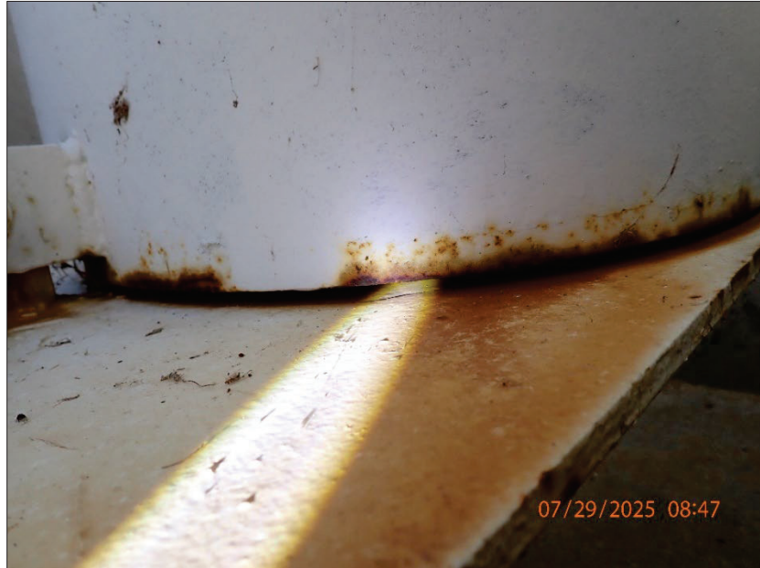
Photograph 1. 7/29/2025 08:47 P7290243.JPG Duncan WTP Backwash Tank Description: Metal flapper on the end of the overflow line on the backwash supply tank that does not create a proper seal.
