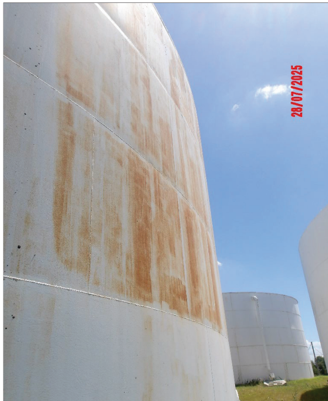
Photograph 70. 7/28/2025 14:04 100_0076.JPG 10th and Elk N.E. Tank Description: Corrosion on the surface coating of the 10th and Elk N.E. Tank
