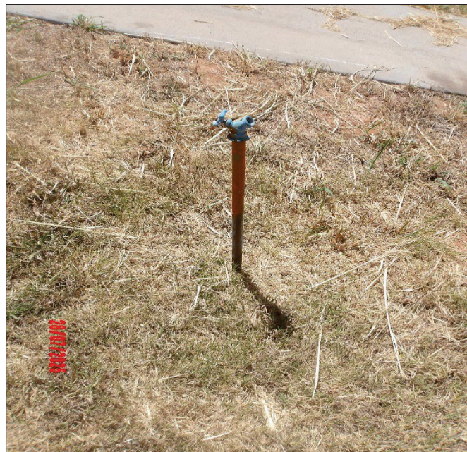
Photograph 76. 7/28/2025 14:53 100_0112.JPG N.W. Sector Tower Description: Threaded hose tap at N.W. Sector Tower is missing a hose bib vacuum breaker device.
