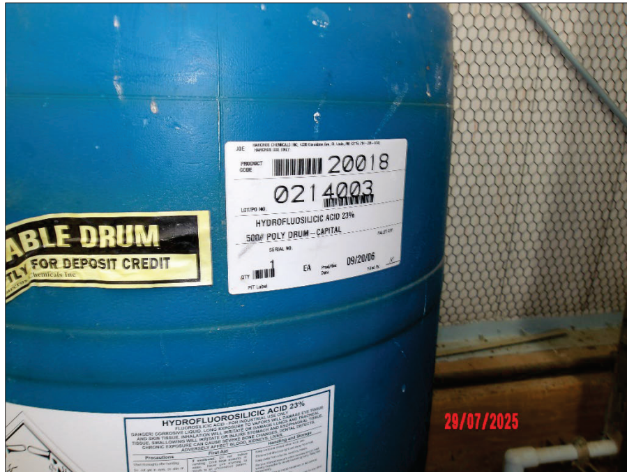
Photograph 41. 7/29/2025 10:27 100_0171.JPG Polyphosphate Storage Room Description: 23 percent hydrofluorosilicic acid drum in the polyphosphate storage room.
