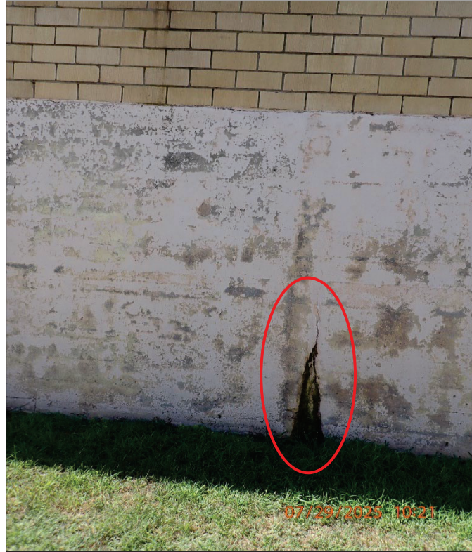
Photograph 17. 7/29/2025 10:21 P7290415.JPG South Plant Filter 6
