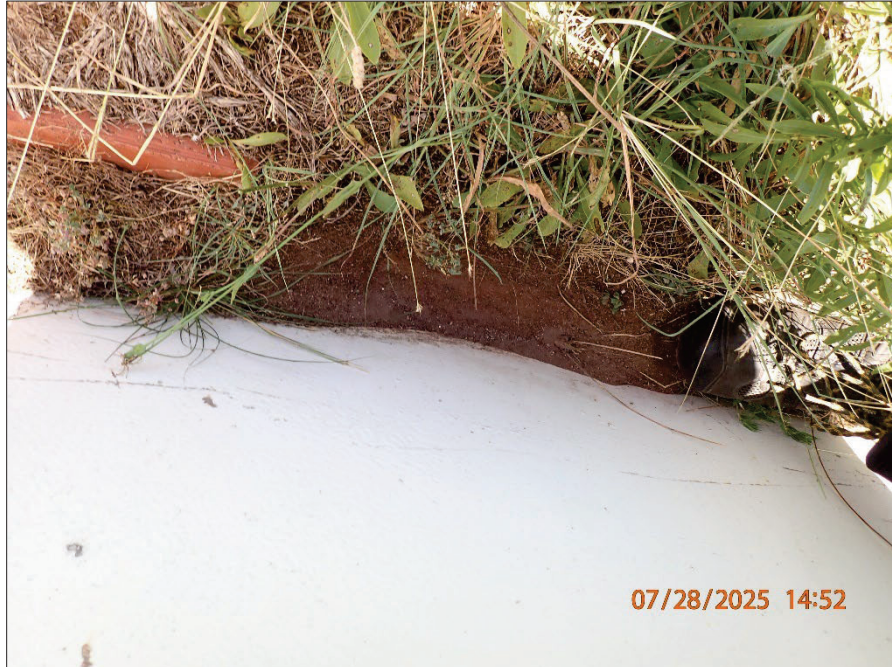
Photograph 63. 7/28/2025 14:52 P7280125.JPG 10 th and Elk N.W Tank Description: Soil build-up at the base of the 10 th and Elk N.W Tank covering the tank ring.
