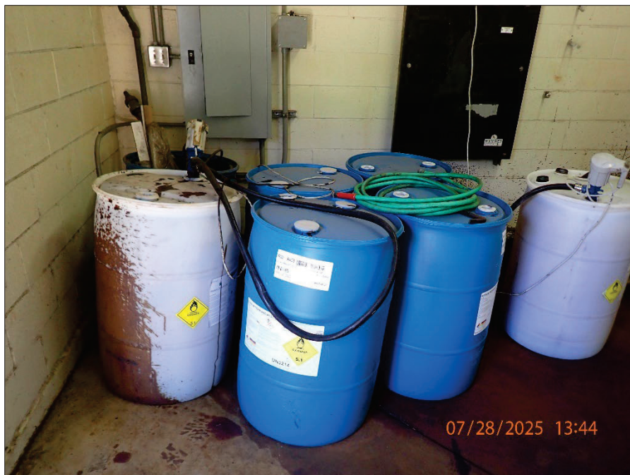
Photograph 52. 7/28/2025 13:44 P7280049.JPG Permanganate Storage and Feed Room Description: Sodium permanganate storage without secondary containment.
