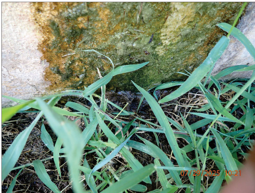
Photograph 18. 7/29/2025 10:21 P7290416.JPG South Plant Filter 6
