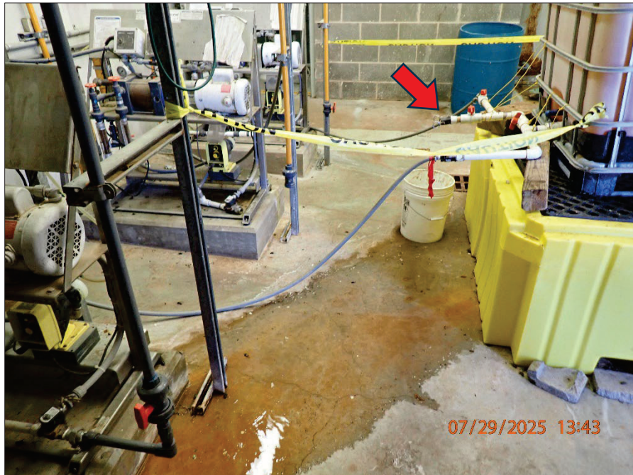
Photograph 49. 7/29/2025 13:43 P7290595.JPG Polymer Feed and Storage Room Description: Spill containment does not extend below the IBC tote pipe connections. Note that the liquid on the floor is ground water and not polymer.
