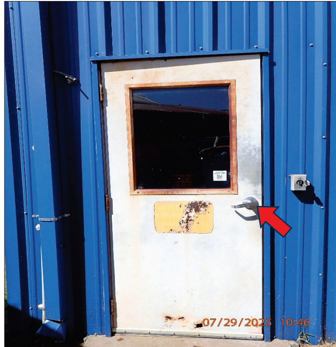
Photograph 31. 7/29/2025 10:46 P7290471.JPG Ammonia Storage Room
