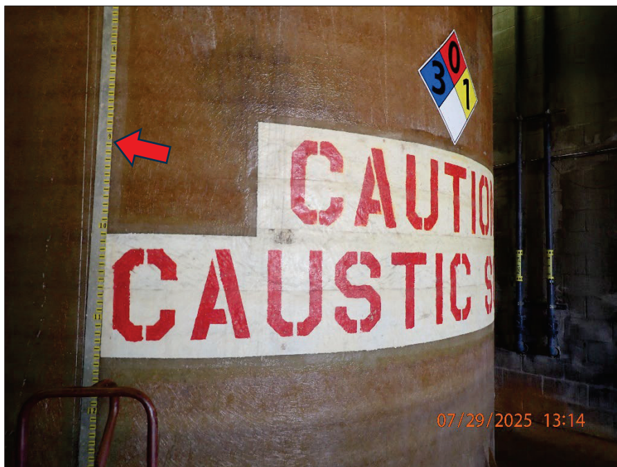
Photograph 44. 7/29/2025 13:14 P7290533.JPG ACH and Caustic Chemical Building Description: Caustic soda and ACH bulk storage tanks with tap measure on the side of the 8,000 gallon fiberglass storage tanks.
