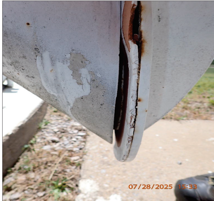
Photograph 75. 7/28/2025 15:33 P7280202.JPG North Industrial Tower #2 (East) Description: Metal flapper on the end of the overflow line on the Industrial #2 Tower that does not create a proper seal.
