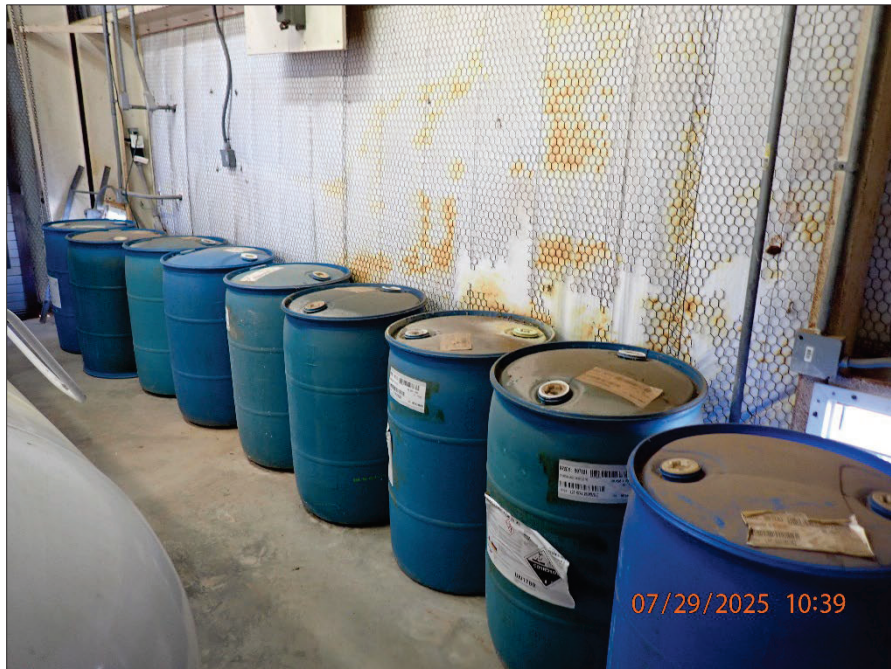
Photograph 22. 7/29/2025 10:39 P7290449.JPG Ammonia Storage Room Description: Hydrochloric acid drums located in the anhydrous ammonia storage room without secondary containment at the Water Treatment Facility.
