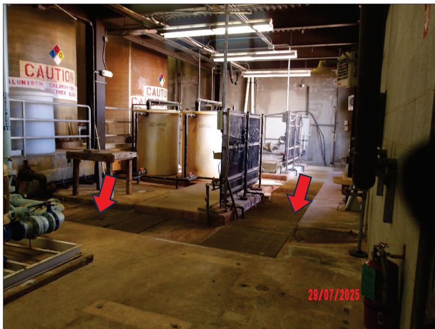
Photograph 43. 7/29/2025 10:32 100_0182.JPG ACH and Caustic Chemical Building Description:. Caustic soda and ACH bulk storage tanks and day tanks with a shared drainage system for accidental spills.
