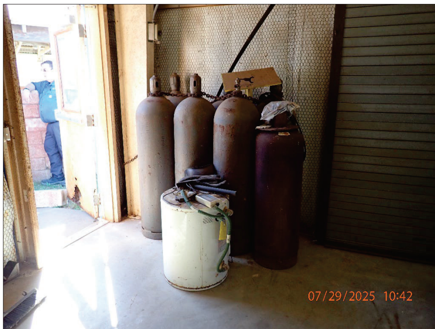
Photograph 26. 7/29/2025 10:42 P7290461.JPG Ammonia Storage Room
