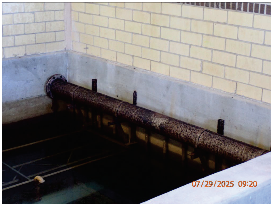
Photograph 8. 7/29/2025 09:20 P7290302.JPG South Plant Filter 5
