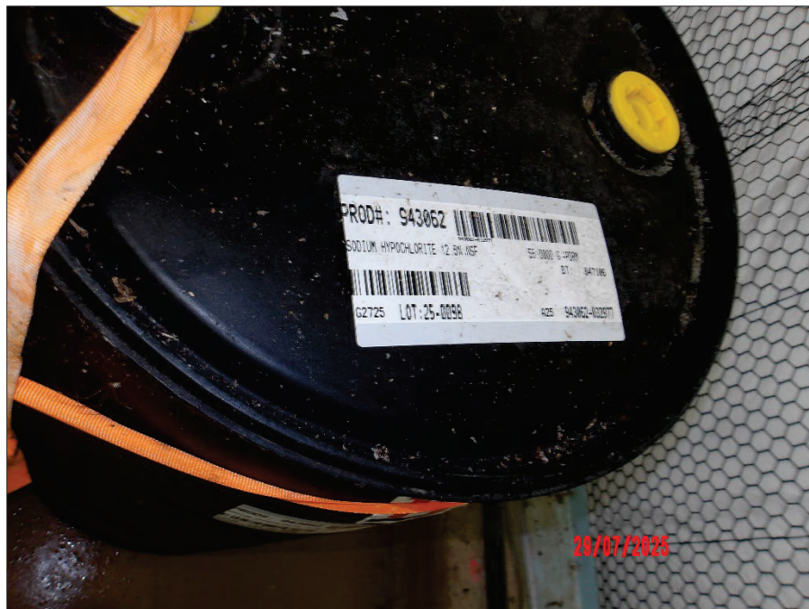
Photograph 42. 7/29/2025 10:23 100_0166.JPG Polyphosphate Storage Room Description: Drums of sodium hypochlorite stored in the Polyphosphate Storage Room.
