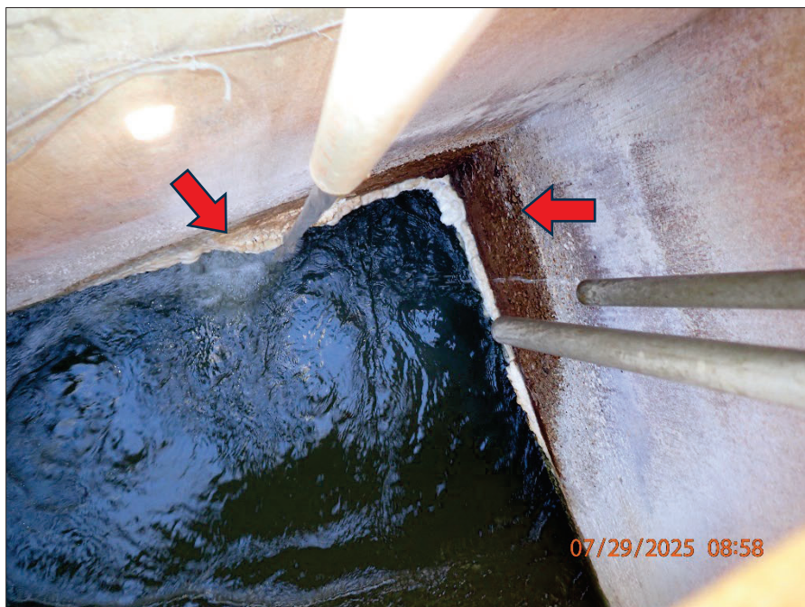
Photograph 4. 7/29/2025 08:58 P7290263.JPG Duncan WTP Flash Mixer Description: ACH and Polymer injection points into the flash mixer. Note the proximity to the concrete wall, chemical buildup on the wall, and erosion of the concrete.
