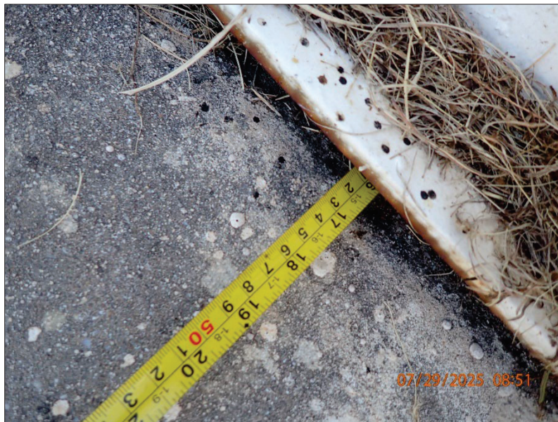
Photograph 2. 7/29/2025 08:51 P7290252.JPG Duncan WTP Backwash Supply Tank Description: Gap between the base of the WTP backwash supply tank and the concrete tank pad.
