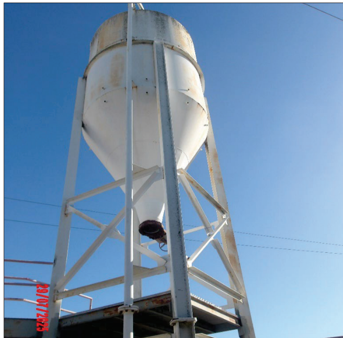
Photograph 6. 7/29/2025 08:04 100_0008.JPG Duncan WTP PAC Tank
