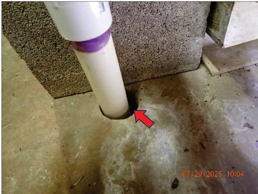
Photograph 16. 7/29/2025 10:04 P7290380.JPG South Plant Filter Gallery Description: Unsealed opening on roof of 0.5 MG clearwell, around sample pump access piping.
