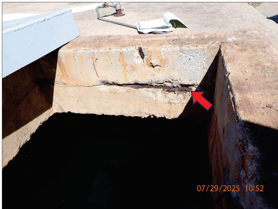
Photograph 34. 7/29/2025 10:52 P7290488.JPG 3.5 MG Clearwell Description: Cracked concrete and exposed rebar around the 3.5 MG Clearwell access hatch.
