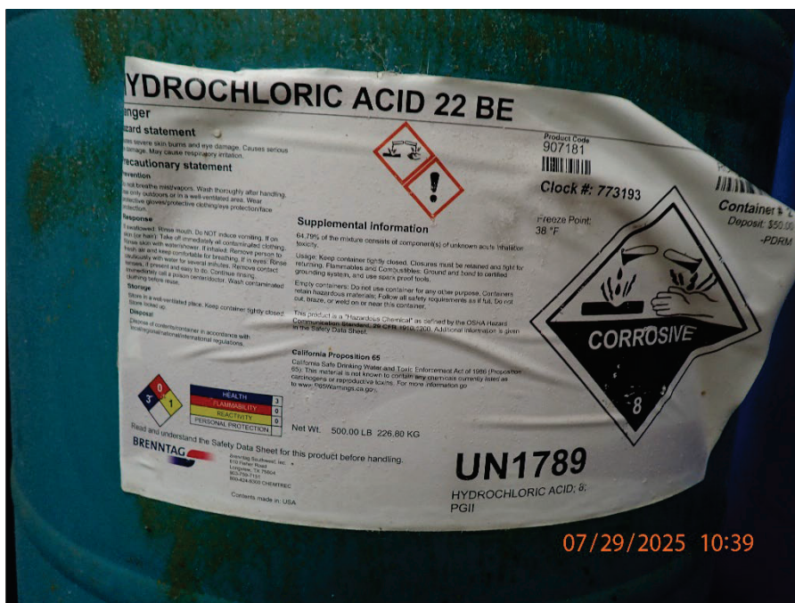
Photograph 24. 7/29/2025 10:39 P7290446.JPG Ammonia Storage Room Description: Hydrochloric acid drum label at the Water Treatment Facility.
