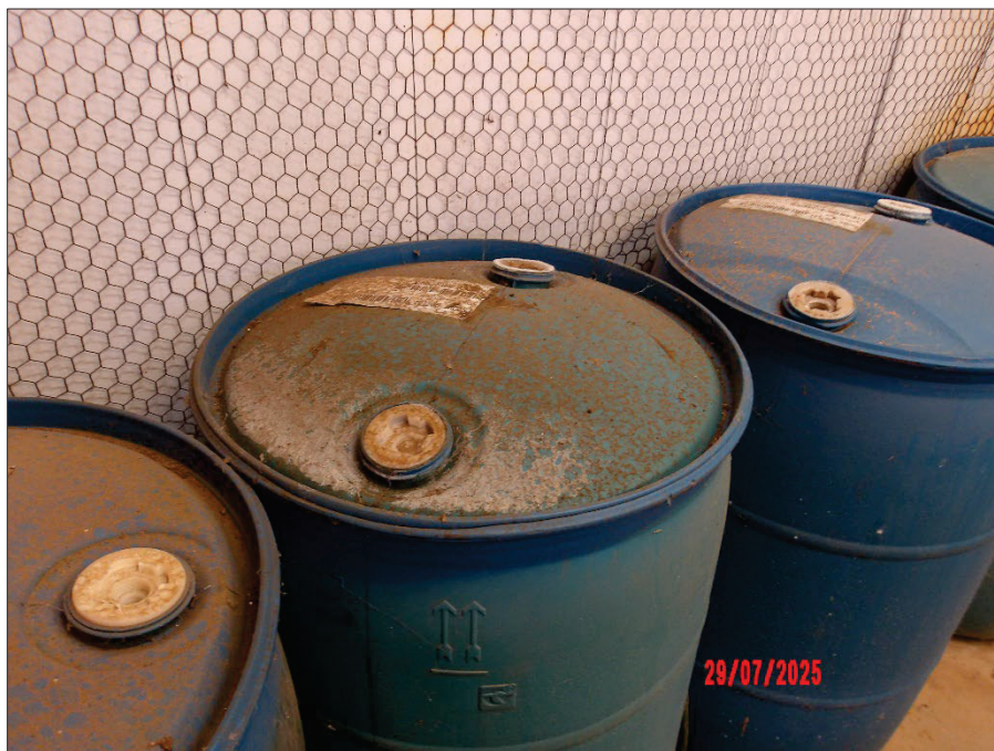
Photograph 23. 7/29/2025 09:40 100_0101.JPG Ammonia Storage Room Description: Hydrochloric acid drums located in the anhydrous ammonia storage room at the Water Treatment Facility, without secondary containment, that are bulging due to increased pressure.
