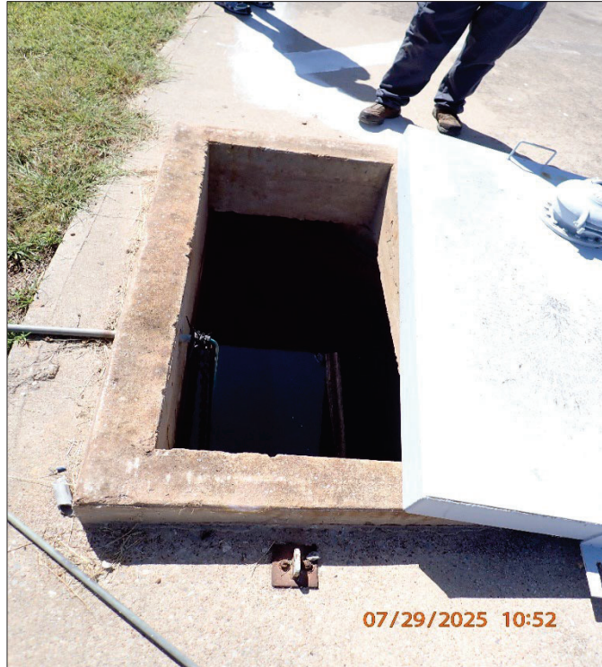
Photograph 33. 7/29/2025 10:52 P7290485.JPG 3.5 MG Clearwell Description: Access hatch to the 3.5 MG clearwell without a gasket seal.
