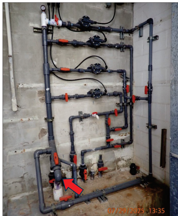
Photograph 48. 7/29/2025 13:35 P7290572.JPG WTP Chlorinator Room
