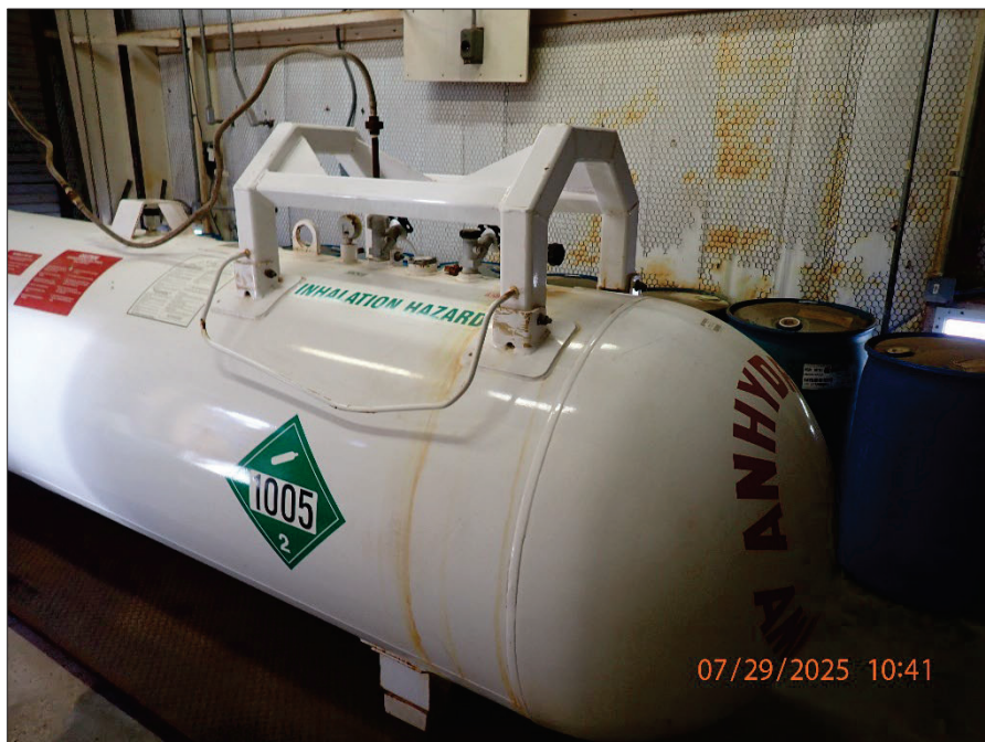
Photograph 27. 7/29/2025 10:41 P7290458.JPG Ammonia Storage Room Description: Hydrochloric acid and phosphate stored in the same room as anhydrous ammonia.
