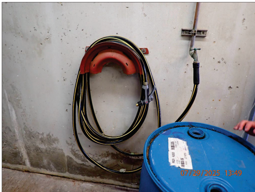
Photograph 50. 7/29/2025 13:49 P7290608.JPG Polymer Feed and Storage Room Description: Garden hose connected to hose bib without vacuum breaker at the polymer storage and feed room.
