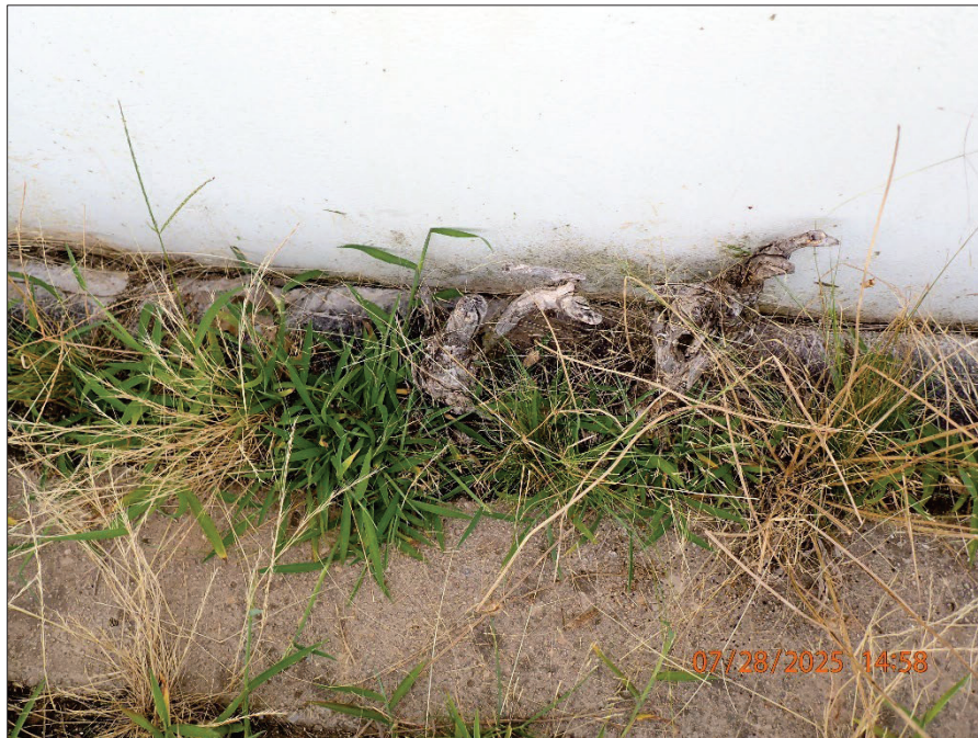
Photograph 64. 7/28/2025 14:58 P7280145.JPG 10 th and Elk N.W Tank Description: Vegetation and roots growing around the foundation of the 10 th and Elk N.W Tank.
