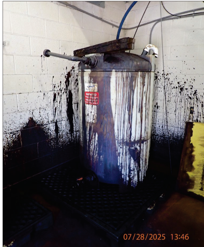
Photograph 53. 7/28/2025 13:46 P7280052.JPG Permanganate Storage and Feed Room Description: Spilled sodium permanganate around the sodium permanganate day tank.
