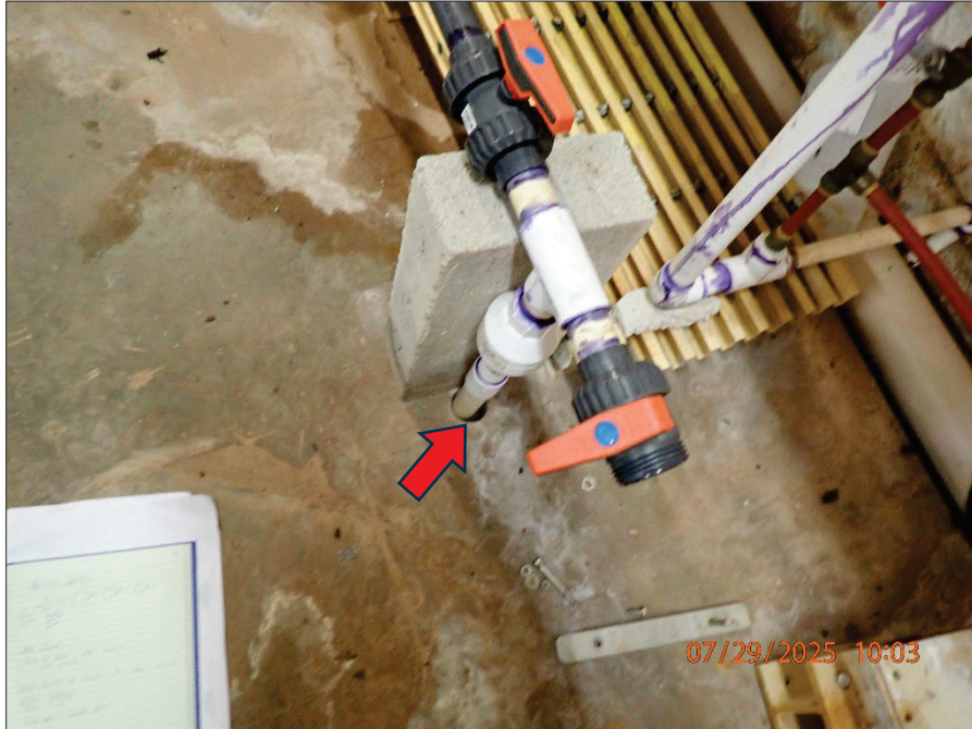
Photograph 15. 7/29/2025 10:03 P7290379.JPG South Plant Filter Gallery Description: Unsealed opening on roof of 0.5 MG clearwell, around sample pump access piping.
