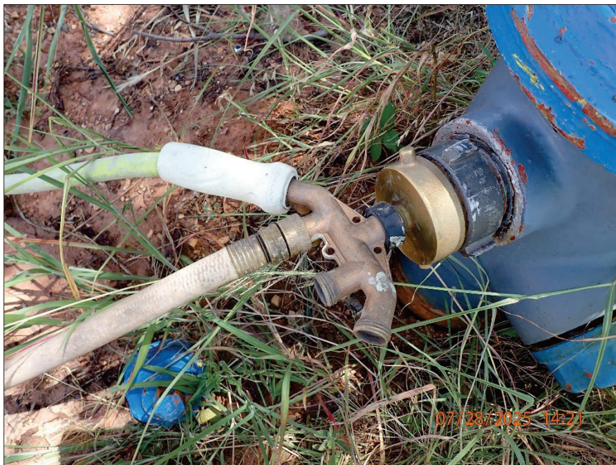
Photograph 54. 7/28/2025 14:21 P7280077.JPG El Rancho Tower Description: Hydrant tap used by the El Rancho Tower construction company without a backflow prevention device.
