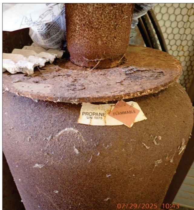
Photograph 28. 7/29/2025 10:43 P7290465.JPG Ammonia Storage Room Description: A single propane tank located in the anhydrous ammonia storage room at the Water Treatment Facility.
