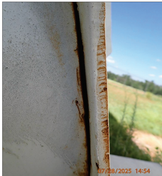
Photograph 66. 7/28/2025 14:54 P7280135.JPG 10 th and Elk N.W Tank
