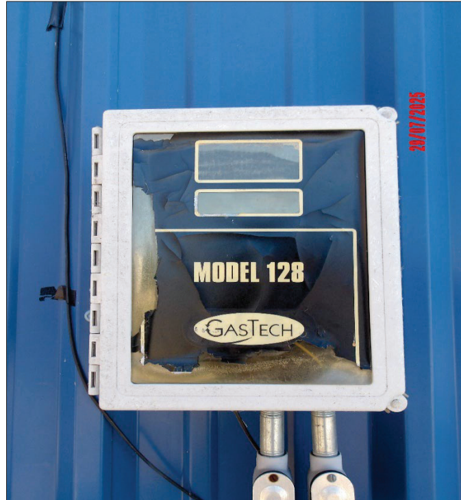
Photograph 21. 7/29/2025 09:34 100_0094.JPG Ammonia Feed Room Description: Disarmed ammonia gas detection alarm at the ammonia feed room.
