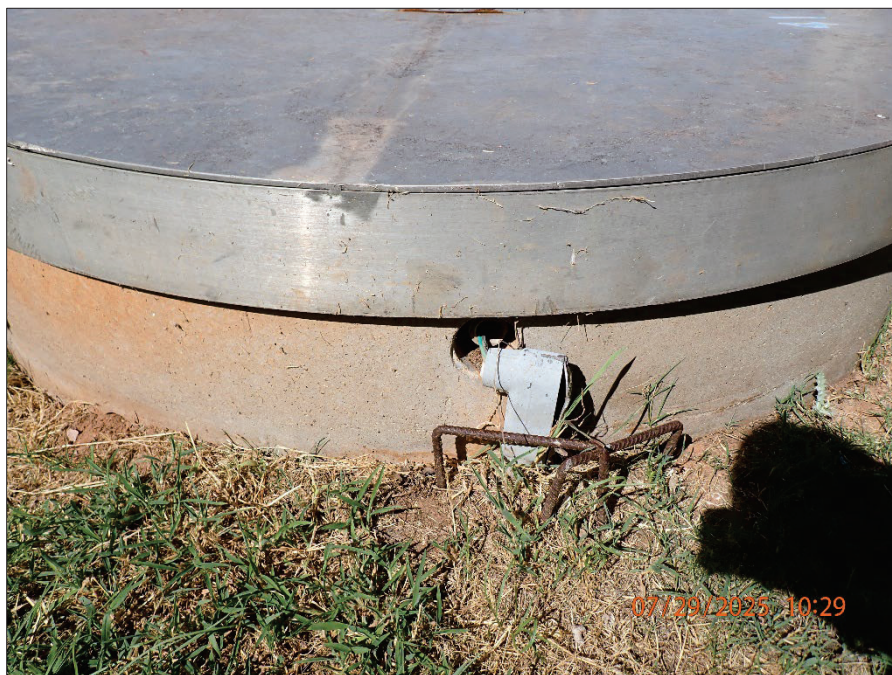
Photograph 20. 7/29/2025 10:29 P7290419.JPG Caustic Feed Pit Description: Caustic feed pit hatch with a broken conduit on the side that allows a direct opening into the pit.
