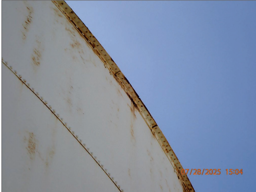
Photograph 69. 7/28/2025 15:04 P7280170.JPG 10 th and Elk South Tank Description: Corrosion on the roof of the 10th and Elk South Tank.
