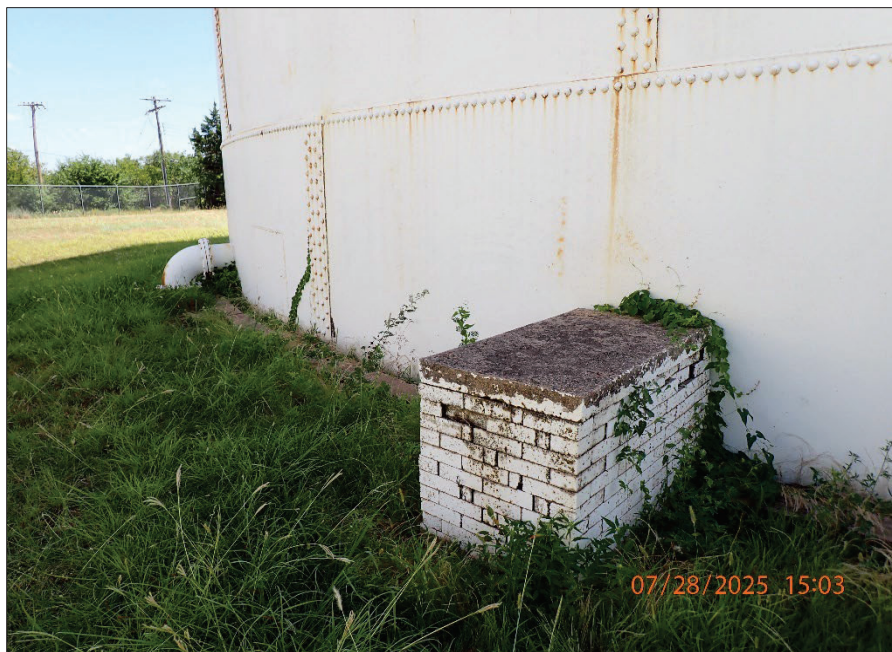
Photograph 62. 7/28/2025 15:03 P7280162.JPG 10 th and Elk South Tank Description: Vegetation growth around the base and climbing up the 10 th and Elk South Tank.
