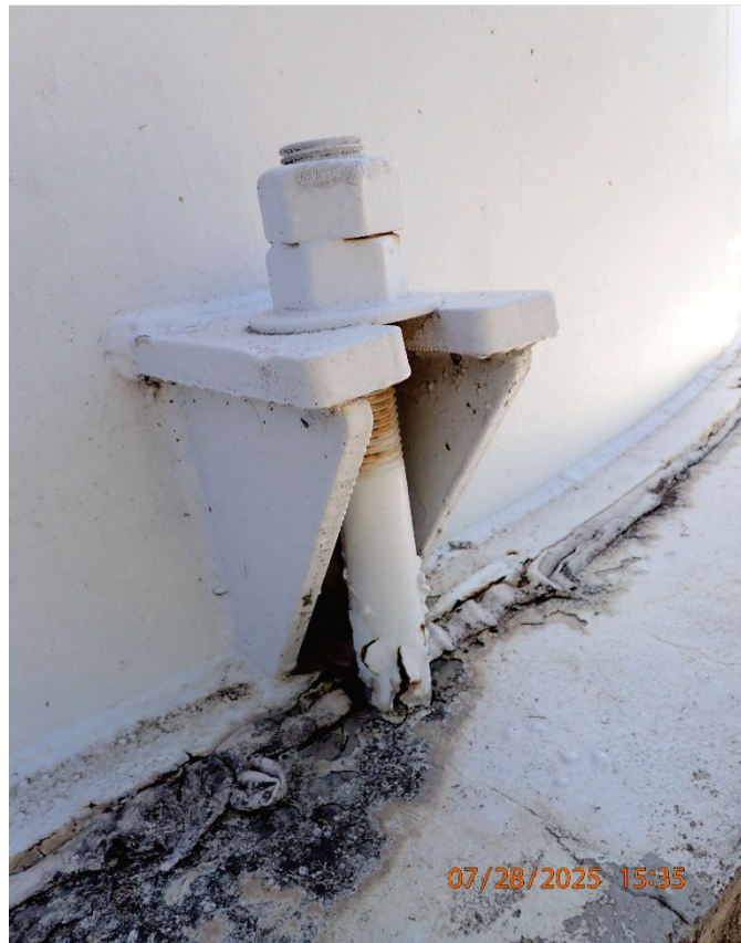
Photograph 74. 7/28/2025 15:35 P7280206.JPG Industrial Tower #2 (East) Description: Corrosion with metal loss on the anchor bolts at Industrial Tower #2.
