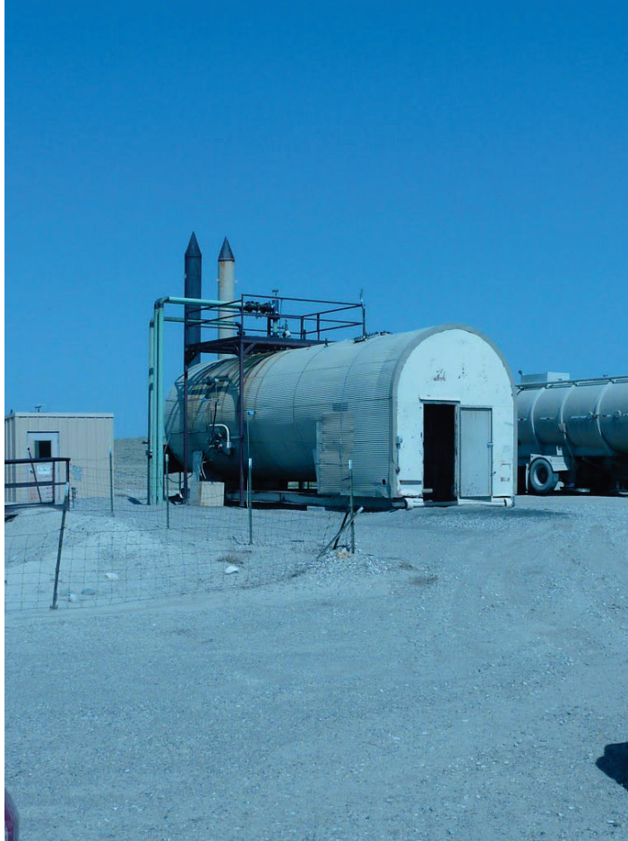
Photo of Current Heater Treater
