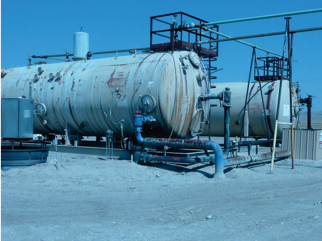
Photo of Water Knockouts
