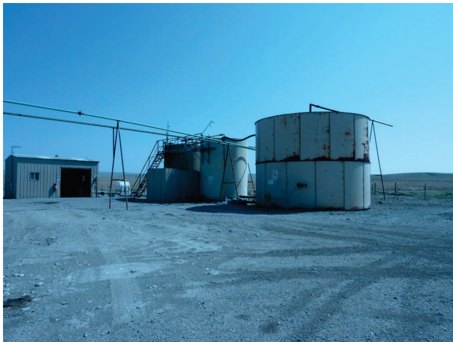
Photo of 2 Produced Water Tanks (each 300 barrels) at the C3 Battery
