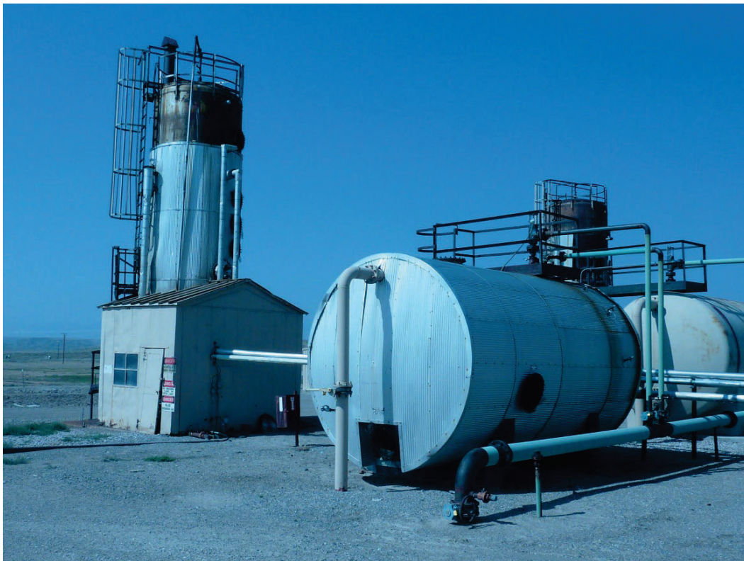
Photo of Two Abandoned Heater Treaters
