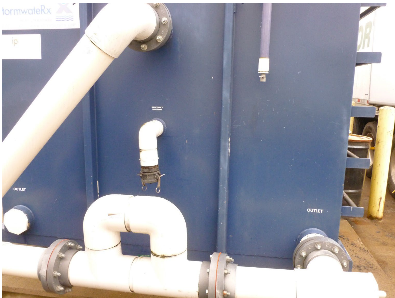
Photo 6 / P1010179 – Filtration System, north end, effluent
