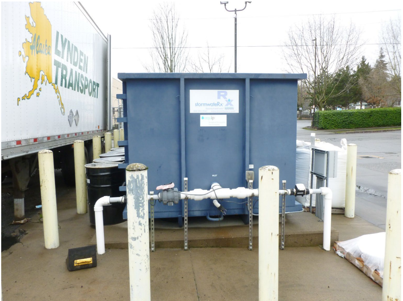
Photo 5 / P1010182 – Filtration System, south end, influent
