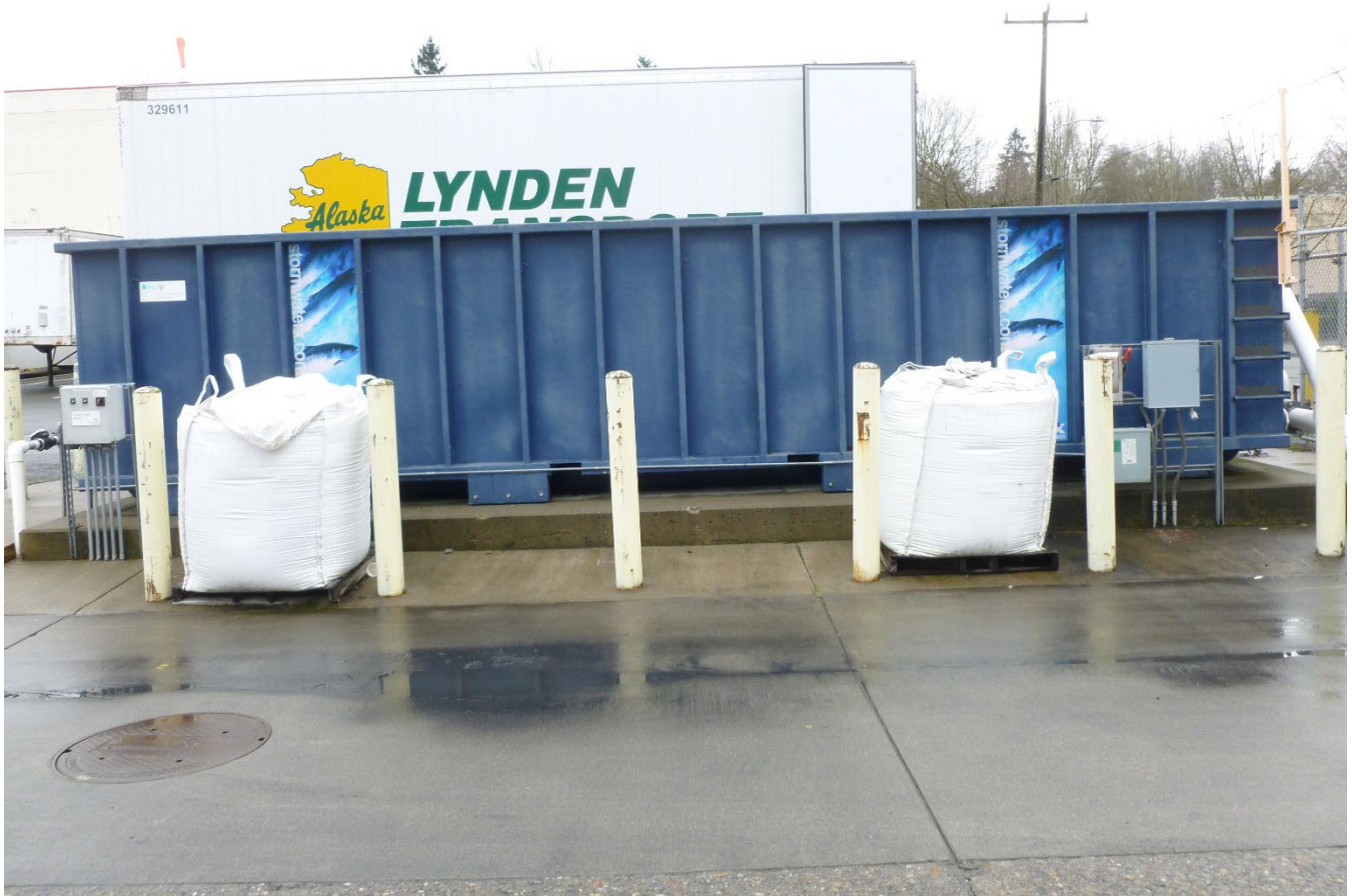
Photo 4 / P1010181 – Filtration System with totes of clean filtration media
