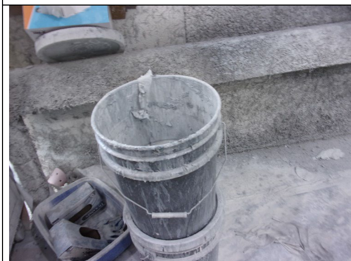
Figure 27: 1:03 PM Commodore Building Lamination One 5-gallon container from spray booth observed.
