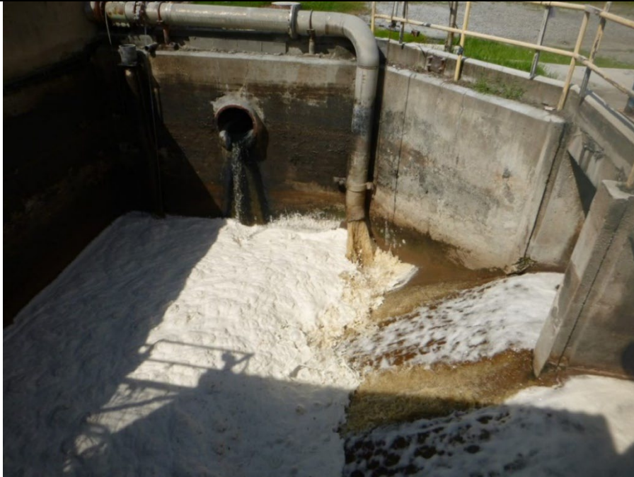
Photograph 6. Sampling point H-2a; the wet well which receives wastewater from H-2, H-2a, and the ash pond, prior to discharge to the POTW.
