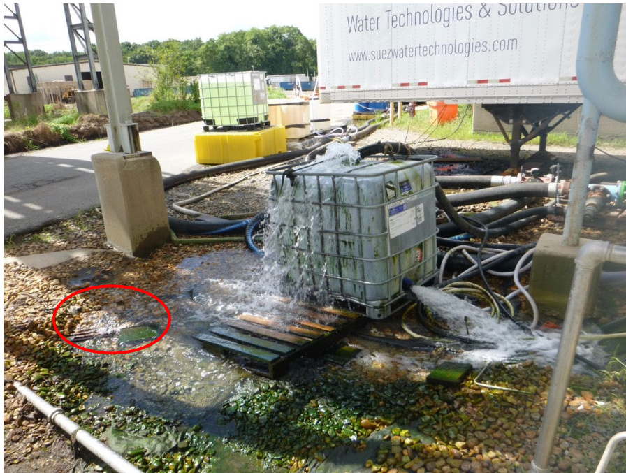
Photograph 8. View of the RO reject water which was overflowing from the tote into a storm drain (circled).
