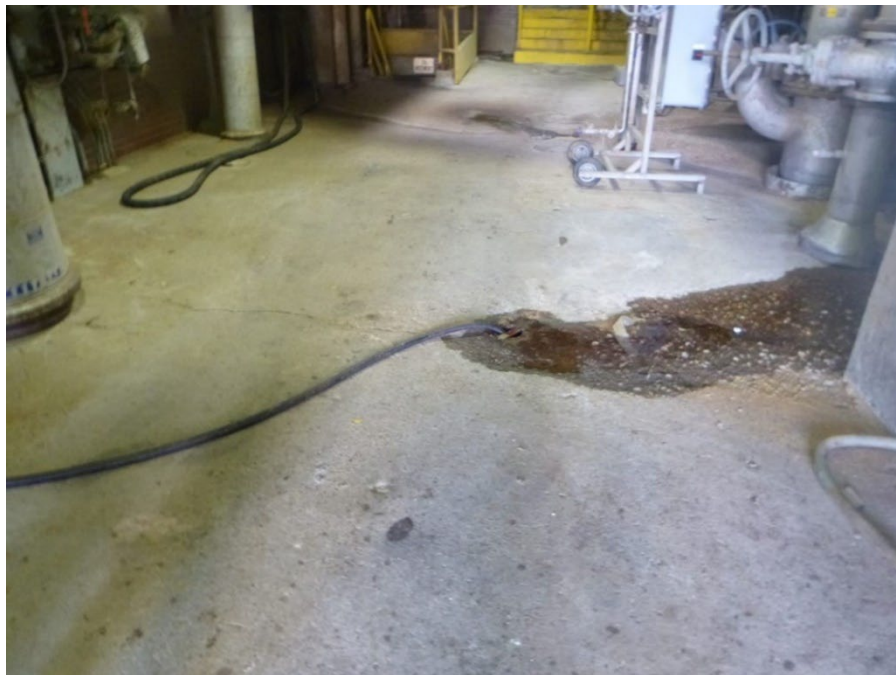
Photograph 9. View of a hose from unknown source located in the paper mill in a room adjacent to the press room.
