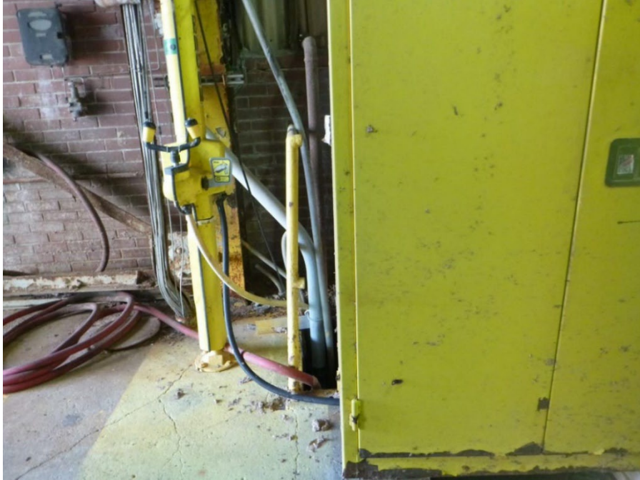
Photograph 10. View of the same hose shown in Photograph 8 from unknown source which is connect to the pipe where the eyewash station is located.
