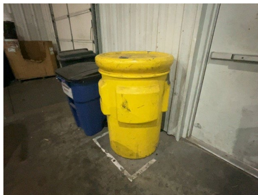
Photo 10: Spill control equipment located in CAA.
