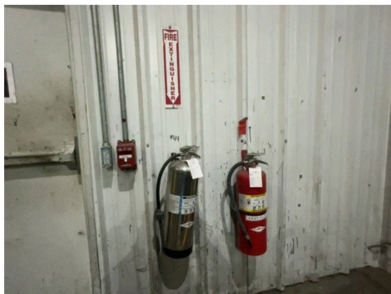
Photo 9: Fire alarms and extinguishers located in CAA and throughout facility.
