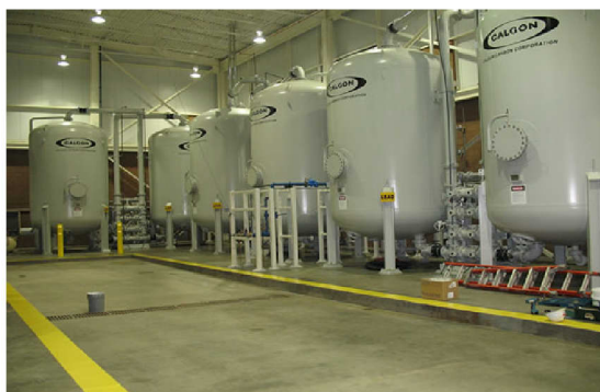
Image: City of Oakdale water treatment plant
